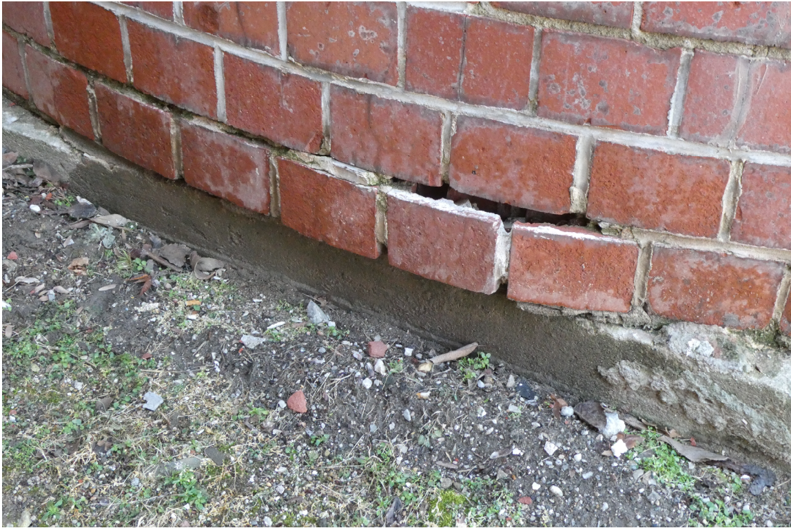
Photo 7 Spalling extends to the base of the stack.
