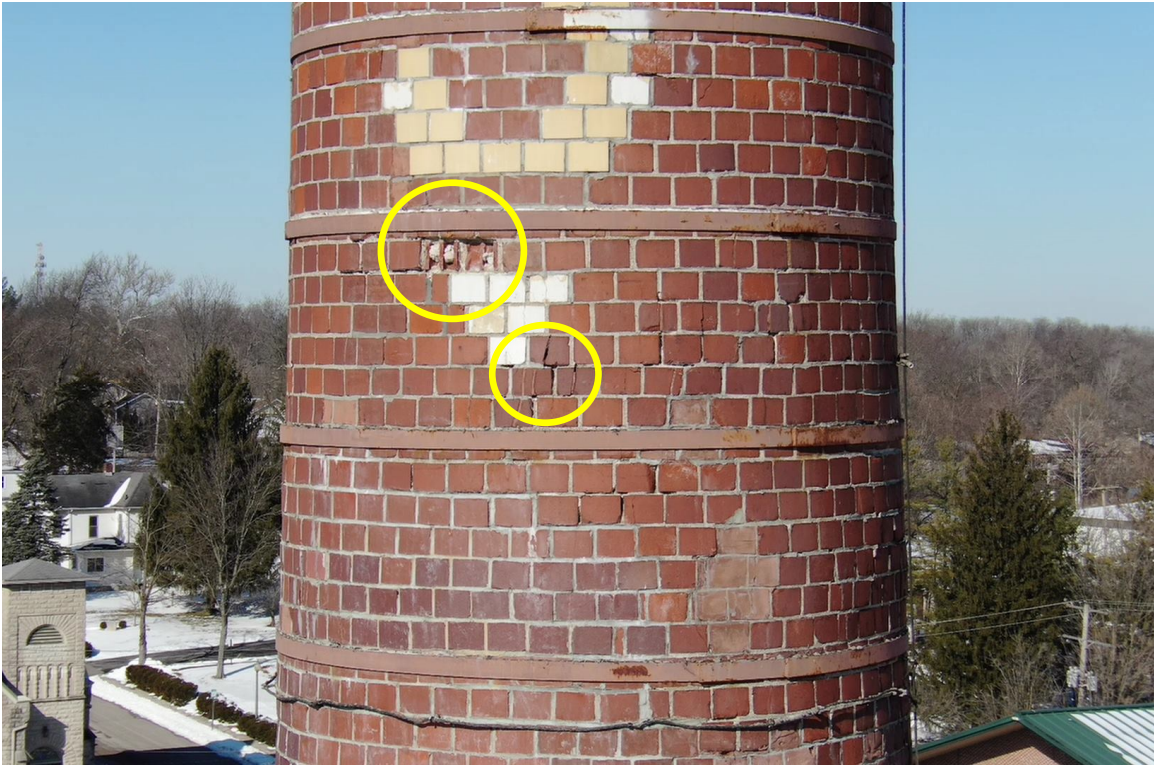
Photo 5 New spalls are highlighted in this 2022 photo.
