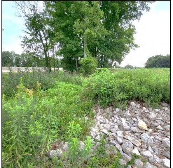
Photo 4: Rock check dam on the western Site boundary; View to the northwest
