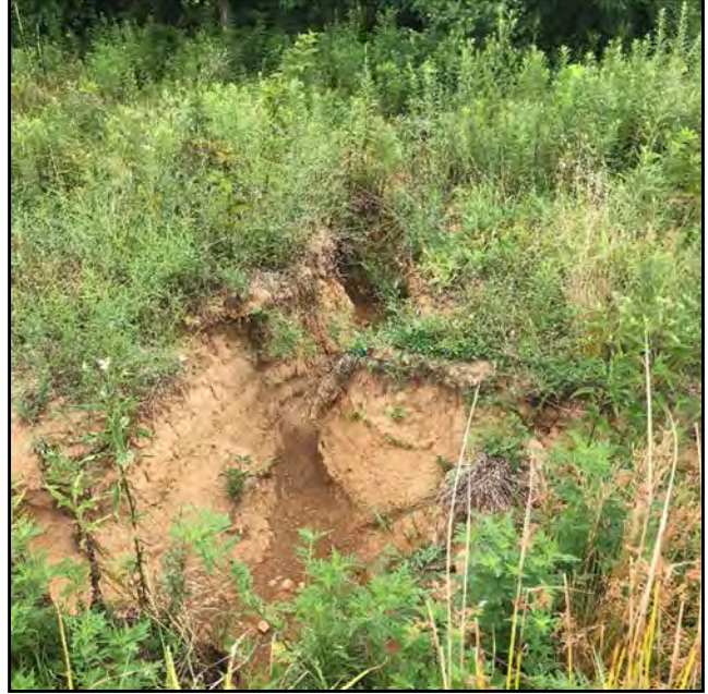
Photo 2: Erosional gulley west of southern wooded portion of Subject Property; View to the east
