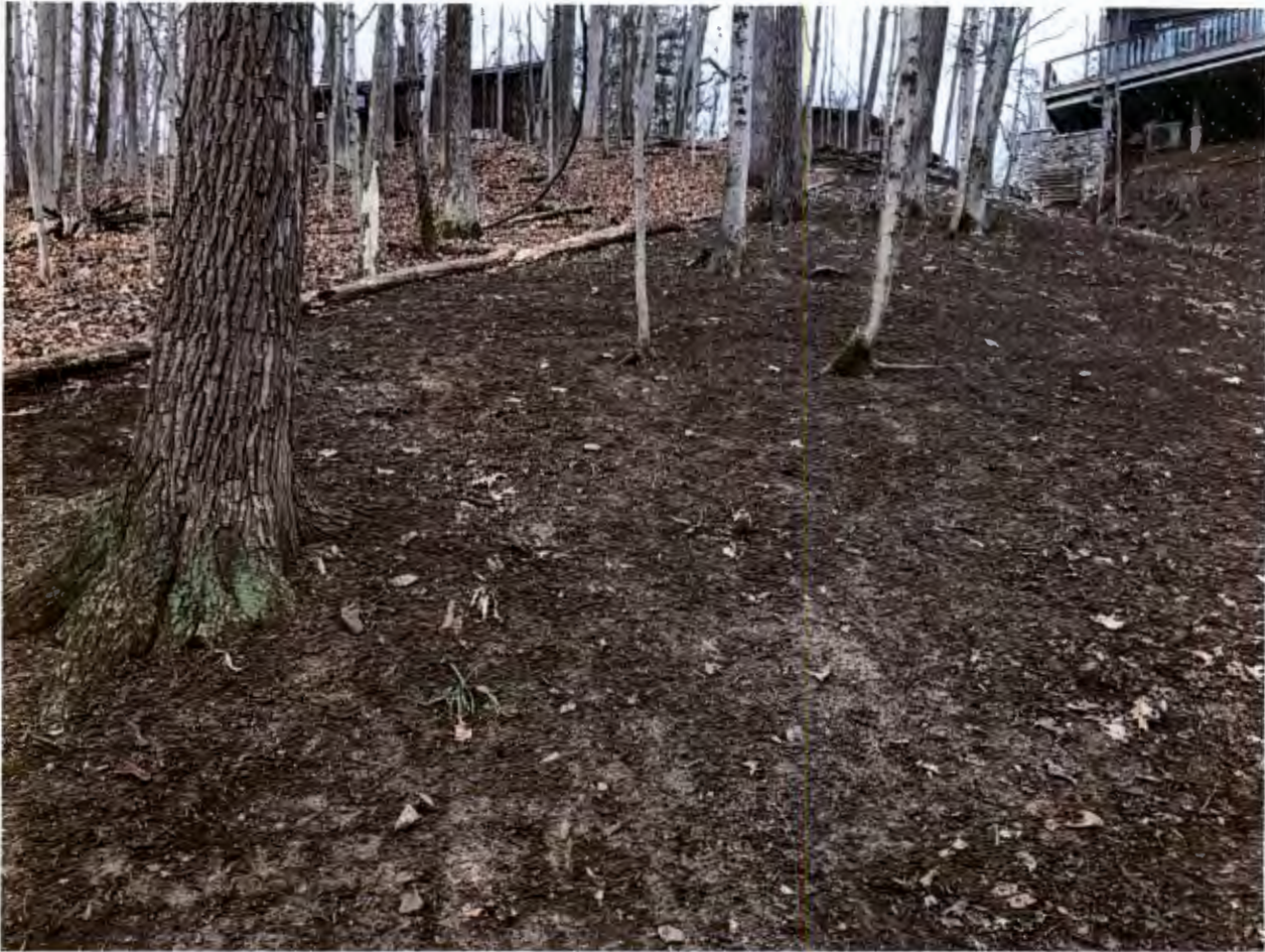
Photo 4: Disturbed land, including trees removed on steep slopes at 2408 S Shadow Grove Ct on 02/22/2024.
