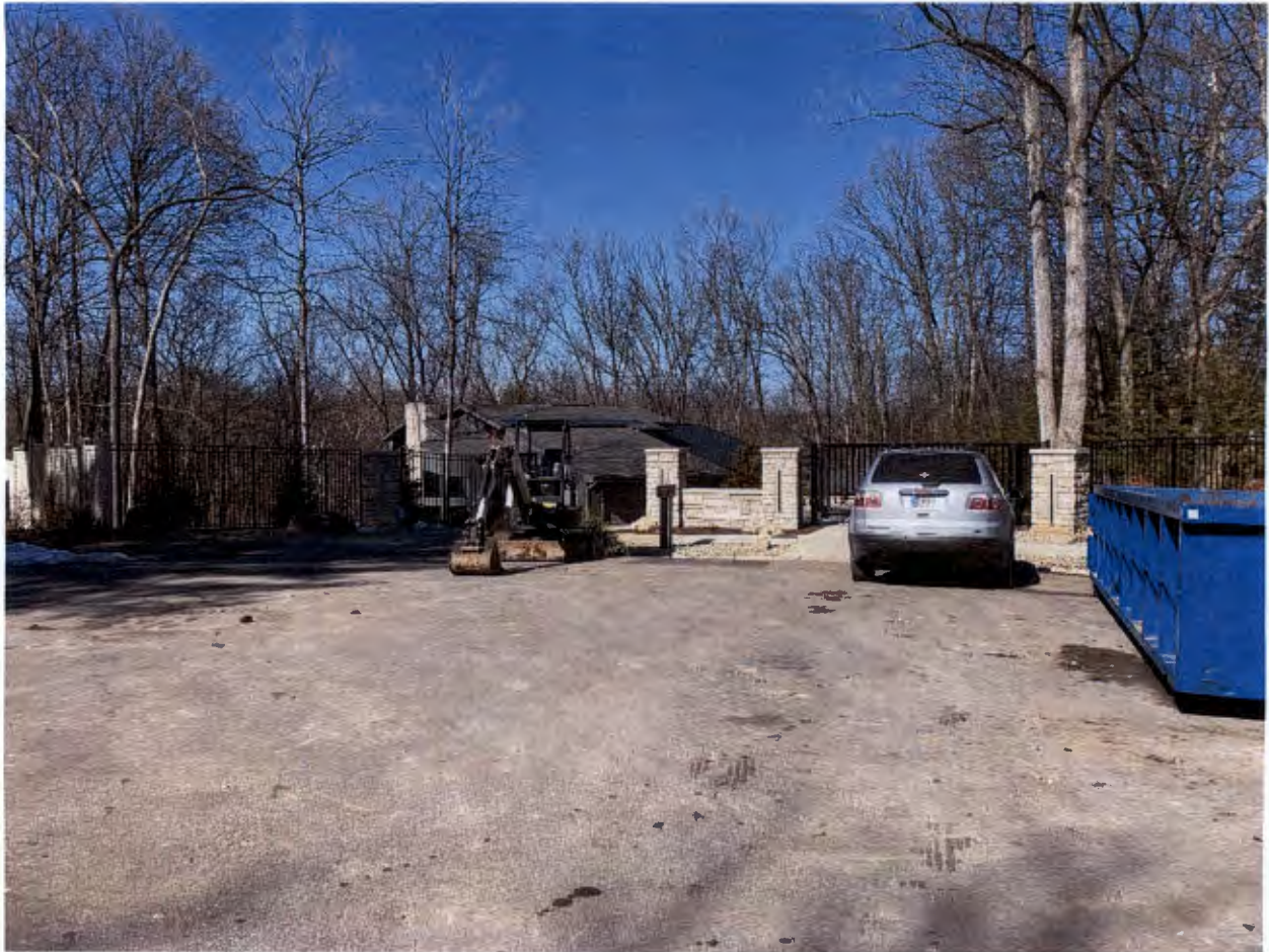
Photo 11: Tracking of sediment from the property into the roadway and fencing exceeding 4 feet in height forward of the front building wall at 2408 S Shadow Grove Ct on 02/20/2024.
