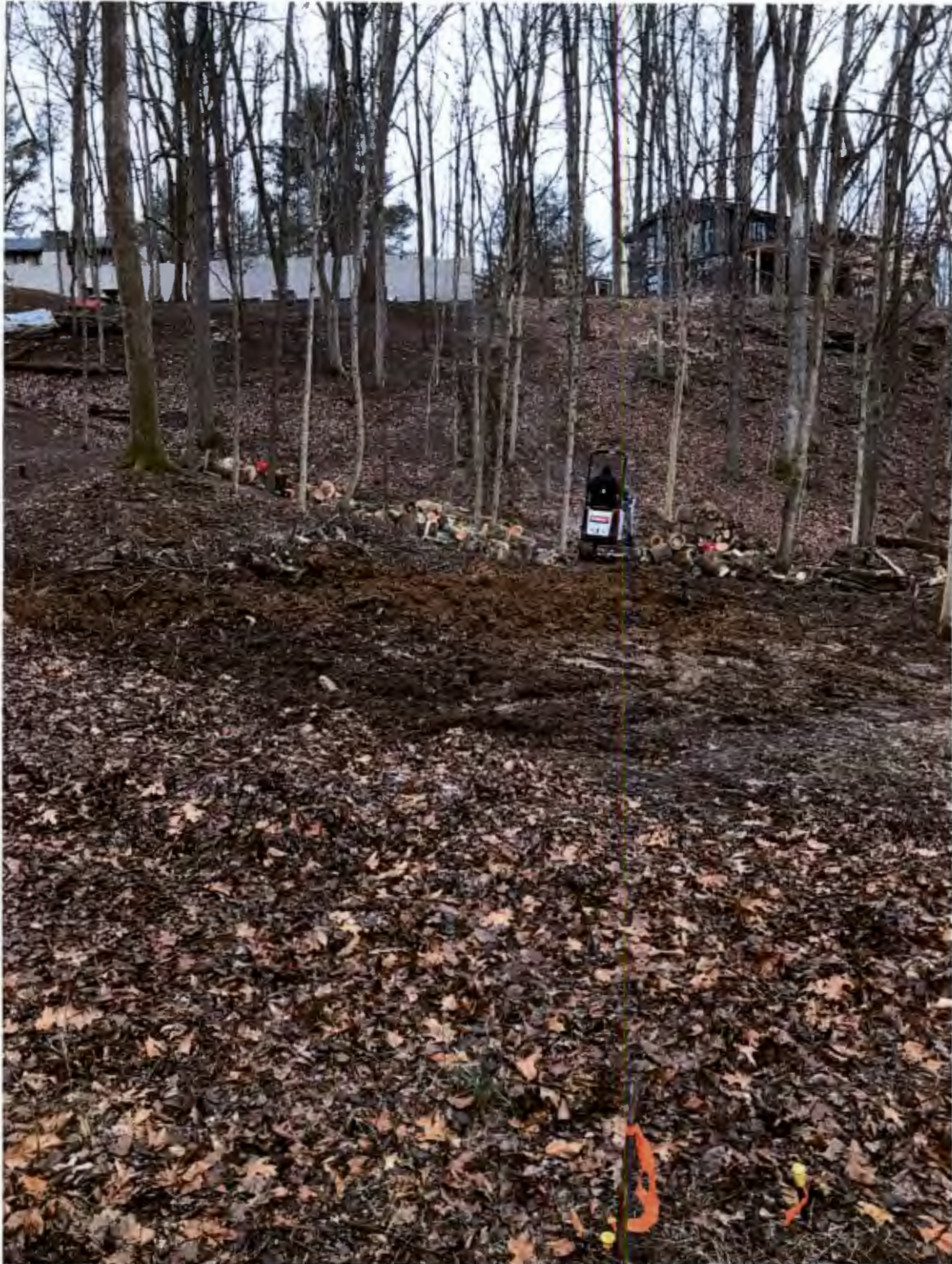
Photo 6: Disturbed land and land disturbing activity, including the removal and burying of trees, and lack of erosion controls installed at 2408 S Shadow Grove Ct on 02/22/2024.
