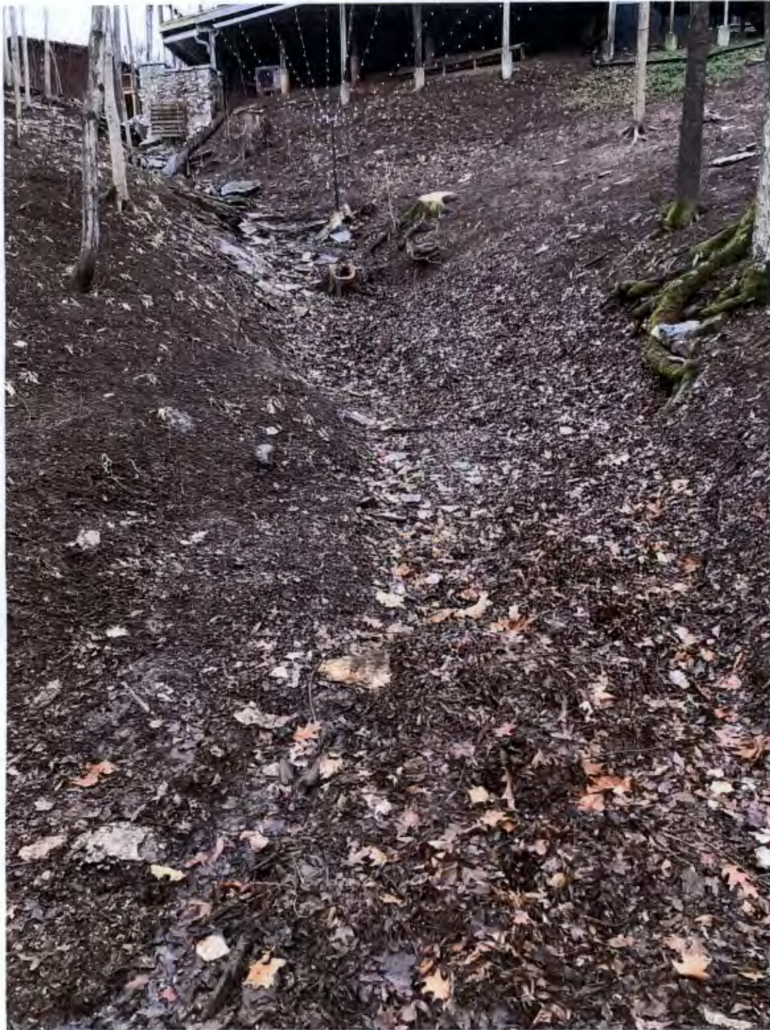
Photo 5: Lighting fixtures (string lights with bulbs not shielded) and disturbed land, including trees removed on steep slopes at 2408 S Shadow Grove Ct on 02/22/2024.
