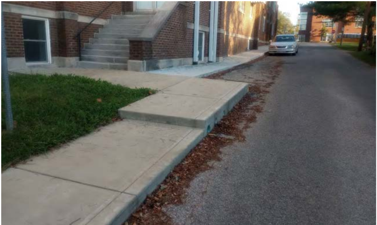
Existing partial pedestrian route on the west side of Jackson Street from 6th Street to 7th Street, second vertical step (looking south to north) 10/11/2024
