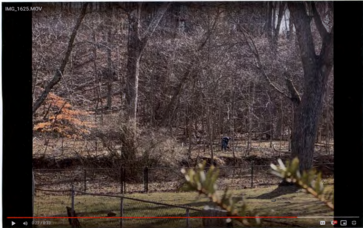
Photo 17: Screenshot of a video of a chainsaw being used to remove and chop up vegetation in the floodplain and riparian buffer on City-owned property adjacent to 2408 S Shadow Grove Ct on 02/29/2024 after the Stop Work Order (SWO) was issued on 02/22/2024.
