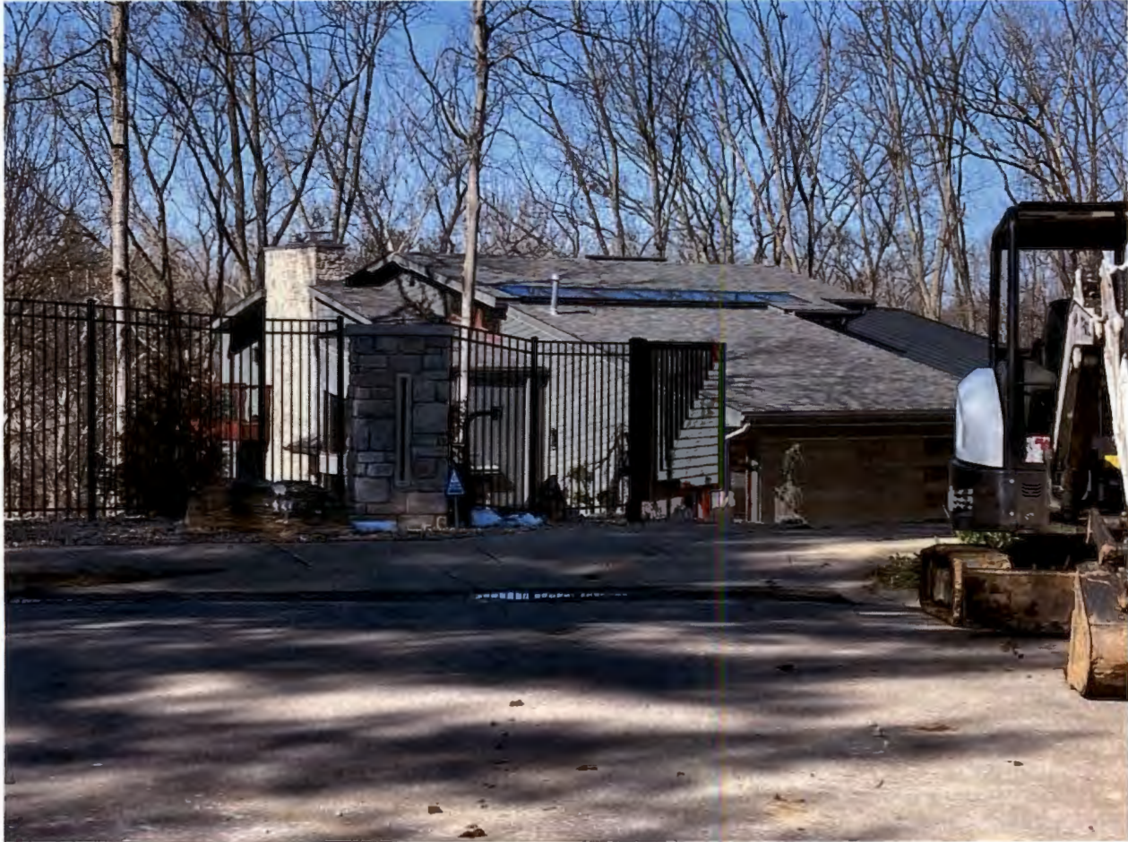
Photo 10: Tracking of sediment from the property and into the roadway at 2408 S Shadow Grove Ct on 02/20/2024.
