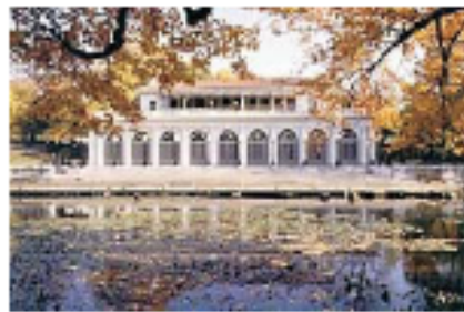
PHOTO: Restoration of this historic terra cotta boathouse included use of ELASTOWALL 351 to match the original terra cotta glaze.
