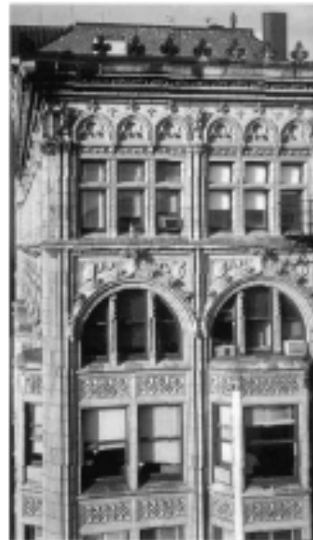
PHOTO: Repointing of Chicago's Historic Landmark Fisher Building with SPEC-JOINT 46 continued through severe winter conditions with the use of a proprietary non-chloride admixture approved by Edison Coatings, Inc.
