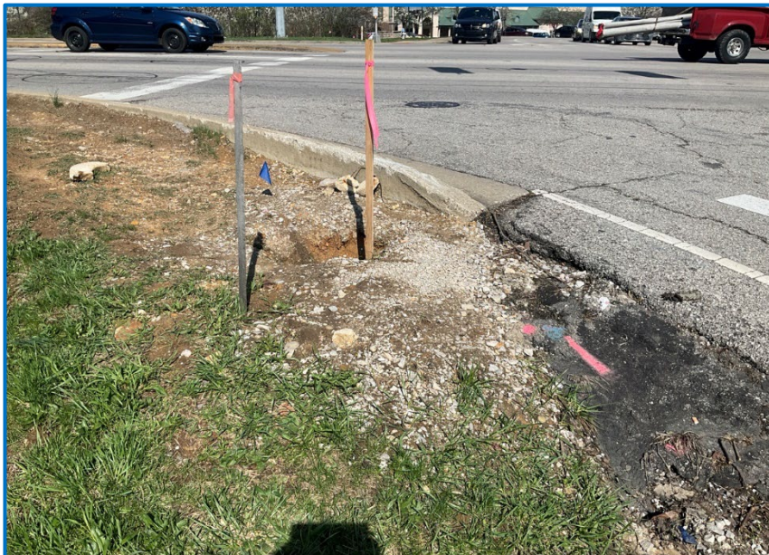
Photo 3 – View of deteriorated concrete at the southwest quadrant of the SR 45 Liberty Drive / South Hickory Leaf Drive intersection (04/01/2025).
