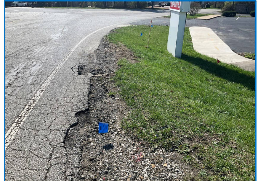
Photo 4 – View along South Hickory Leaf Drive from the southwest quadrant of the intersection, facing southeast (04/01/2025).
