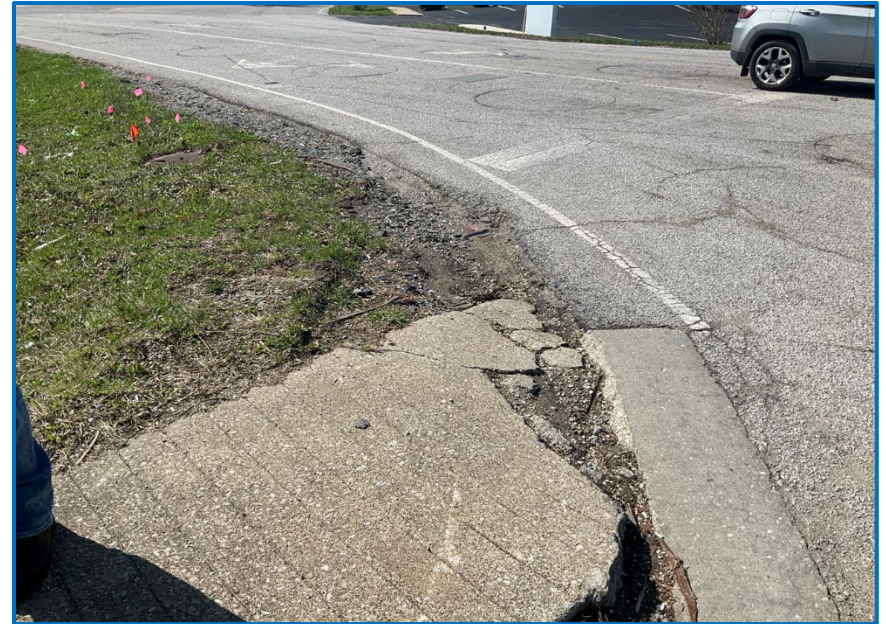
Photo 6 – View of deteriorated concrete curb at the southeast quadrant of the SR 45 and Liberty Drive/South Hickory Leaf Drive intersection (04/01/2025).
