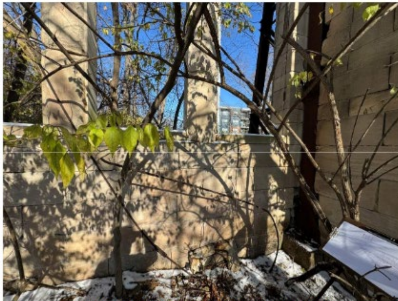
Photo 6: Southeast Corner Showing Condition of Limestone
