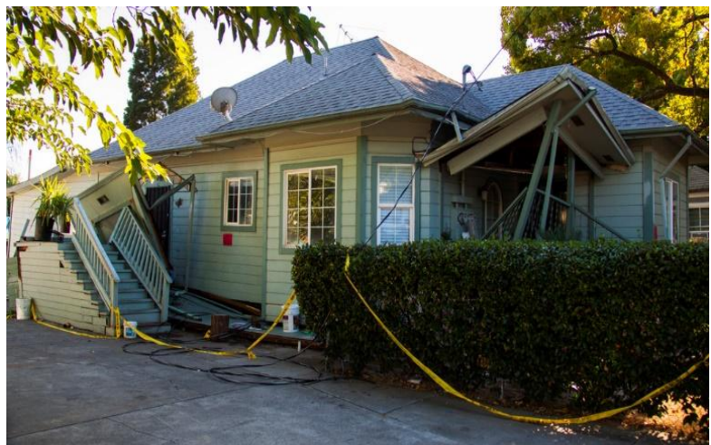
Figure 25 Structural Earthquake Damage
