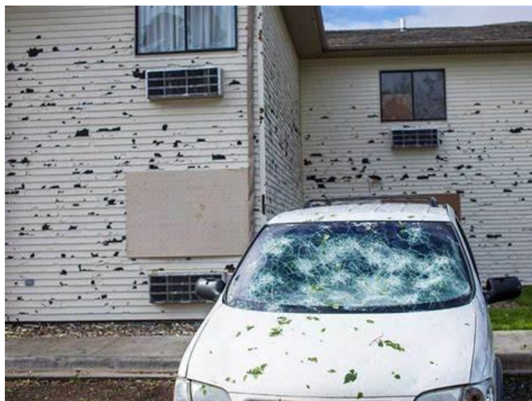
Figure 40 Damage to Vehicle and Structure Caused by Hail
