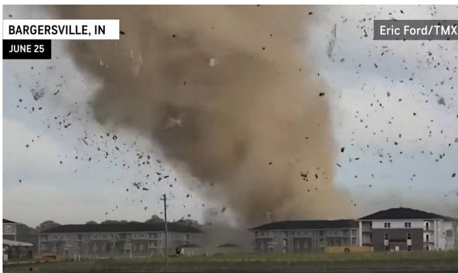
Figure 45 Debris Flying as Tornado Destroys Apartments under Construction
