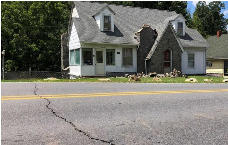
Figure 24 Minor Earthquake Damage
