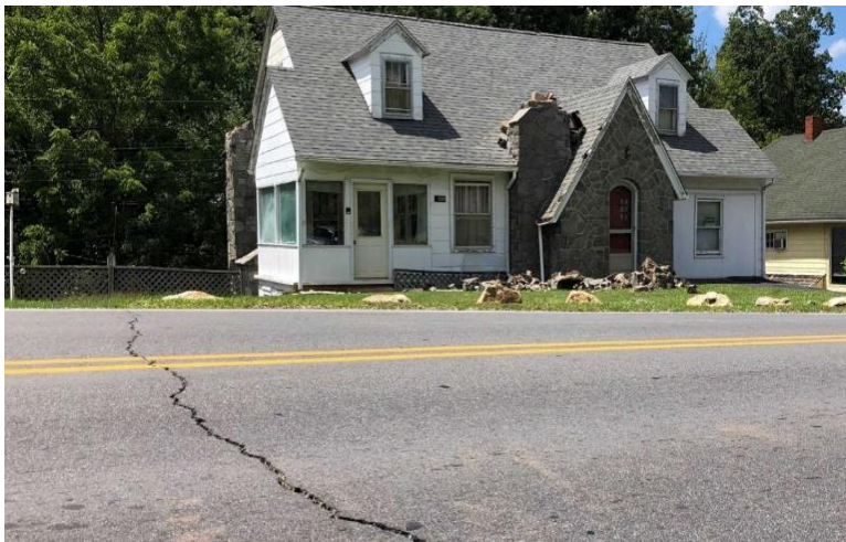
Figure 24 Minor Earthquake Damage
