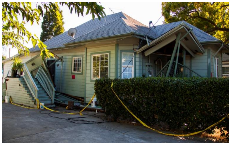
Figure 25 Structural Earthquake Damage
