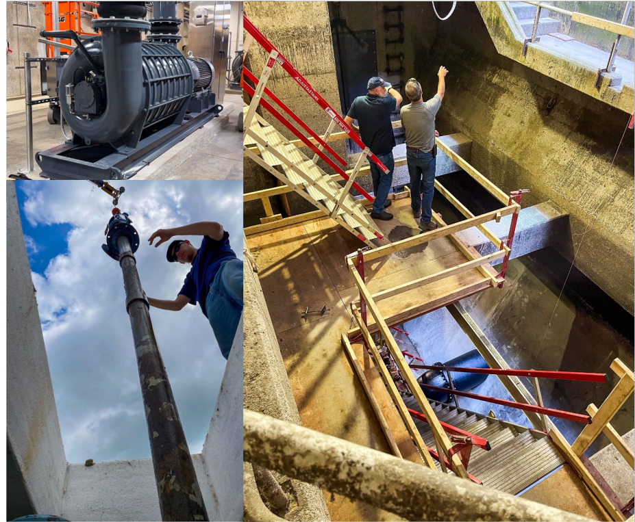
Top Left: Blower #5 - Bottom Left: Non-potable water pumps - Right: Suction lines in pump station
