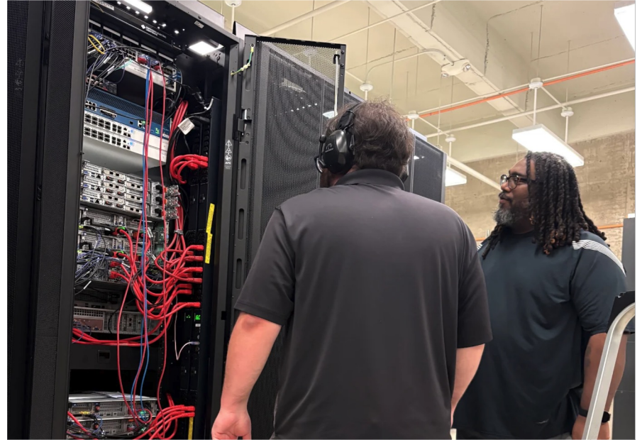
ITS Infrastructure team at the IU Datacenter
