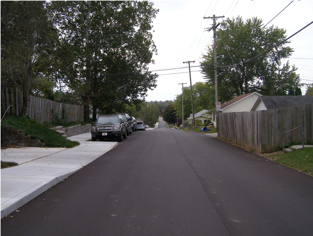
Looking south along S. Fairview Street from Wylie Street (~24). The new parking bump-outs and sidewalk can be seen on the left of the photo (east-side of street).
