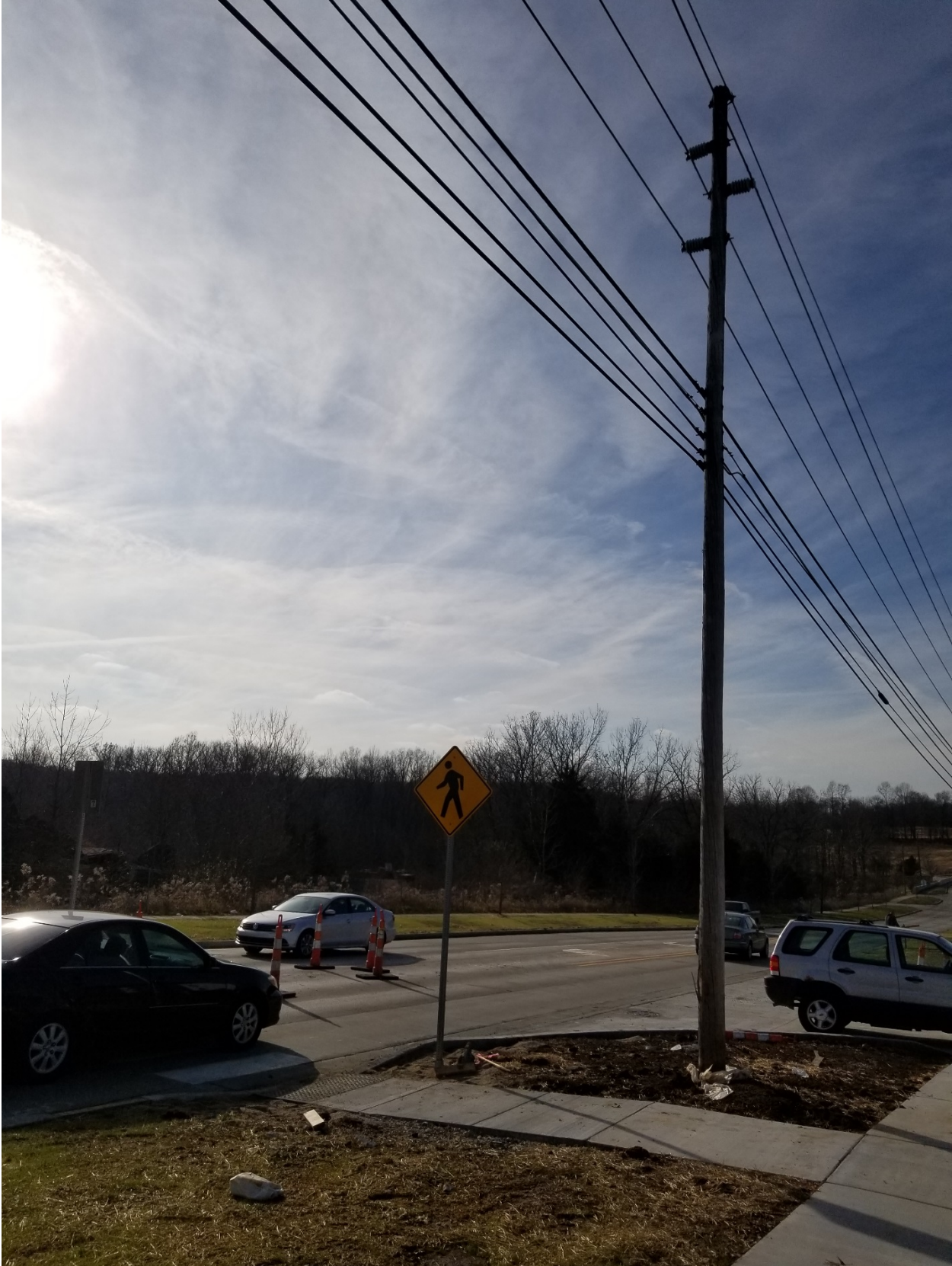
Roadway LED 110 Watt Fixture Mounted on Existing Wooden Pole to Illuminate Pedestrian Crossing Along W. Tapp Road
