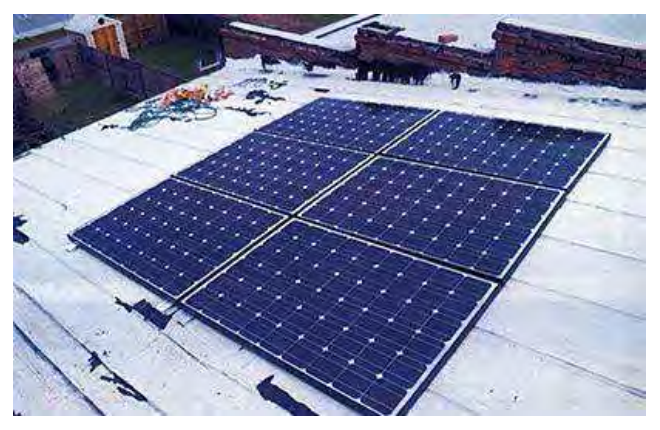
Recommended Solar panels were installed appropriately on the rear portion of the roof on this historic row house that are not visible from the primary elevation.
