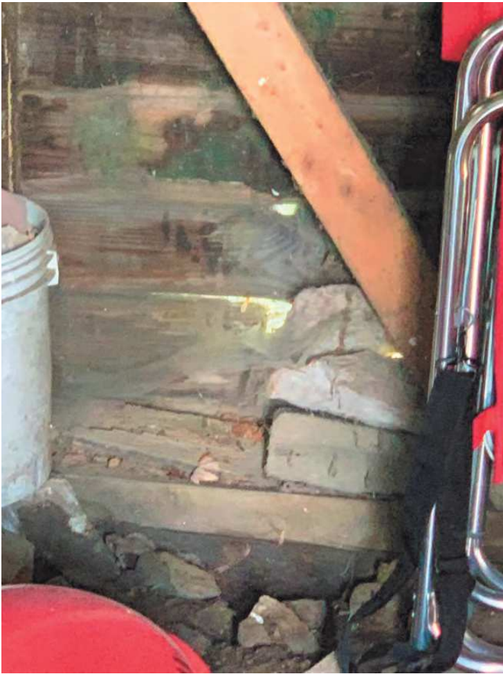
-Lack of foundation - rubble wall stack
