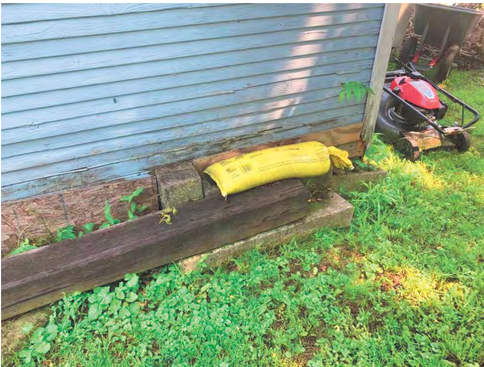
-Lack of foundation and lower wall rotted
