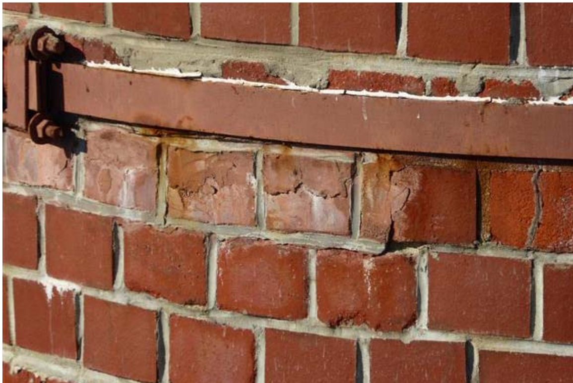
Photo 24 The patching material cracks and falls away itself.
