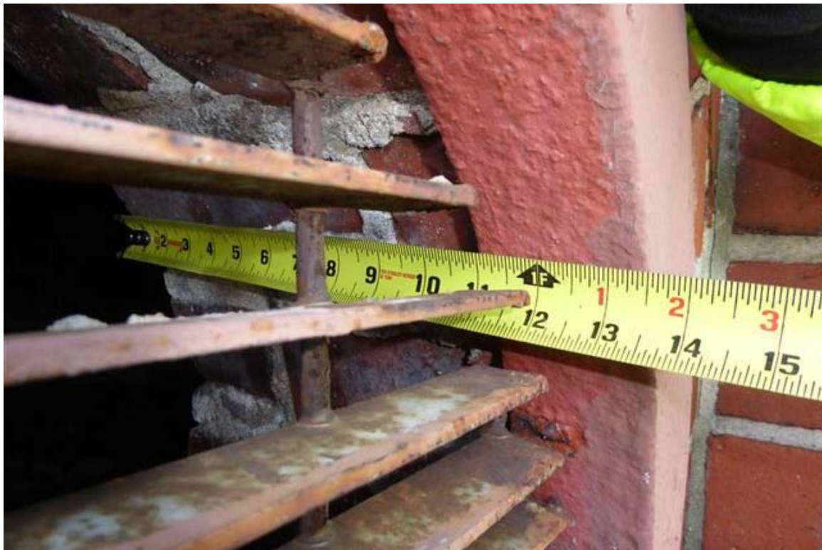
Photo 14 Wall thickness at the opening is 13 inches or 3 wythes of brick. This flares out to 5 wythes of brick or 20 inches in thickness on the sides of the opening.
