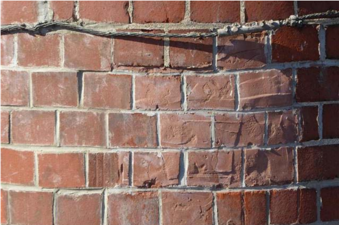
Photo 23 Cementitious patches have been used to replace spalled brick in numerous locations.
