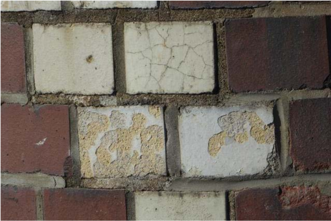
Photo 29 Glaze spalls continue to occur.
