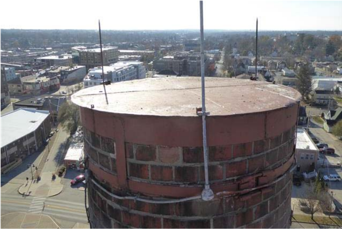
Photo 11 The top of the stack has been capped with a steel plate.
