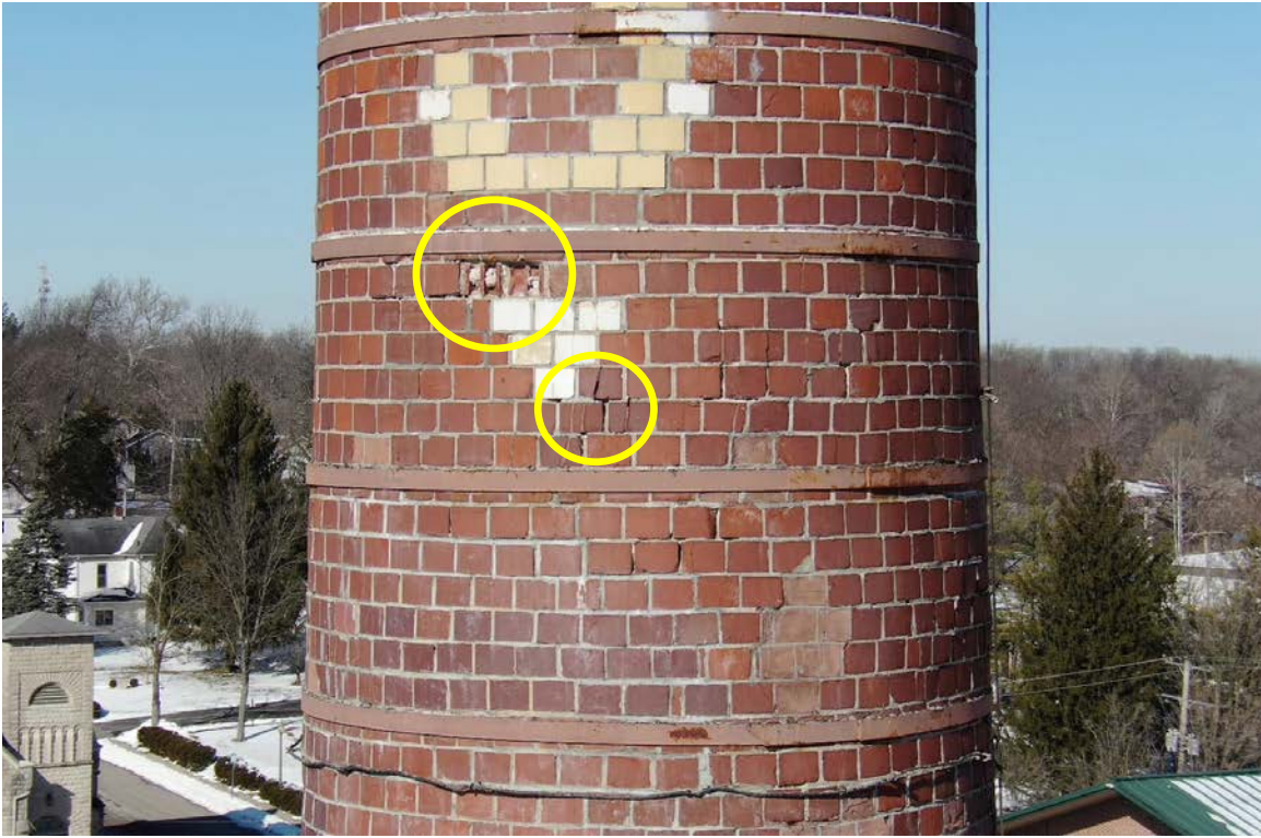
Photo 5 New spalls are highlighted in this 2022 photo.
