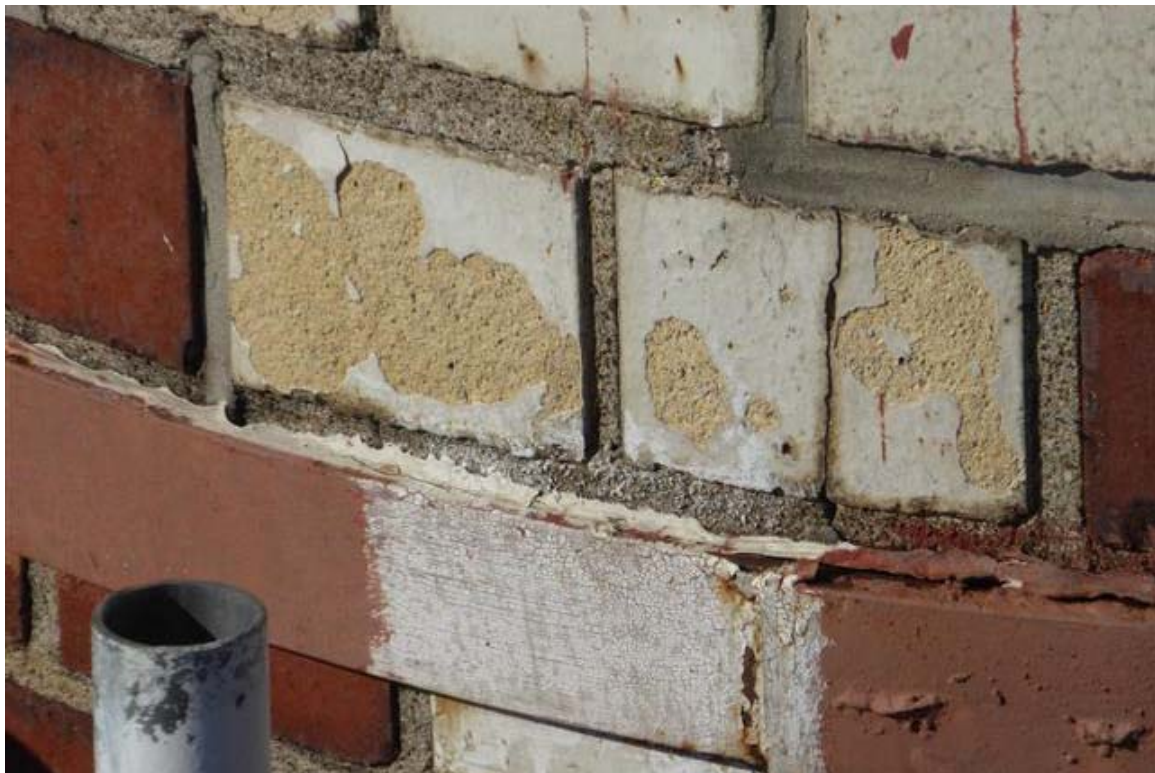
Photo 30 Similar condition in another location.
