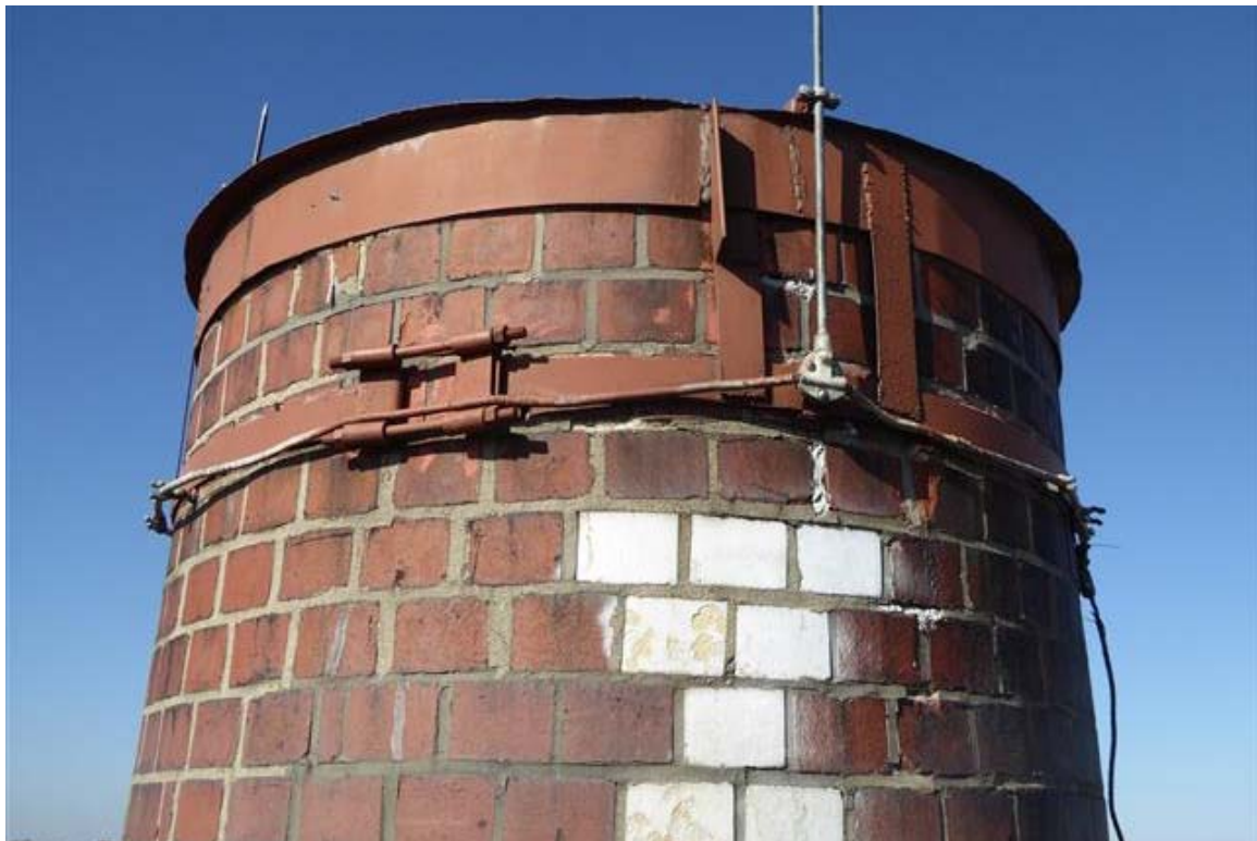
Photo 12 This prevents rain from falling inside but promotes freeze/thaw deterioration due to the “chimney effect” where warm, moist air rises and condenses on the inside face of the masonry.
