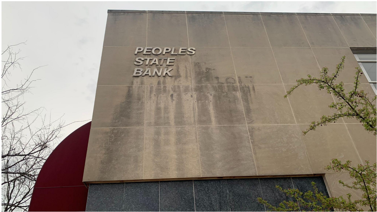
Figure 7: The lines and drilled holes from the original sign create a palimpsest of the bank's original name.
