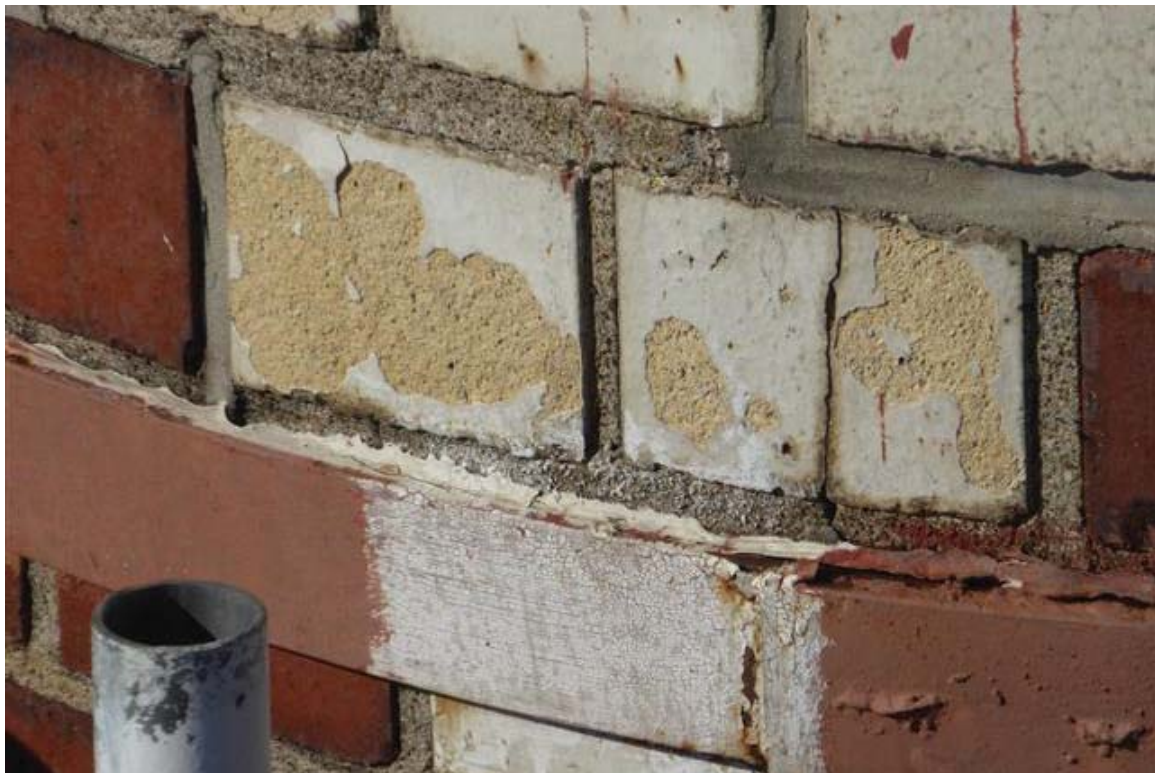
Photo 30 Similar condition in another location.
