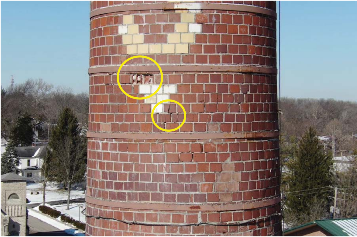
Photo 5 New spalls are highlighted in this 2022 photo.
