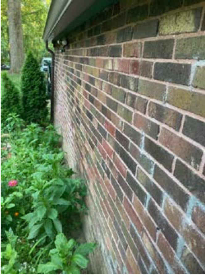
Existing bowing wall
