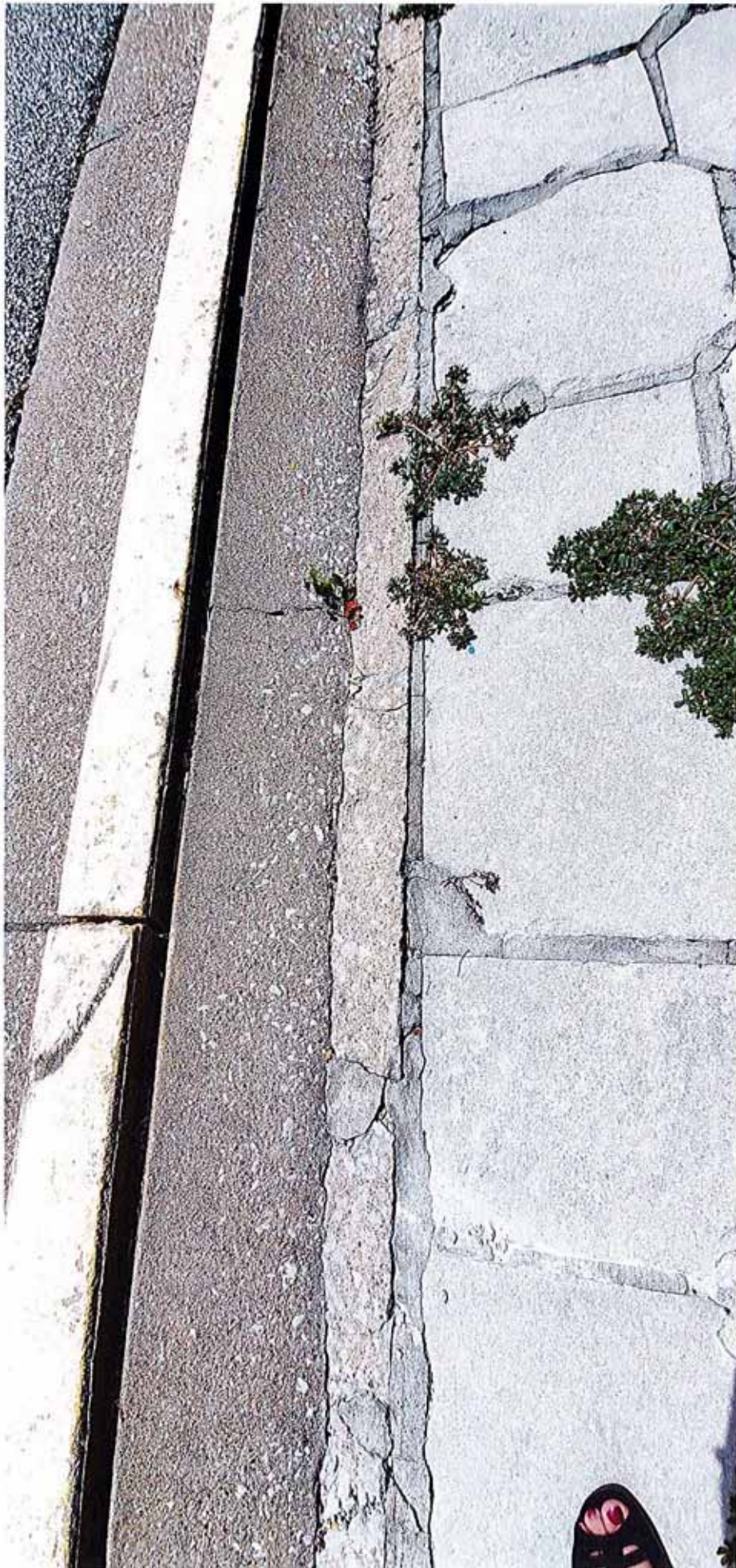
8 th St Sidewalk to be renovated
