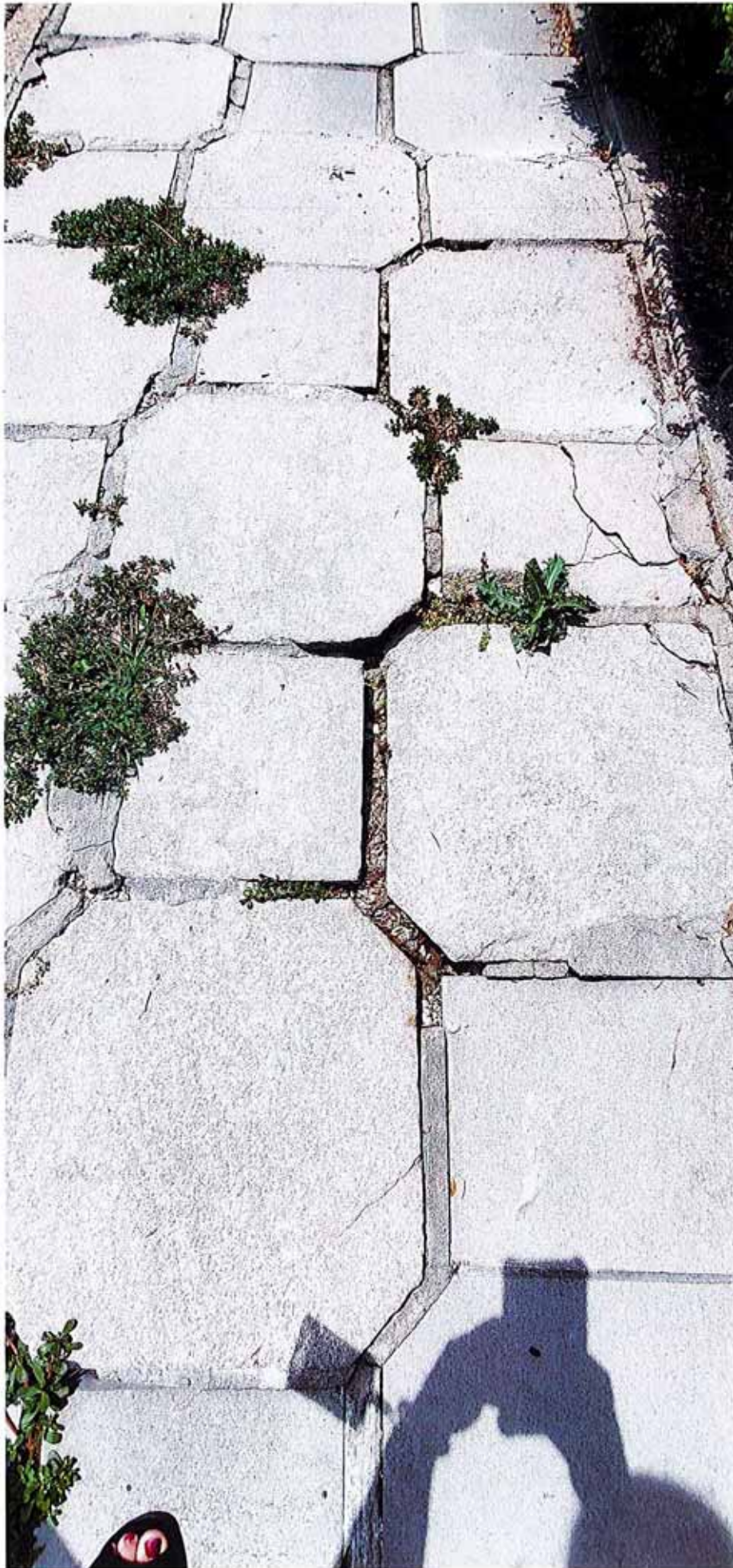
8th St WPA sidewalk disrepair
