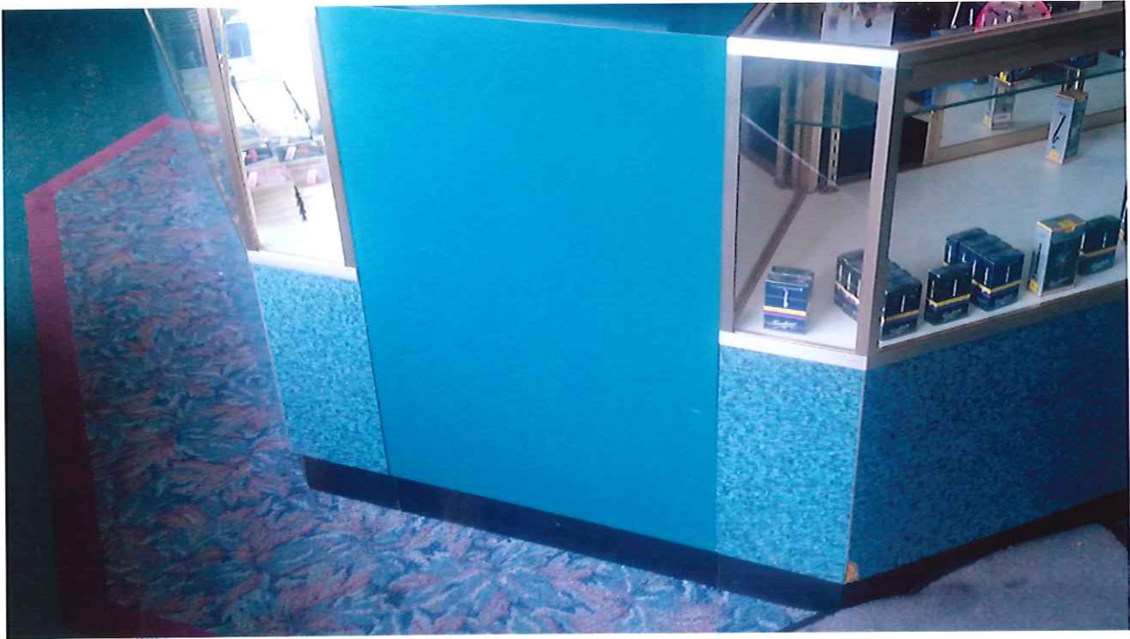
Fixtures worn and colors outdated
