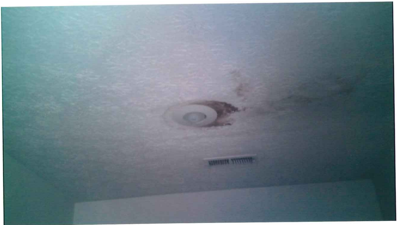
Water damage to ceilings
