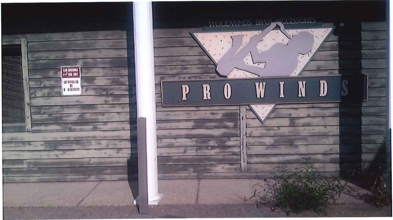
Paint of outside of building faded
