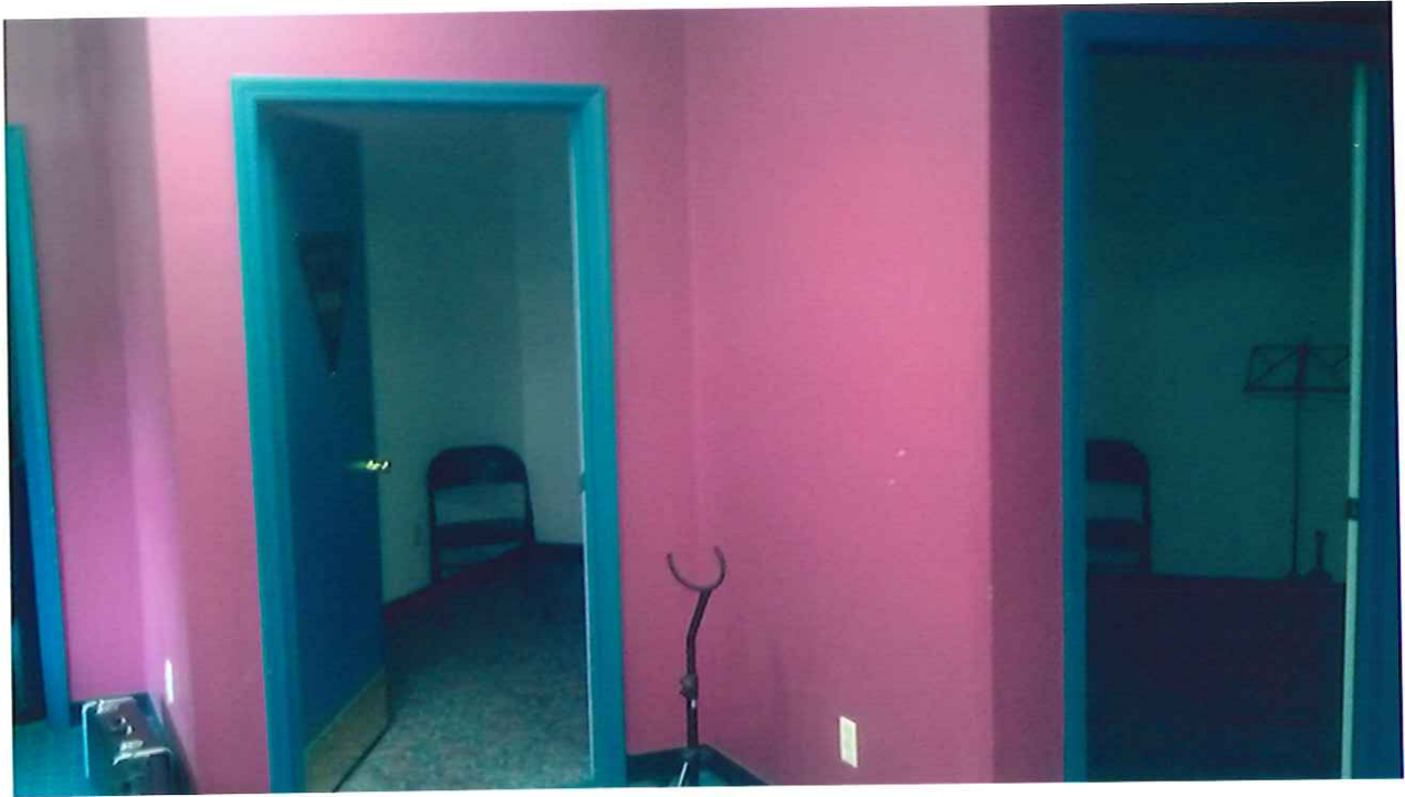
Inside paint colors outdated
