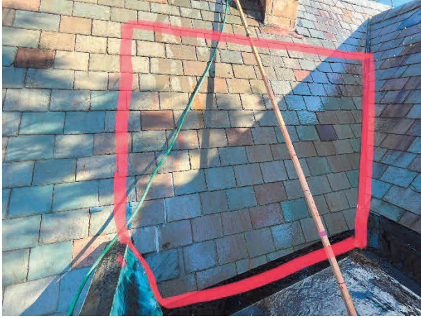
Slate to be removed, new ice and water shield installed, slate re-installed
