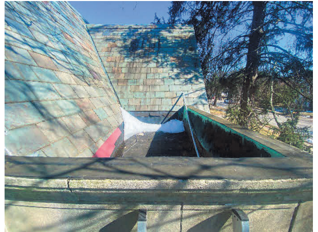
Copper to all be removed and replaced inside "pool" – detail on top of parapet coping to extend over edge 1"
