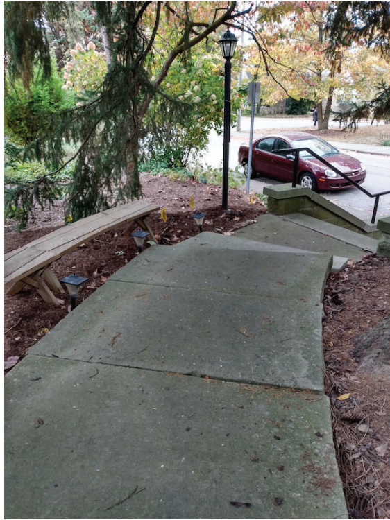
FIGURE 4. View of walkway in need of railing, which will be near bench.
