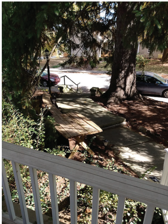
FIGURE 5. Alternate view of walkway in need of railing (on the left side of walkway in the photo).
