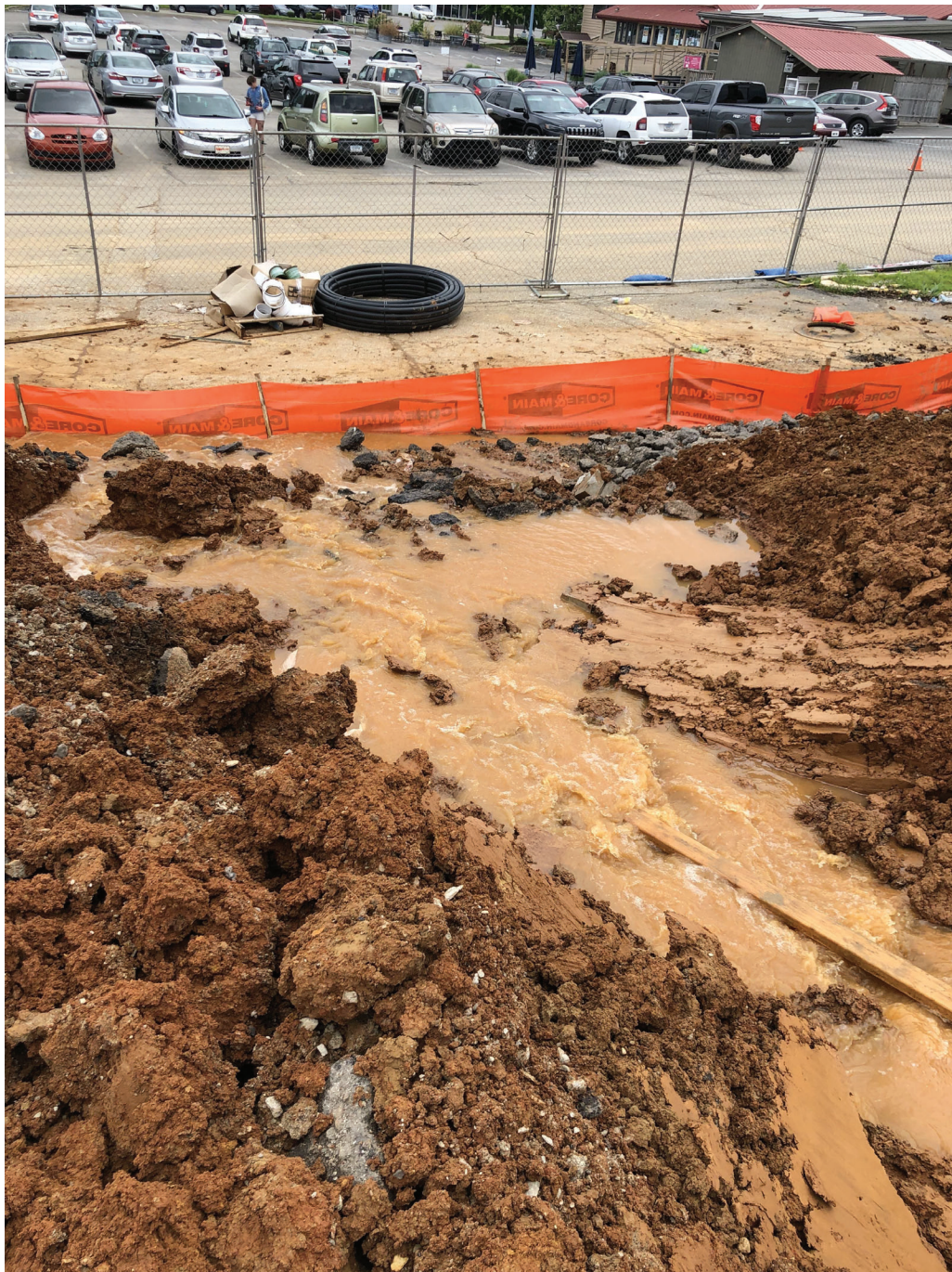
Sediment-laden water flowing off-site as sediment basins had not been constructed, per the construction sequence, to contain the water at 3216 E. 3rd Street on 06/07/2022.
