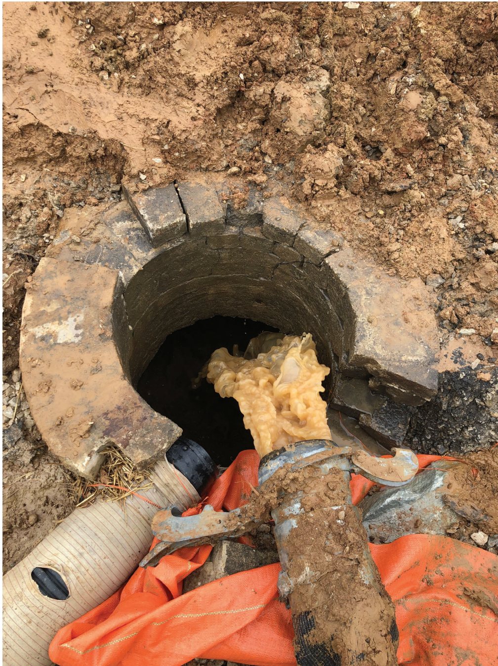
Sediment-laden water being pumped directly into a storm inlet as it cannot be contained on site at 3216 E. 3rd Street on 06/07/2022.
