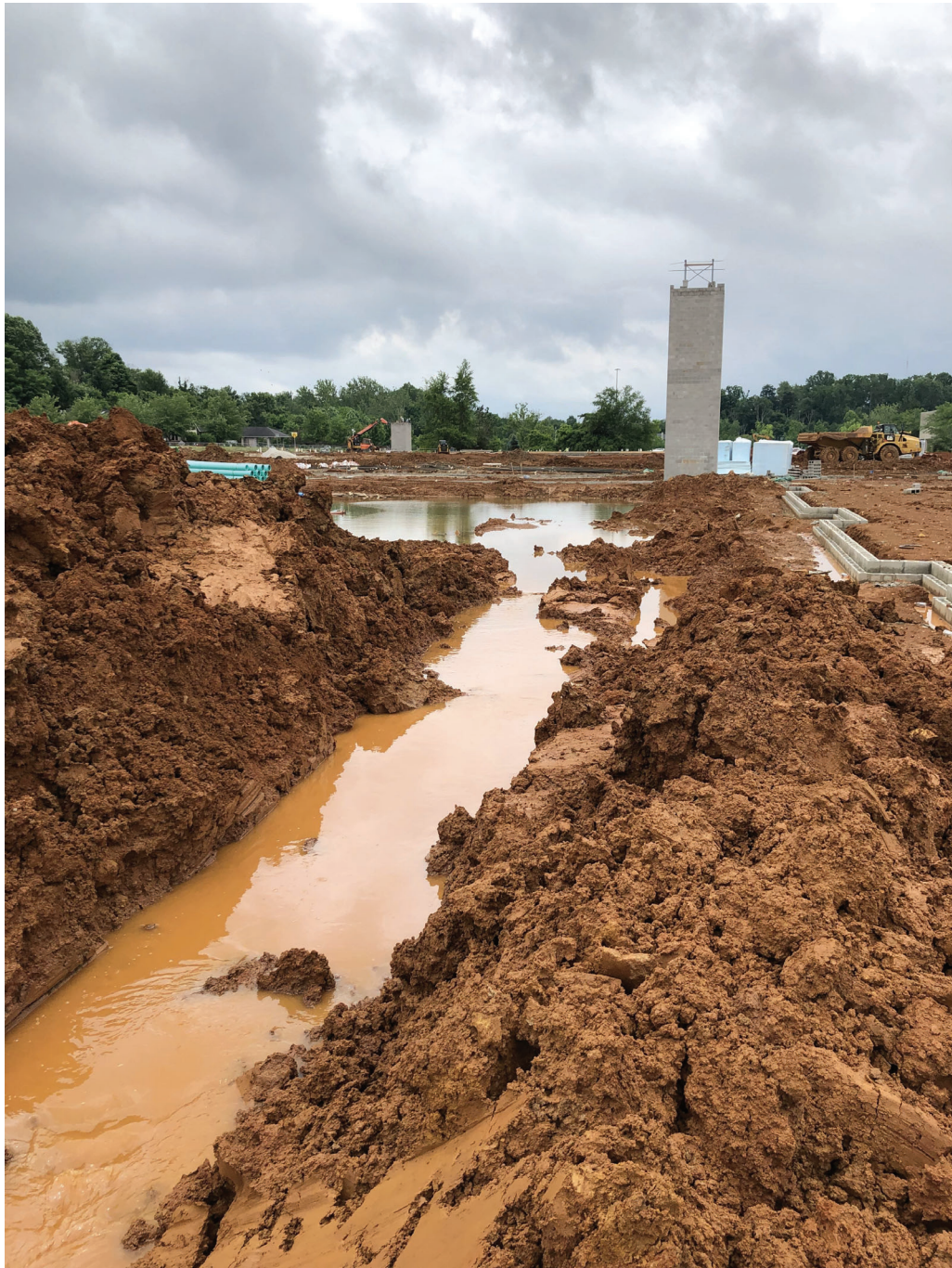
Sediment-laden water flowing across the site as sediment basins had not been constructed, per the construction sequence, to contain the water at 3216 E. 3rd Street on 06/07/2022.
