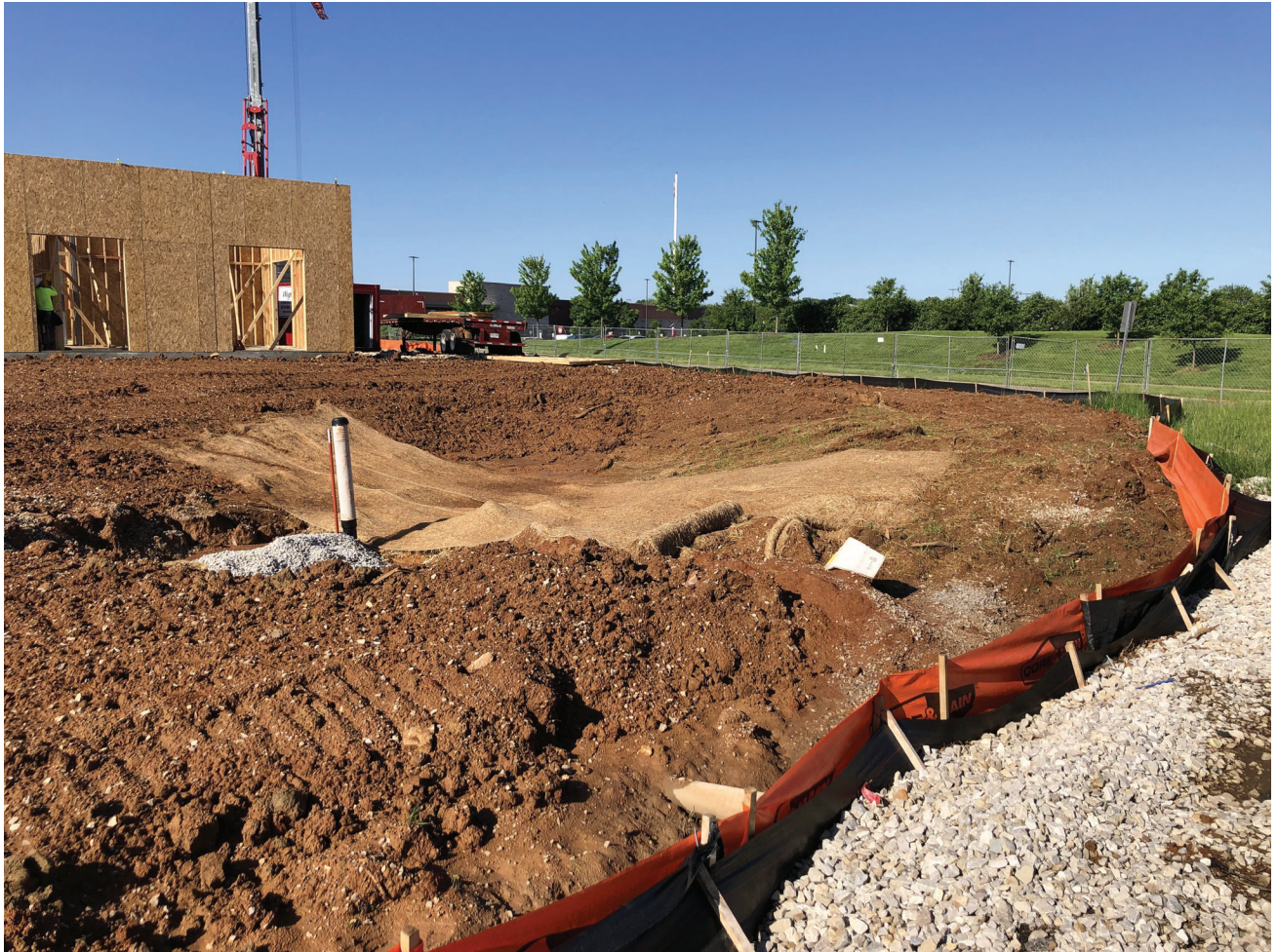
Incomplete and non-stabilized sediment basin at 3216 E. 3rd St on 05/16/2022.
