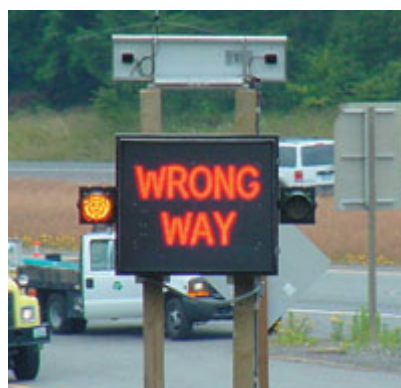
When the sensors determine a vehicle is traveling the wrong way, the message sign illuminates a red "Wrong Way" message (right).
