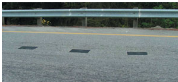
Electromagnetic sensors embedded in the pavement (the three dark squares) detect vehicles moving in the wrong direction (above).
