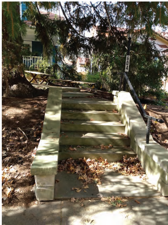
FIGURE 3. View from street of entry stairway and walkway in need of railing.
