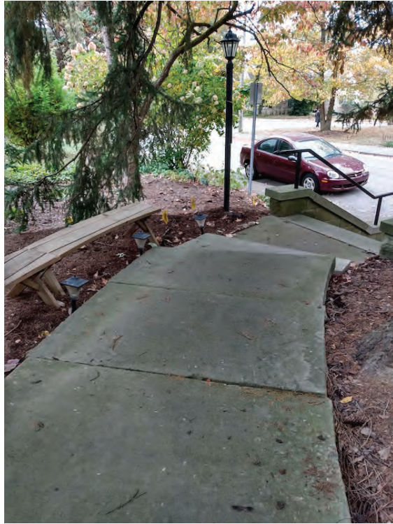
FIGURE 4. View of walkway in need of railing, which will be near bench.
