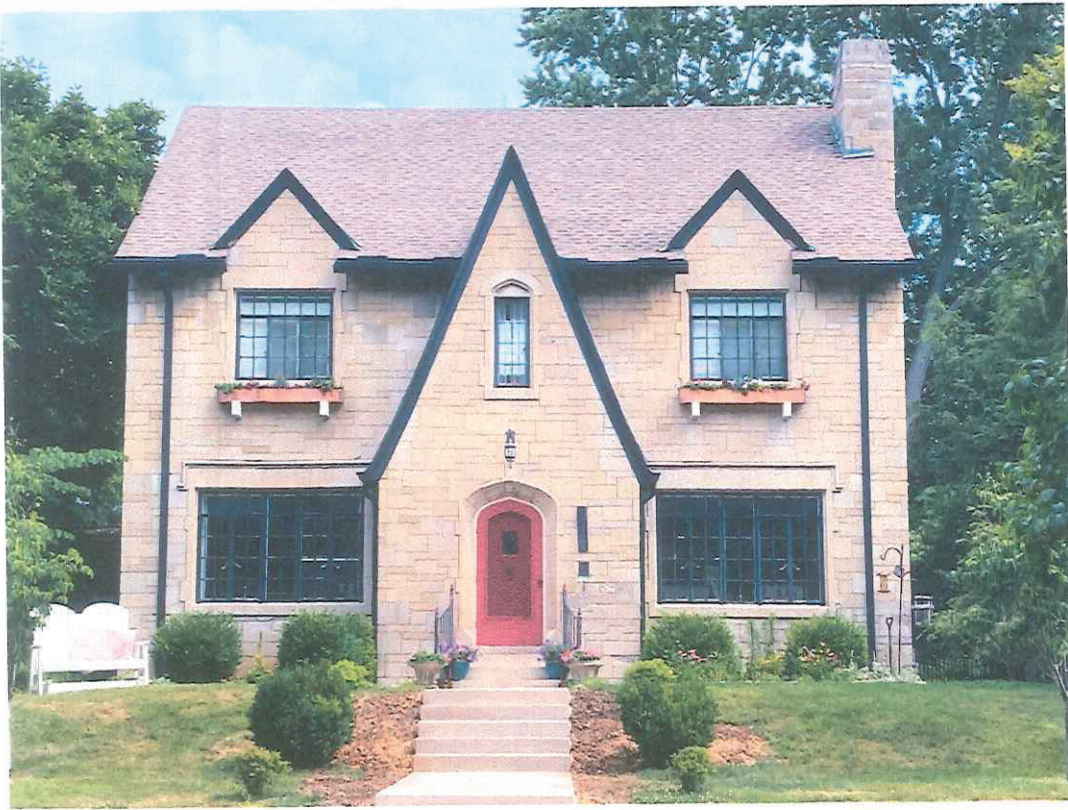
Existing House with damaged asphalt shingles
