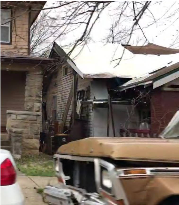
Photo from staff observation of 530 South Washington Street on 3/31/2022 documenting progress toward compliance.
