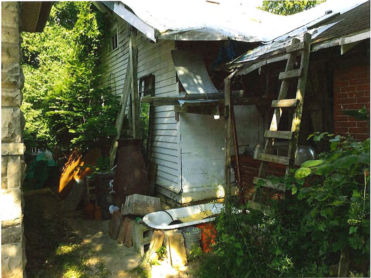
Photo 1: Building materials stored outdoors at 530 S. Washington Street on 08/09/2022.
