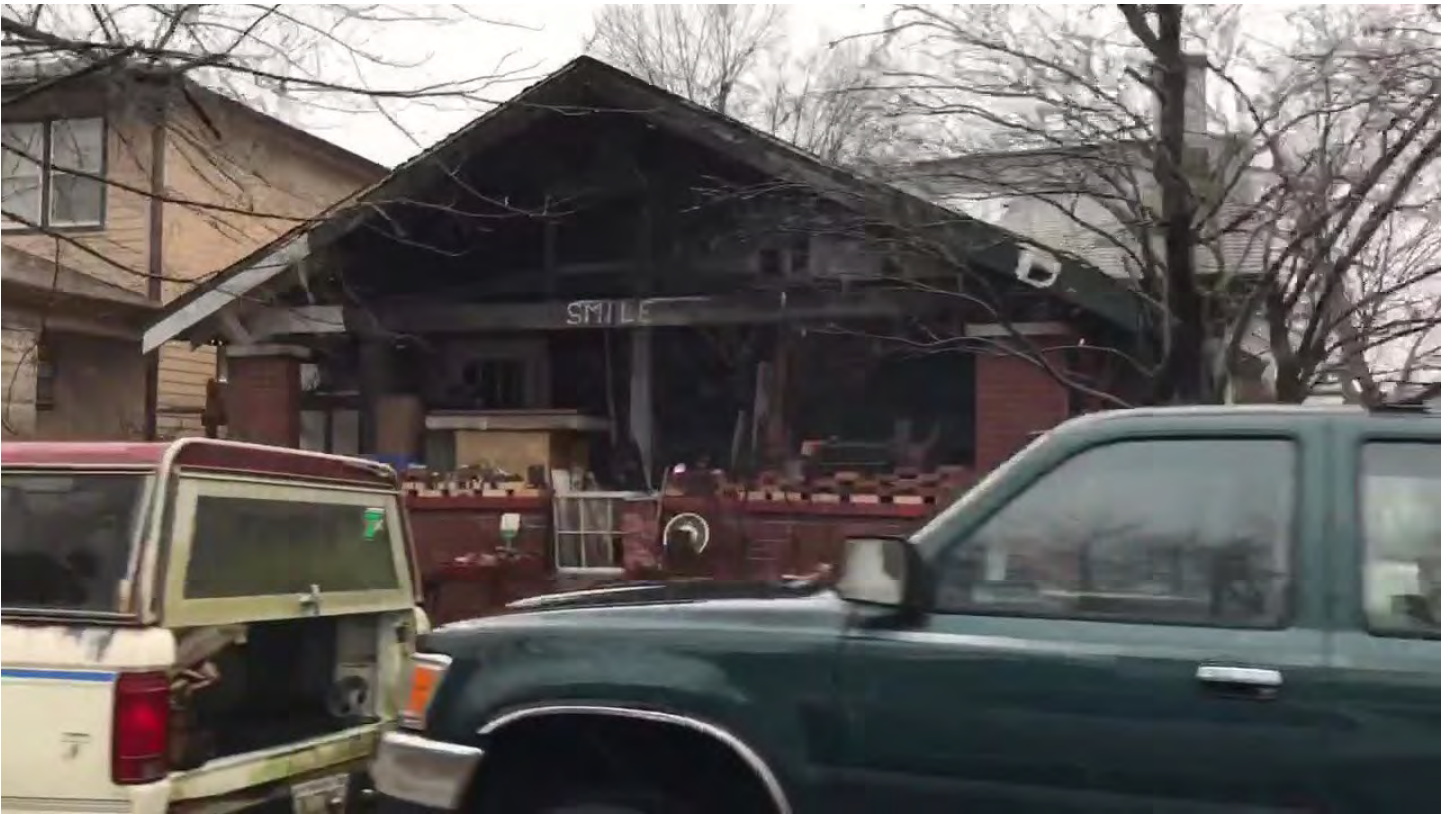
Photo from staff observation of 530 South Washington Street on 2/17/2022 documenting progress toward compliance.
