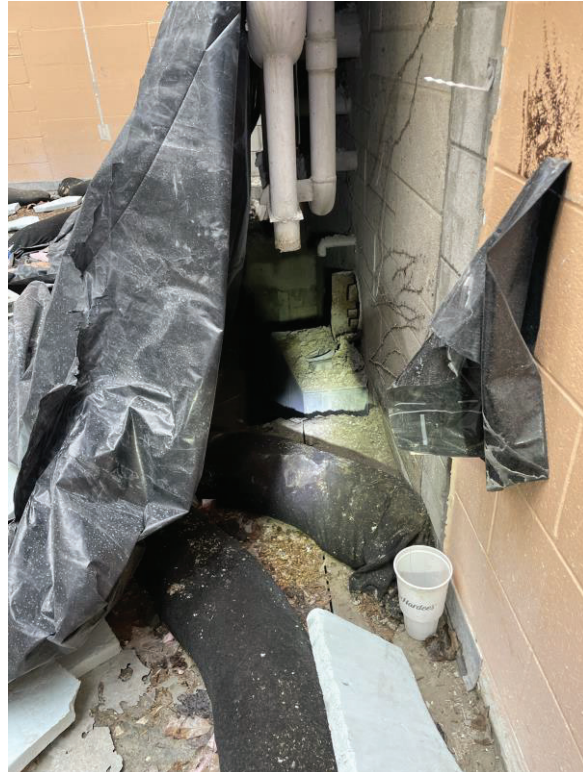
Photo 15. Mechanical Equipment Routed Through Wall
