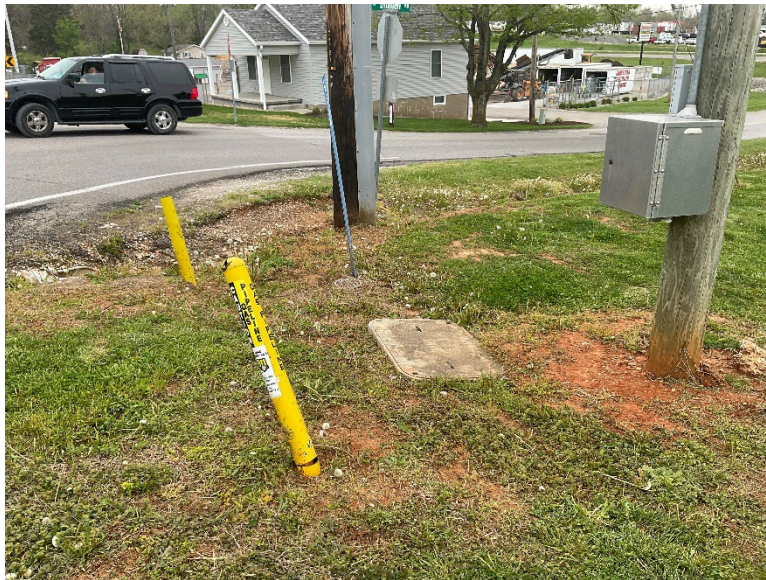
Utilities and Flasher Controller Cabinet in Northwest Quadrant of intersection
