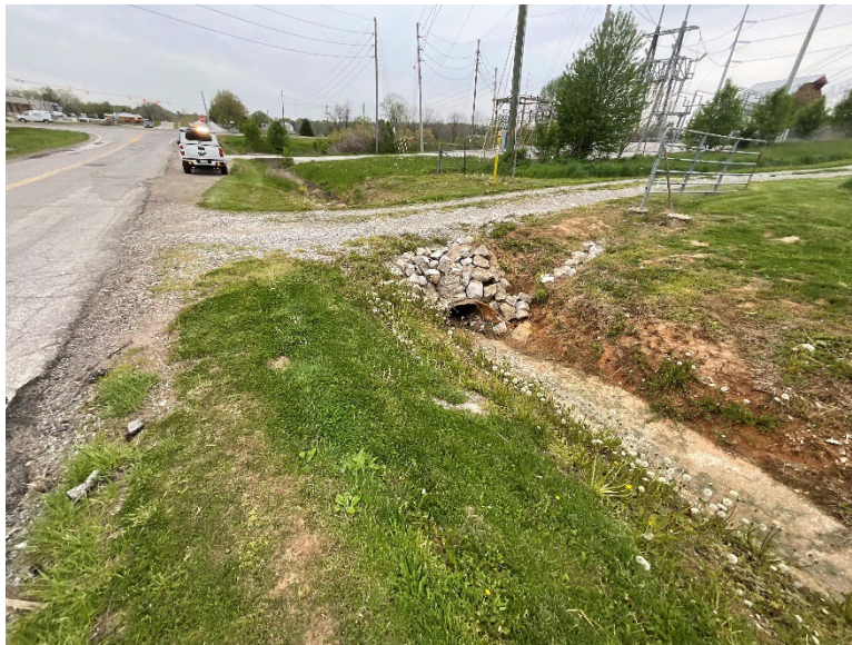
Driveway to Electric Substation on Northside of Dillman Road
