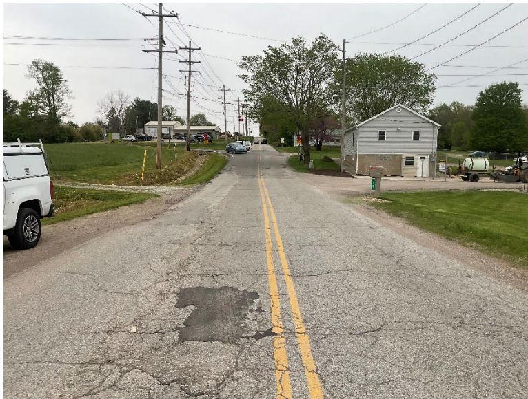
Dillman Road Pavement Conditions
