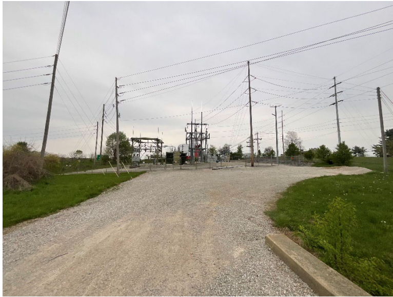
Electric Substation entrance off Dillman Road between SR 37 and Old SR 37
