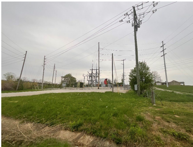
Electric Utility Substation and Overhead Electric lines Northwest Quadrant of intersection
