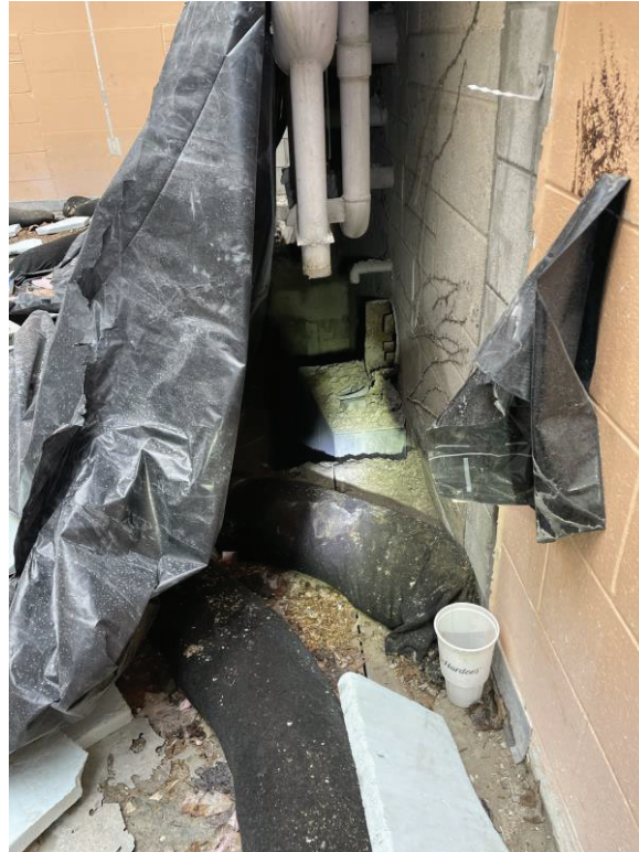
Photo 15. Mechanical Equipment Routed Through Wall
