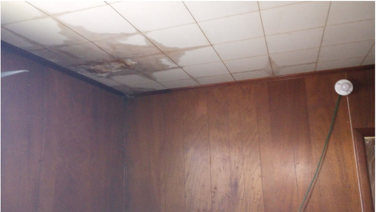
#8 Roof leak damage
