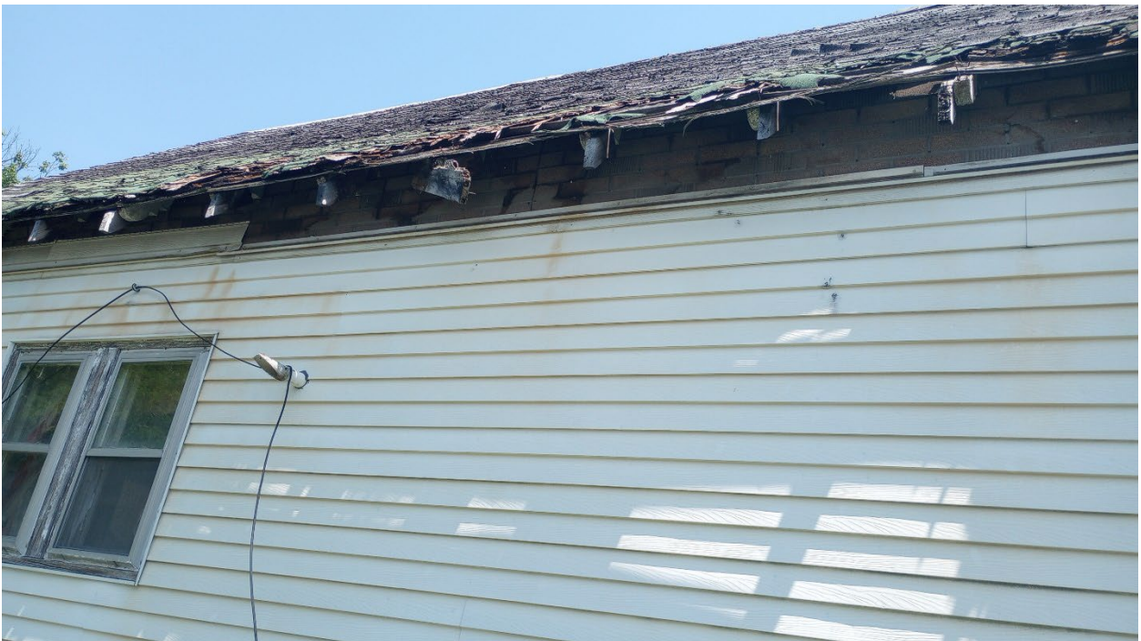
#2 Multiple shingle layers, warped decking, damaged rafter tails
