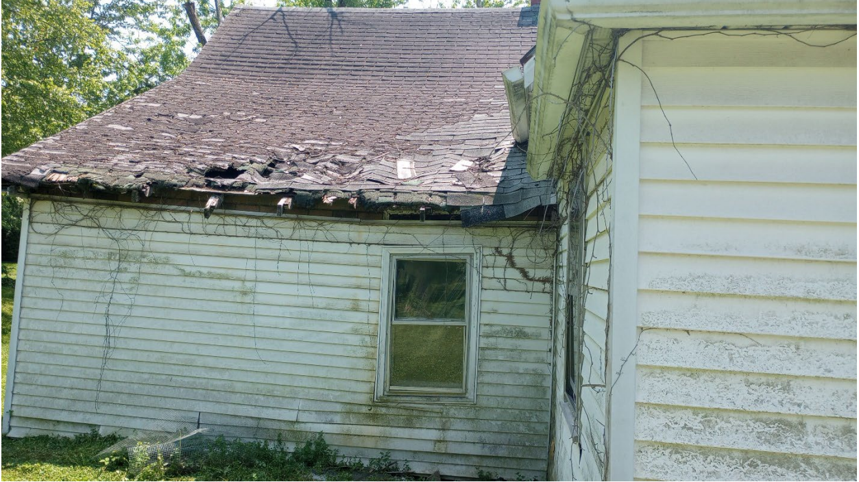
#3 Failed shed roof section above northeast room
