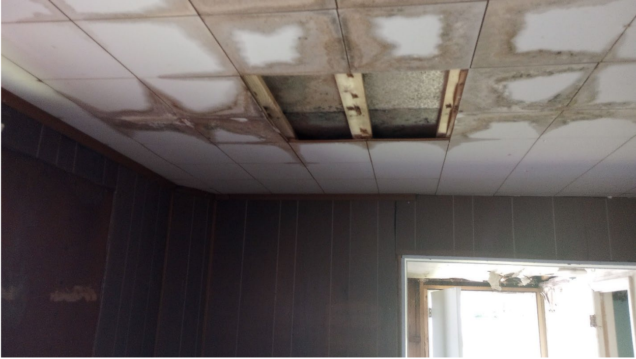
#9 Roof leak damage
