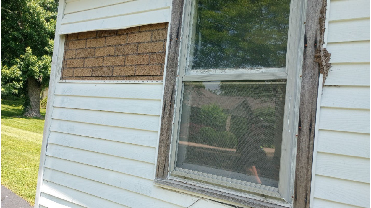
#5 Failed siding at northwest corner with "insulbrick" siding behind
