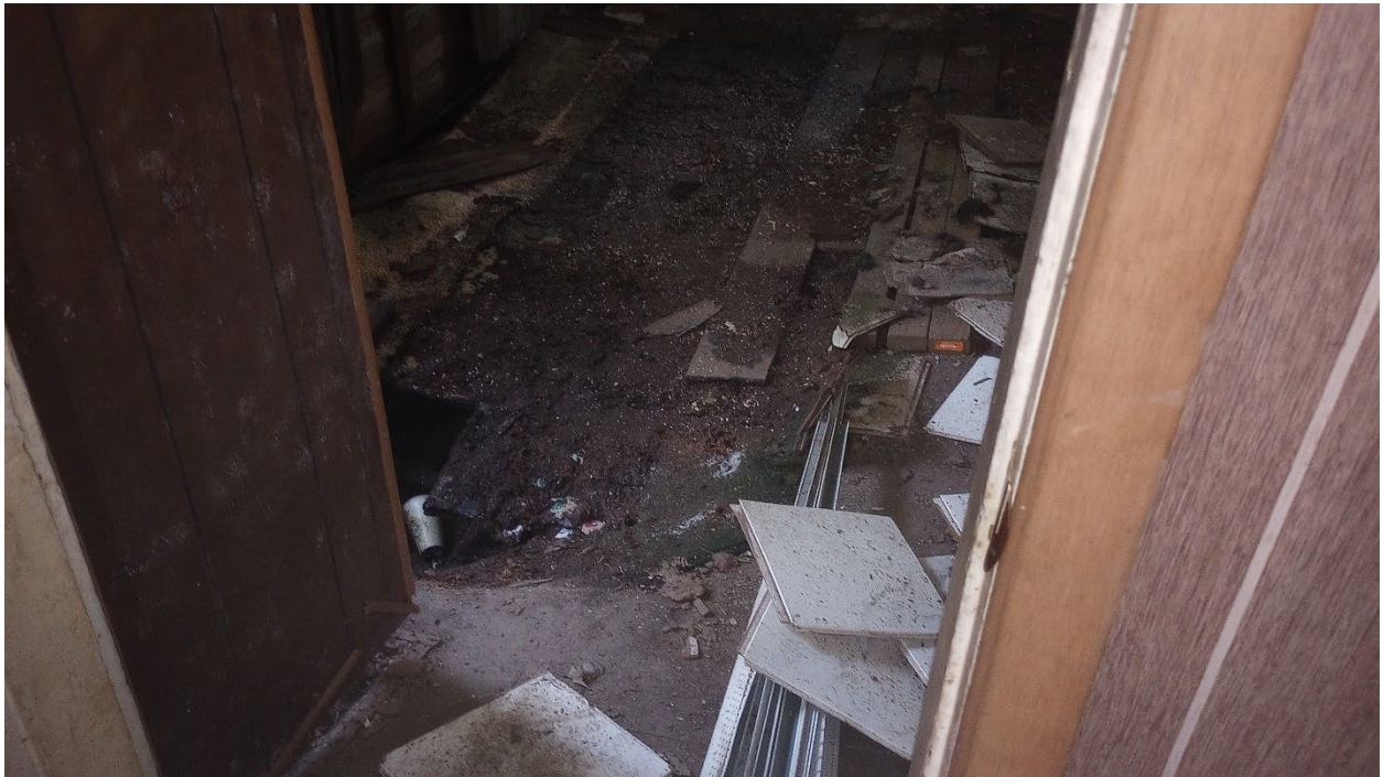
#6 Failed floor structure in Northeast room due to roof leaks
