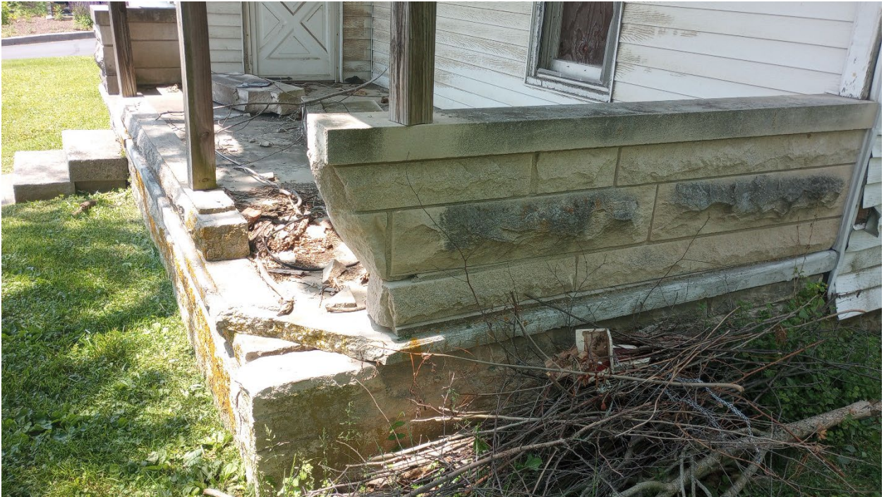
#1 Front porch wall damage
