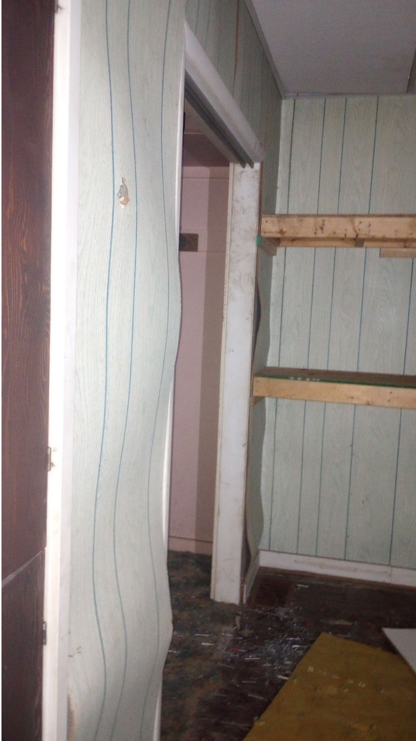
#11 Warped interior walls
