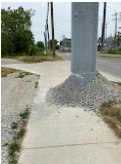
Pole at S Rogers - Warehouse.jpeg 153K
