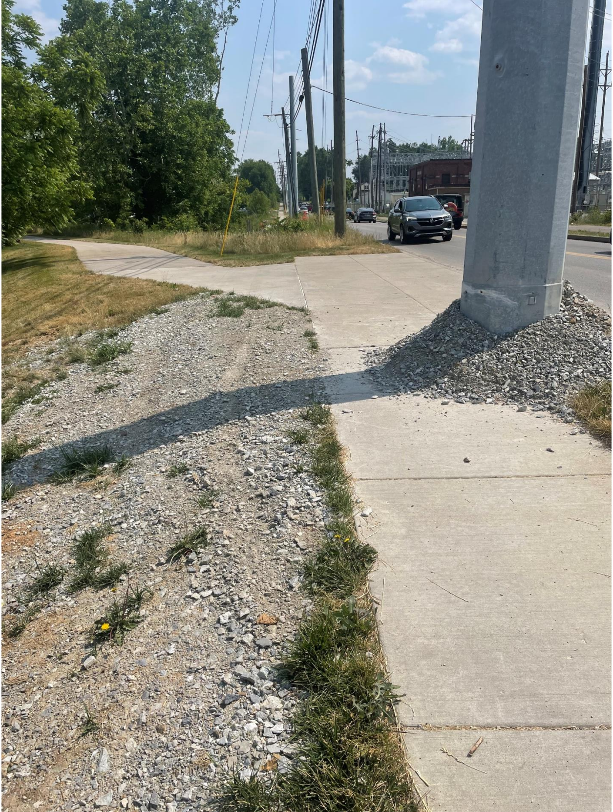
Photo 2 Obstruction at app. 1525 S Rogers St, facing south. June 8th, 2023.
