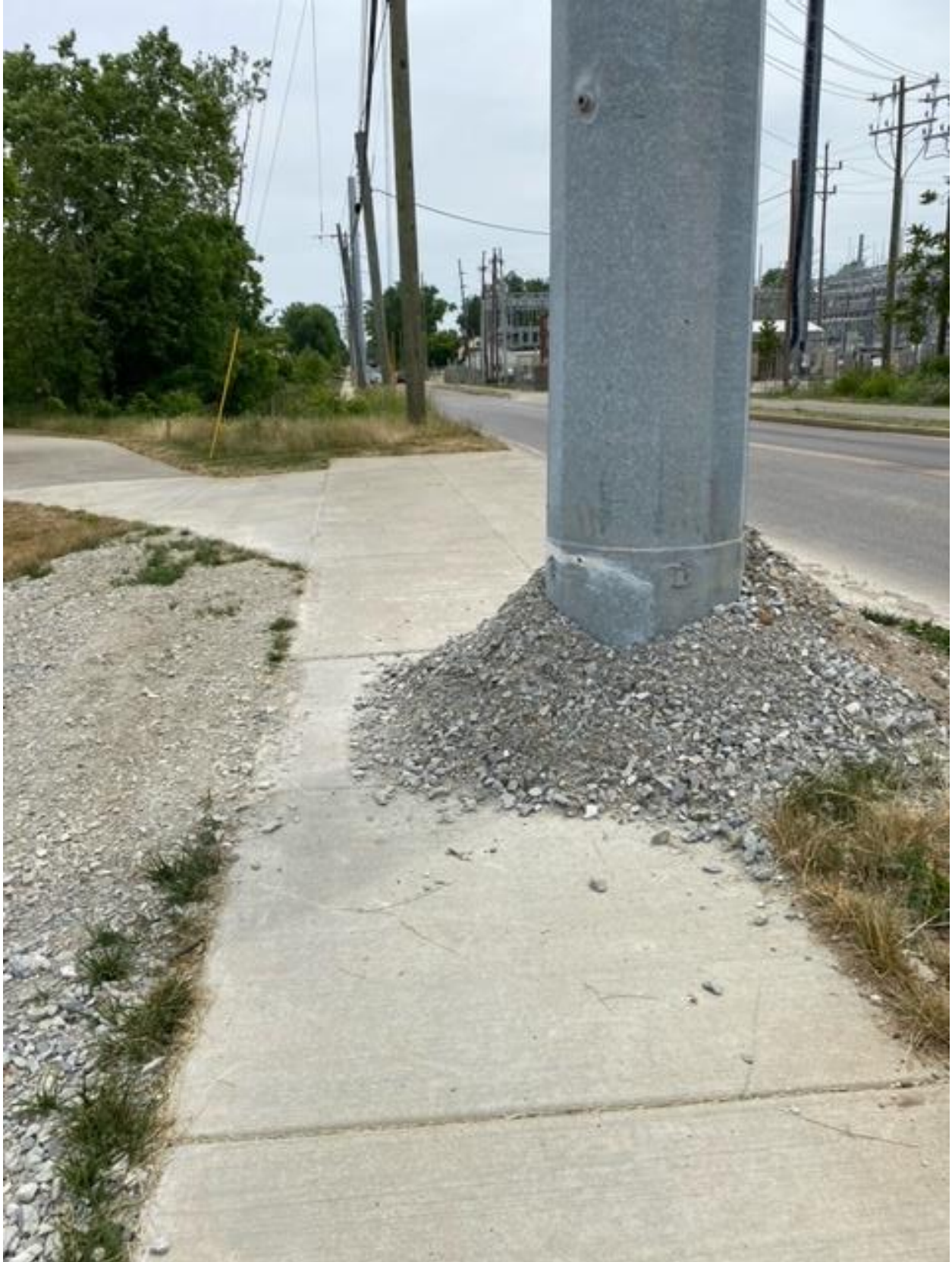
Photo 1 Obstruction at app. 1525 S Rogers St, facing south. June 7th, 2023.
