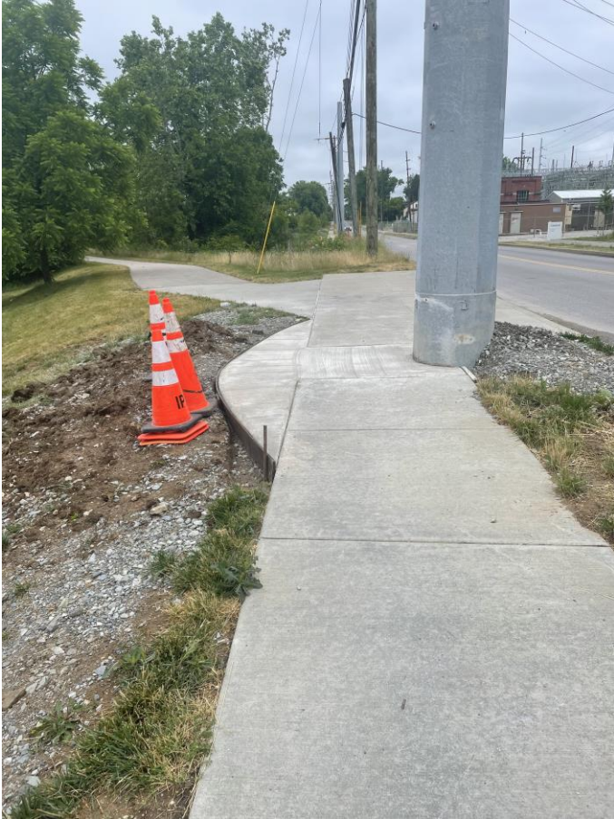
Photo 4: Current state of sidewalk 6/12/2023
