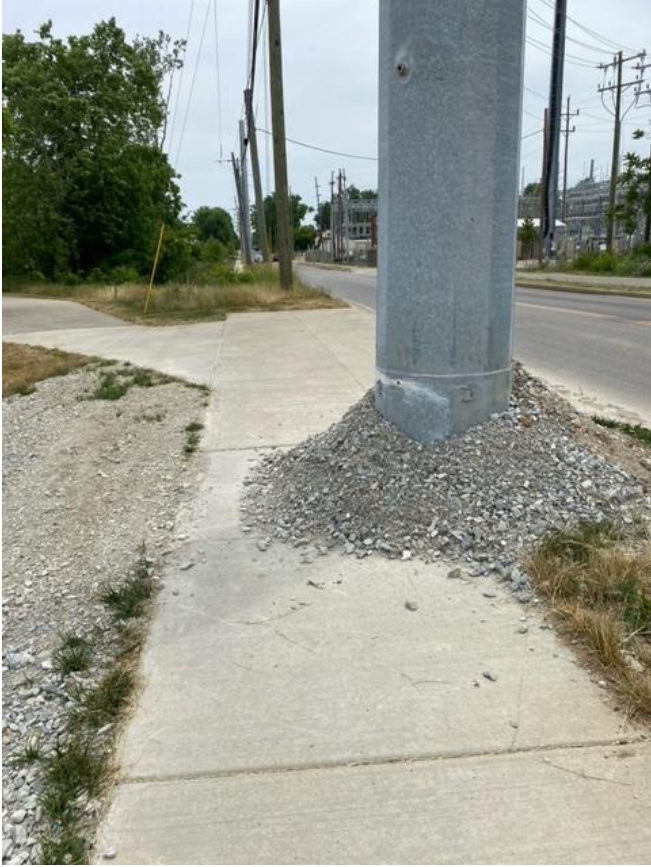
Photo 1: Gravel backfill blocking sidewalk 6/7/2023
