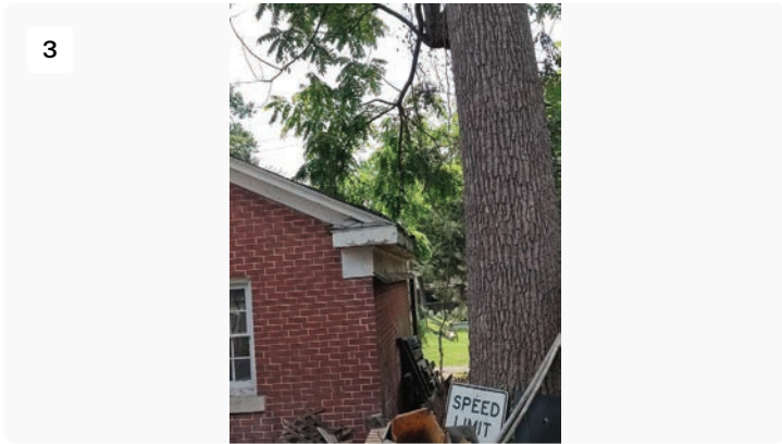
Branches resting on garage roof.
