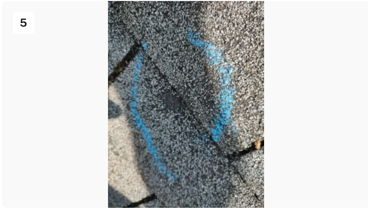
Damage from falling walnuts.
