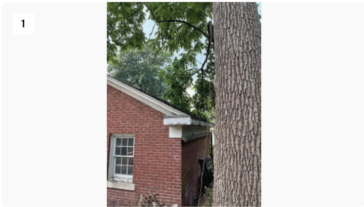
Walnut tree proximity to north easterly corner of detached garage.
