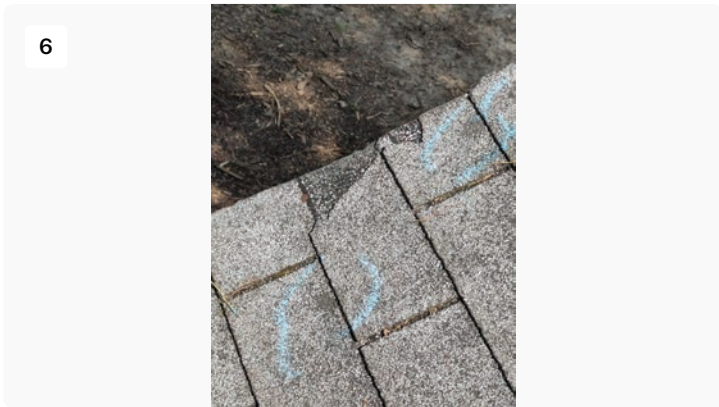
Broken shingles and falling walnut damages.
