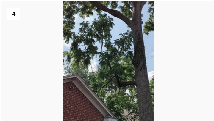
Large branch from tree causing all other branches that are resting on the roof.
