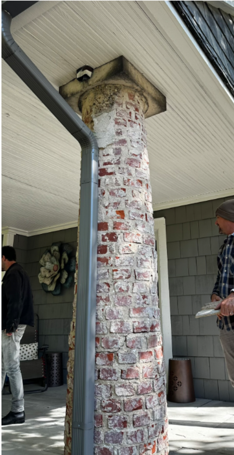
Southwest column with remaining pebble dash stucco on the side facing west.
