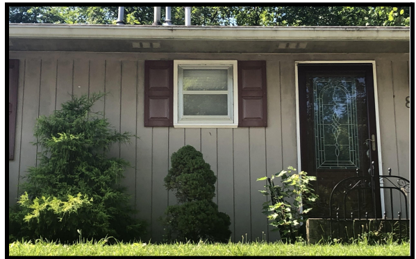
Not Recommended: Vertically-oriented siding.
