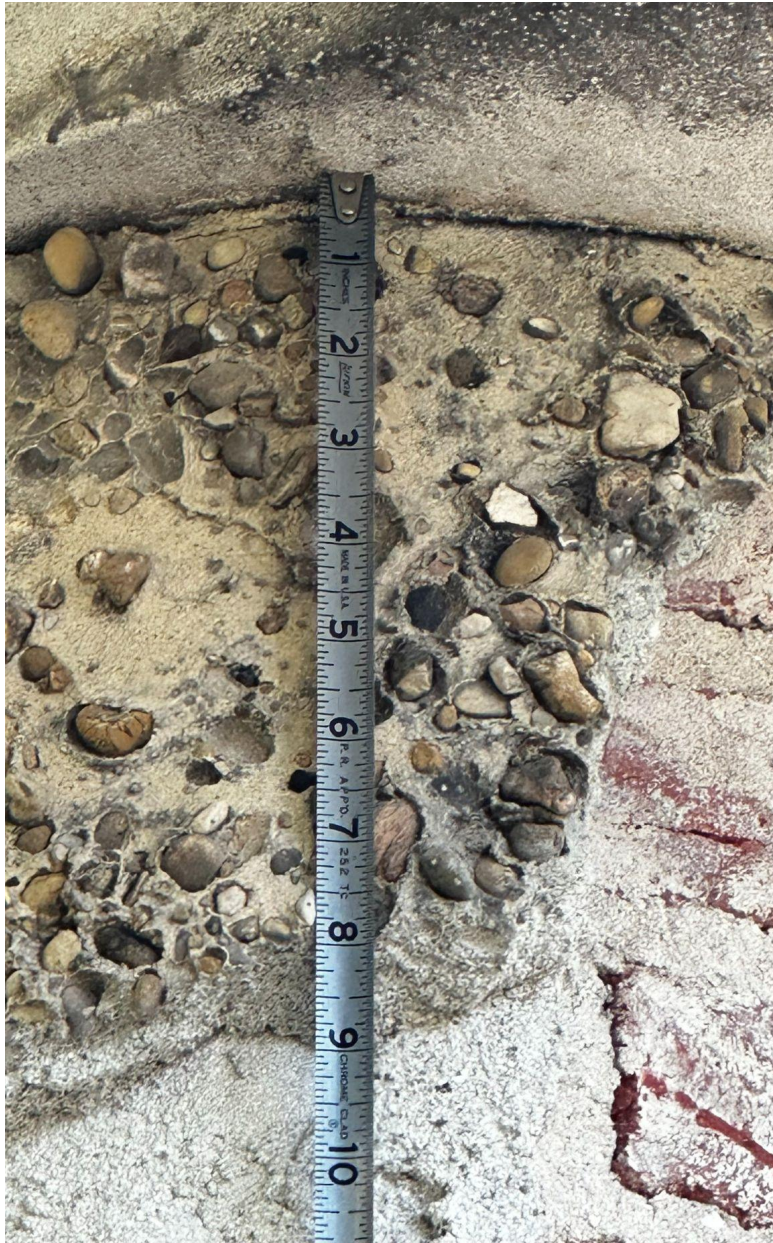
Detailed view of the Southwest column with remaining pebble dash stucco on the side facing west.
