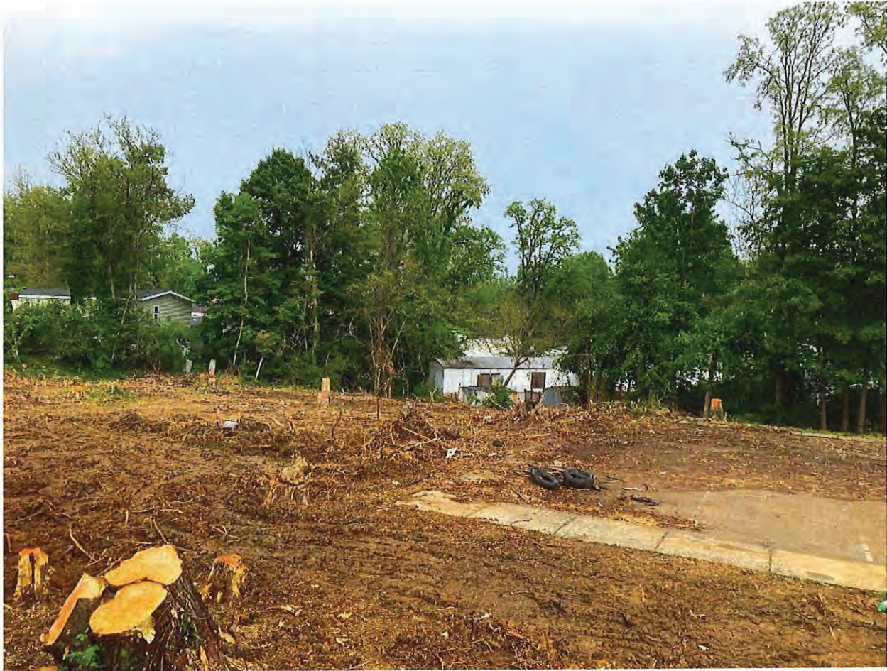
Photo 1: Earth disturbance, absence of erosion control measures, and trees removed on the northern side of 1450 N Willis Drive on 05/16/2023.
