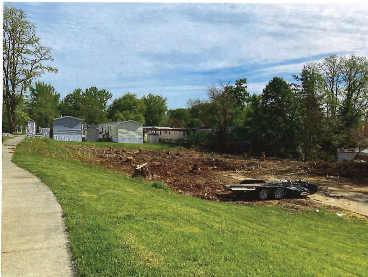
Photo 4: Earth disturbance, absence of erosion control measures, and trees removed on the northern side of 1450 N Willis Drive on 05/11/2023.
