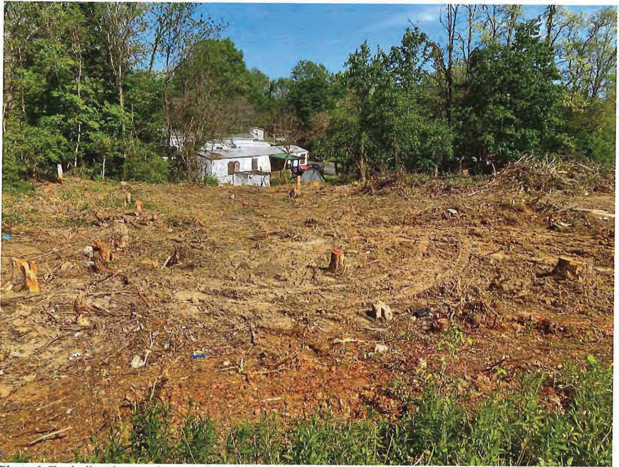
Photo 6: Earth disturbance, absence of erosion control measures, and trees removed on the northern side of 1450 N Willis Drive on 05/09/2023.
