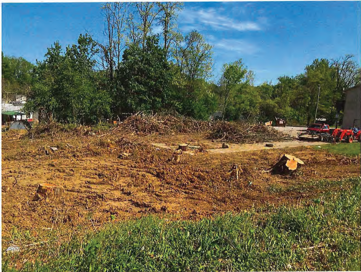
Photo 5: Earth disturbance, absence of erosion control measures, and trees removed on the northern side of 1450 N Willis Drive on 05/09/2023.
