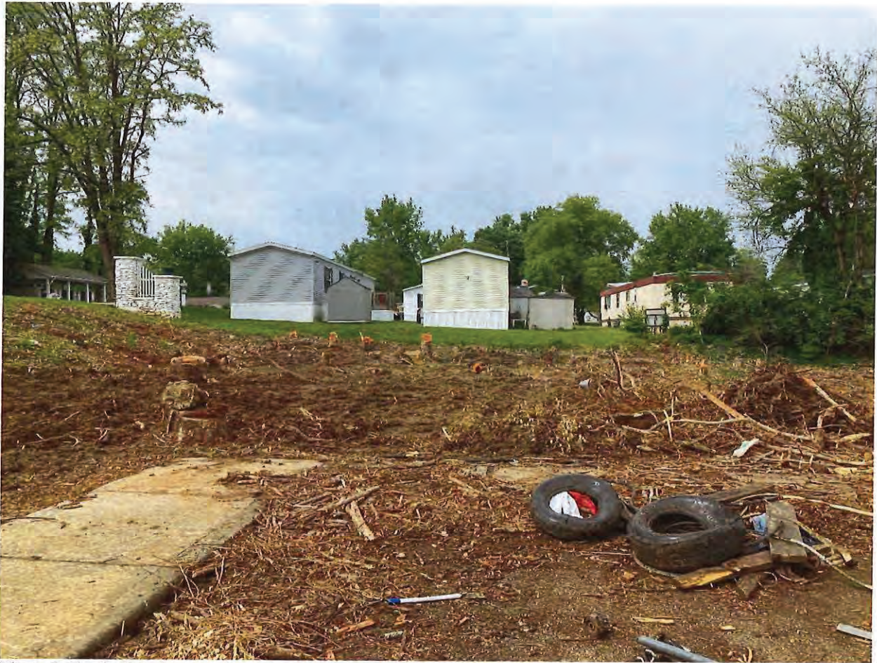
Photo 2: Earth disturbance, absence of erosion control measures, and trees removed on the northern side of 1450 N Willis Drive on 05/16/2023.
