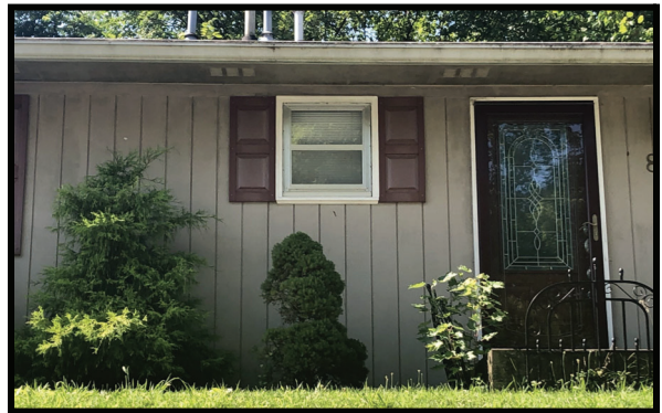
Not Recommended: Vertically-oriented siding.
