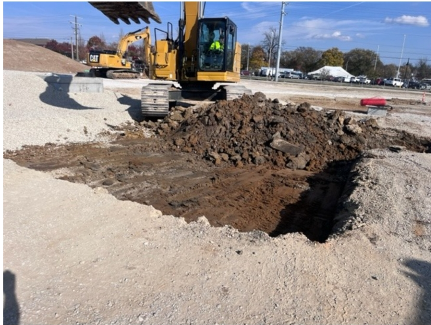
View of undercut location #3.
