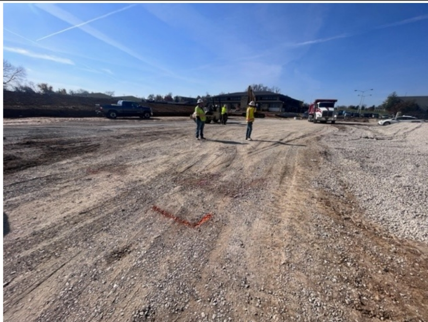
View of undercut location #3 after failing the proofroll.
