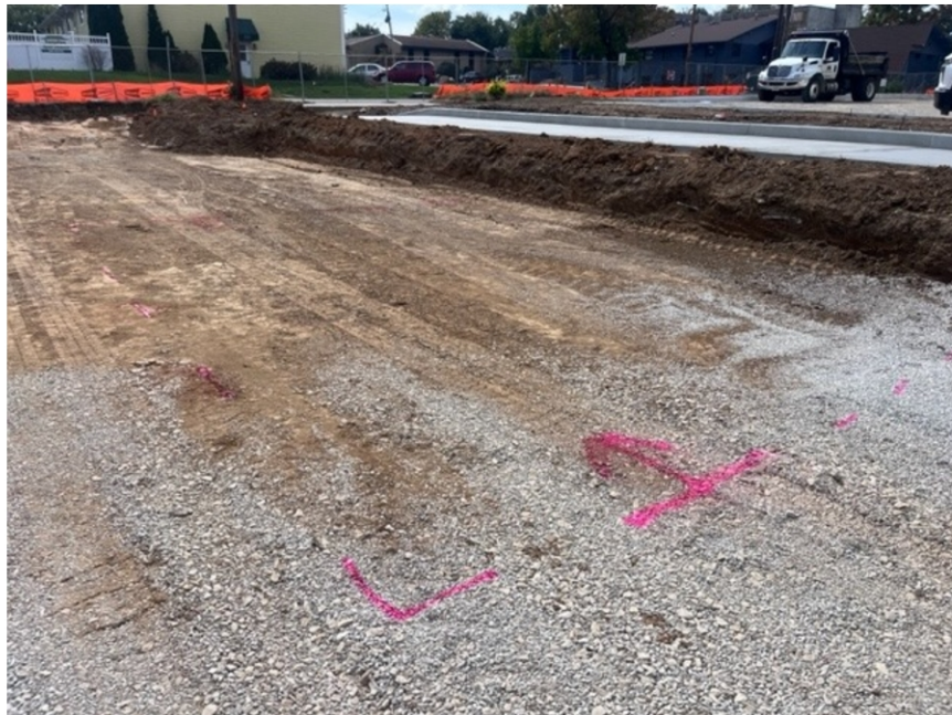
View of Failed location marked up at the Southern end of the proofrolling location.
