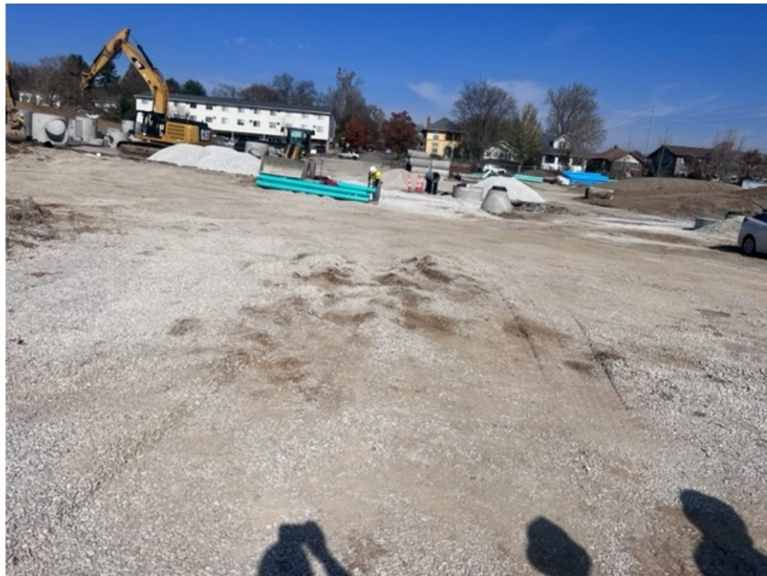
View of undercut location #2
