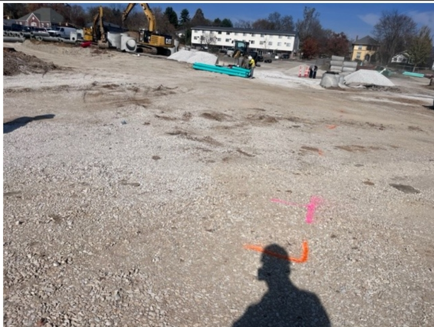
View of undercut location #2 after failing the proofroll.
