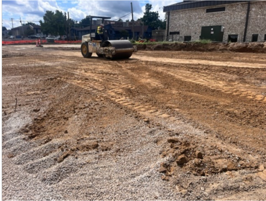
View of the site being prepped prior to proofrolling East of Centerstone.
