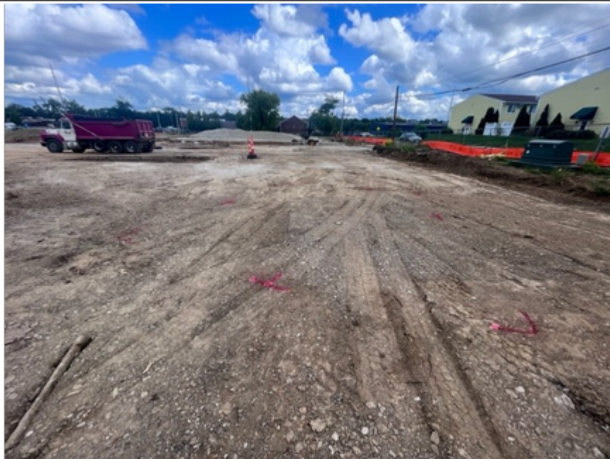
View of failed location near the Southern entrance of Centerstone.
