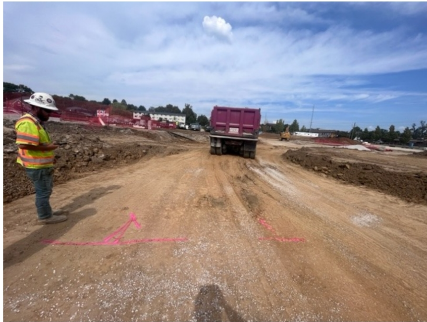
View of Failed location marked up at the Northern end of the proofrolling location.
