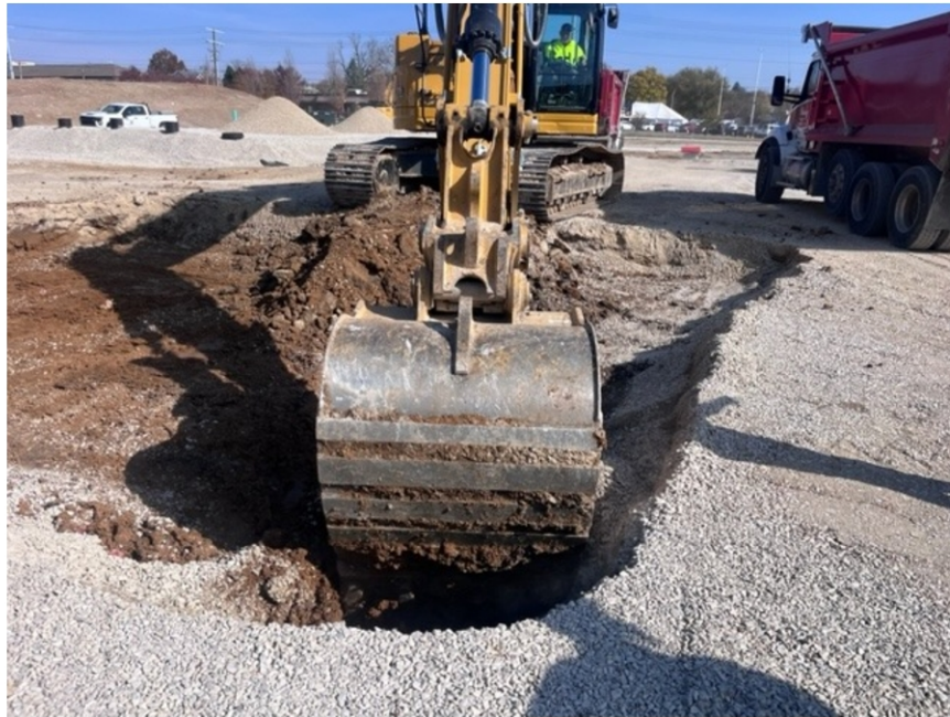
View of unsuitable soils for undercut location #2.
