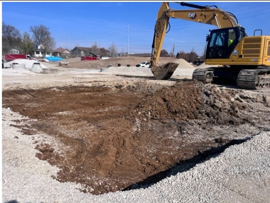
View of unsuitable soils for undercut location #2.
