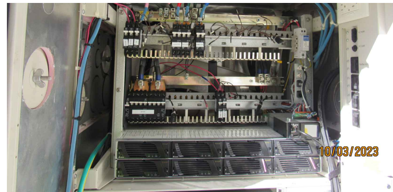
EXISTING DC BREAKER SHELF PHOTO
