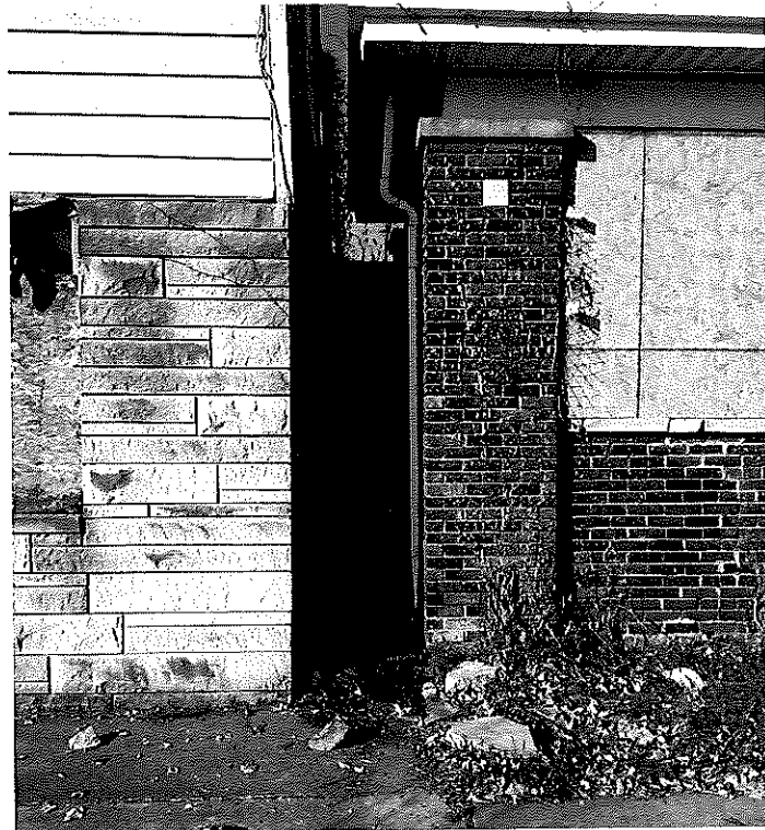
Gap between structures
