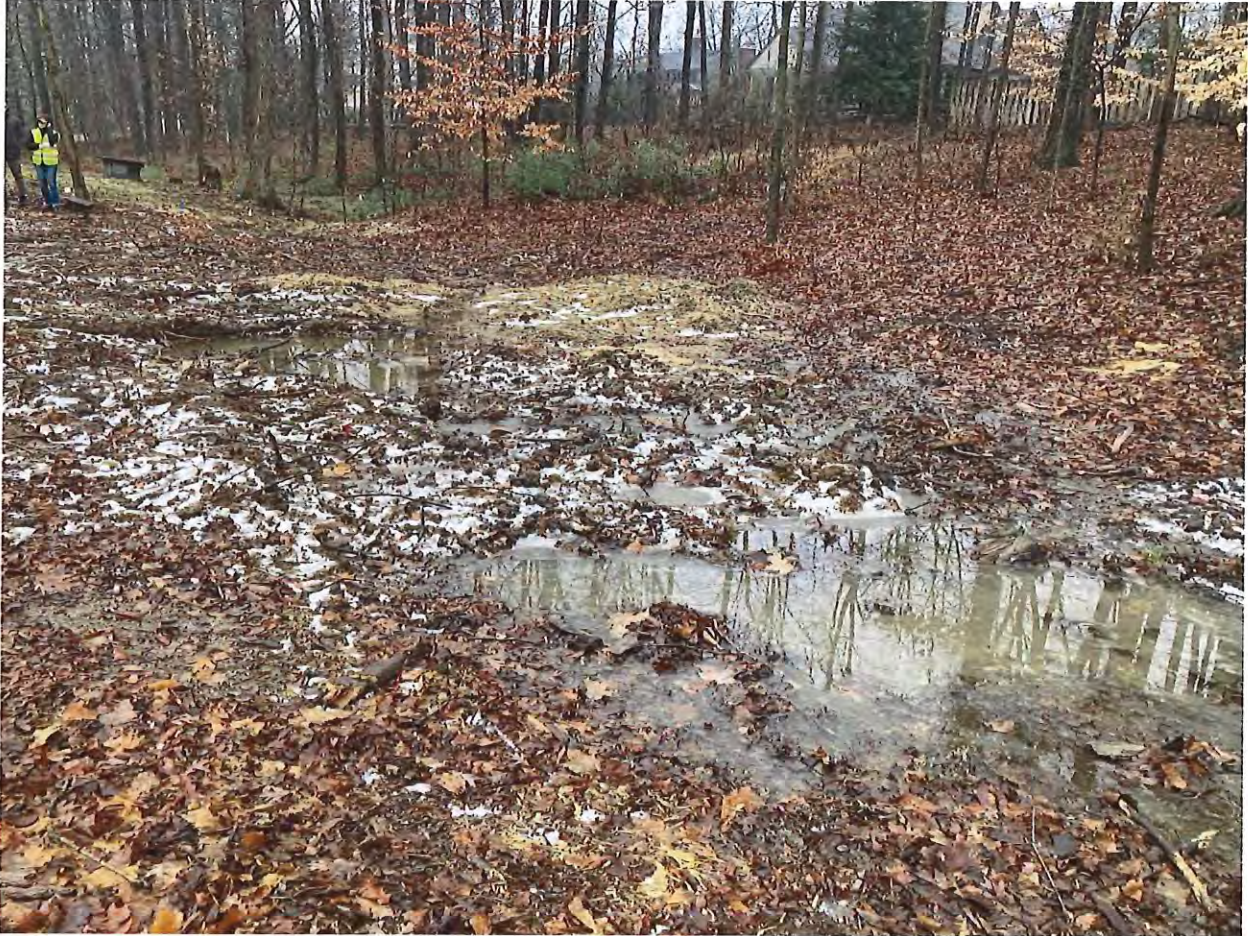
Photo 7: Intermittent stream, earth disturbance, absence of erosion control measures, and trees and vegetation removed near the intermittent stream (south-central area of the lot) at 2214 E Maxwell Lane on 01/23/2024, facing east.
