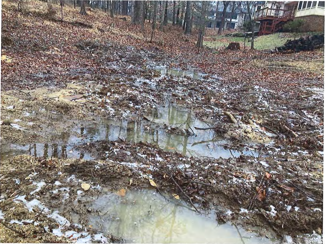
Photo 5: Intermittent stream, earth disturbance, absence of erosion control measures, and trees and vegetation removed near the intermittent stream (south-central area of the lot) at 2214 E Maxwell Lane on 01/23/2024, facing west.
