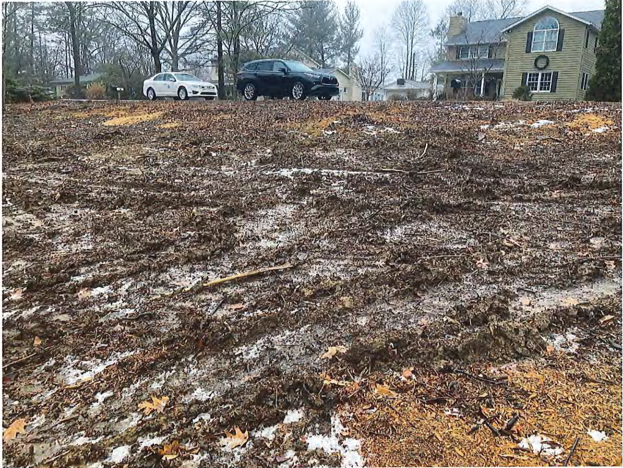
Photo 4: Earth disturbance, absence of erosion control measures, and trees removed on the northern side at 2214 E Maxwell Lane on 01/23/2024 from central portion of site, facing north.
