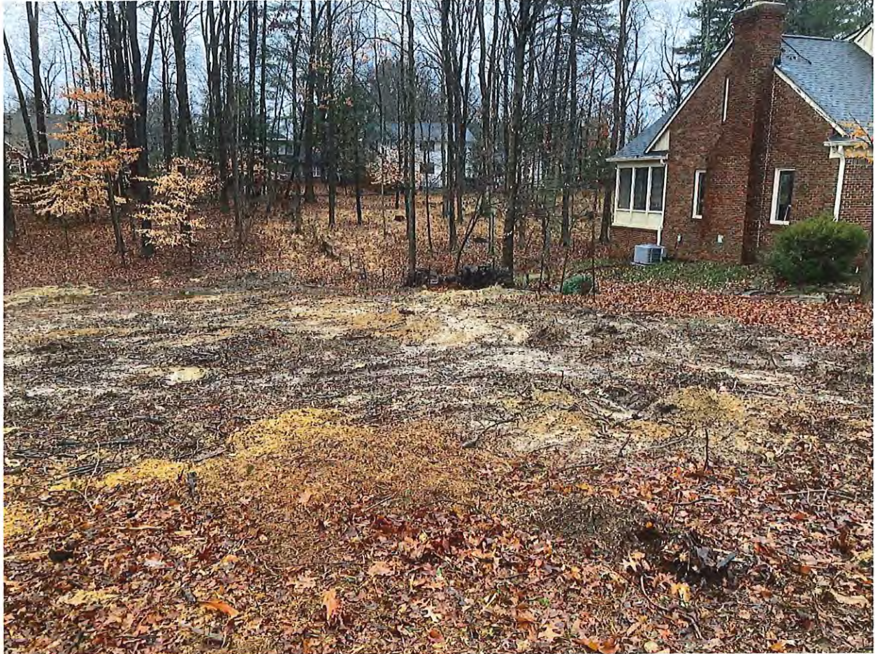
Photo 2: Earth disturbance, absence of erosion control measures, and trees removed on the northwestern side of 2214 E Maxwell Lane on 01/09/2024.
