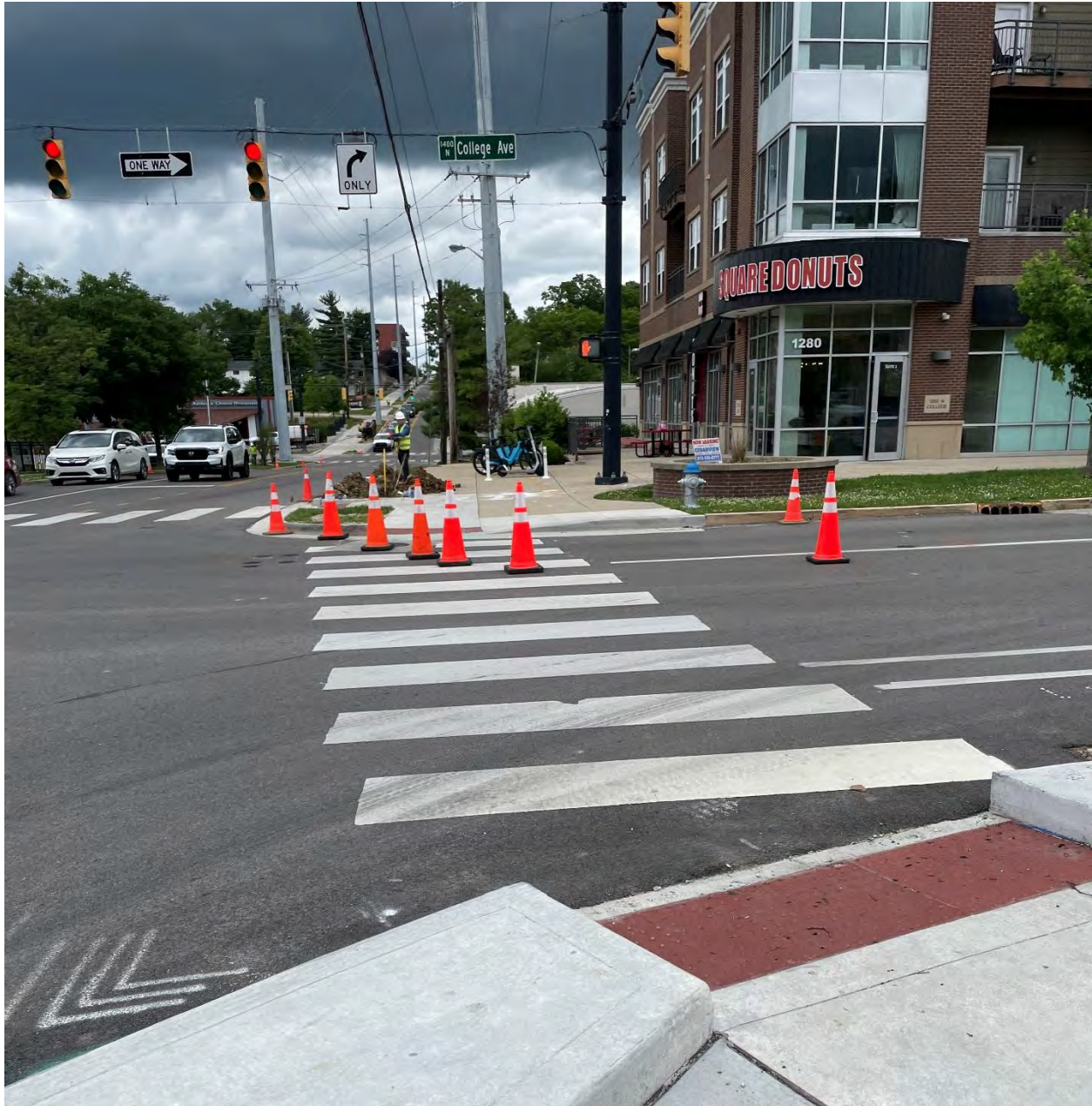
Photo 8: Crosswalk blocked by lane closure on N College Ave. Sidewalk beyond lane closure is also blocked by dirt, but does not have signage as required. (5/29/2024)
