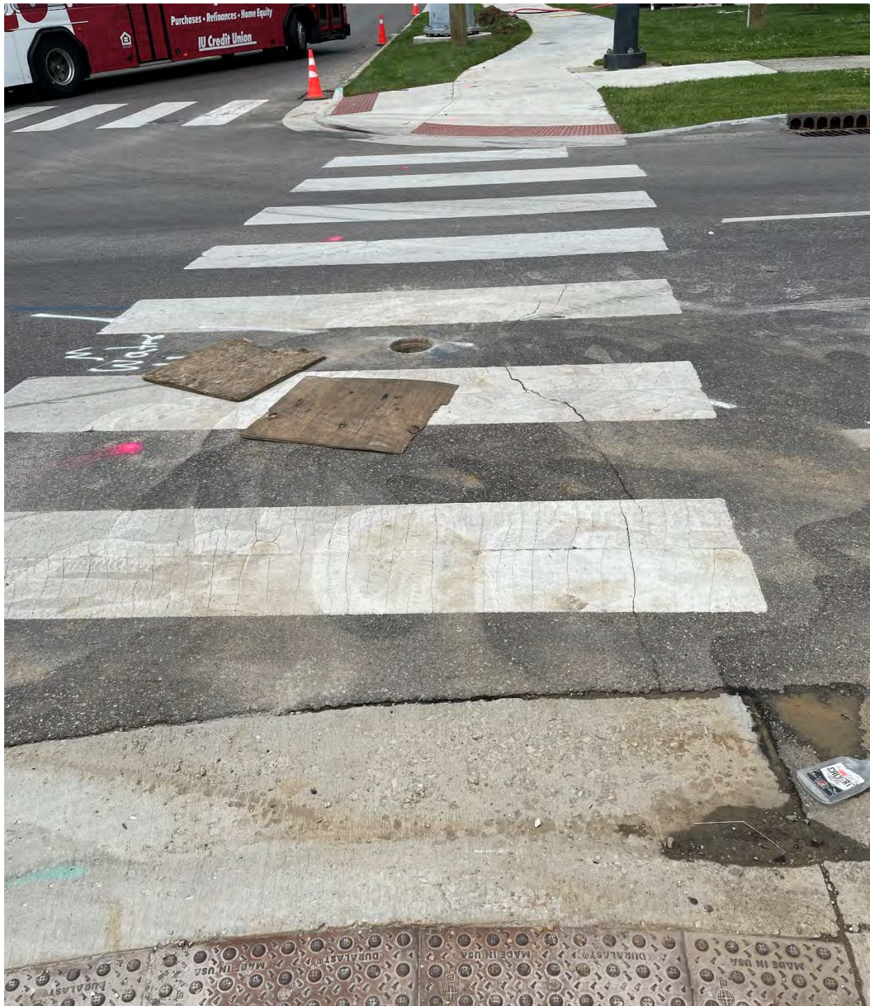
Photo 9: Open core holes within the crosswalk that is open to pedestrian traffic. (5/29/2024)
