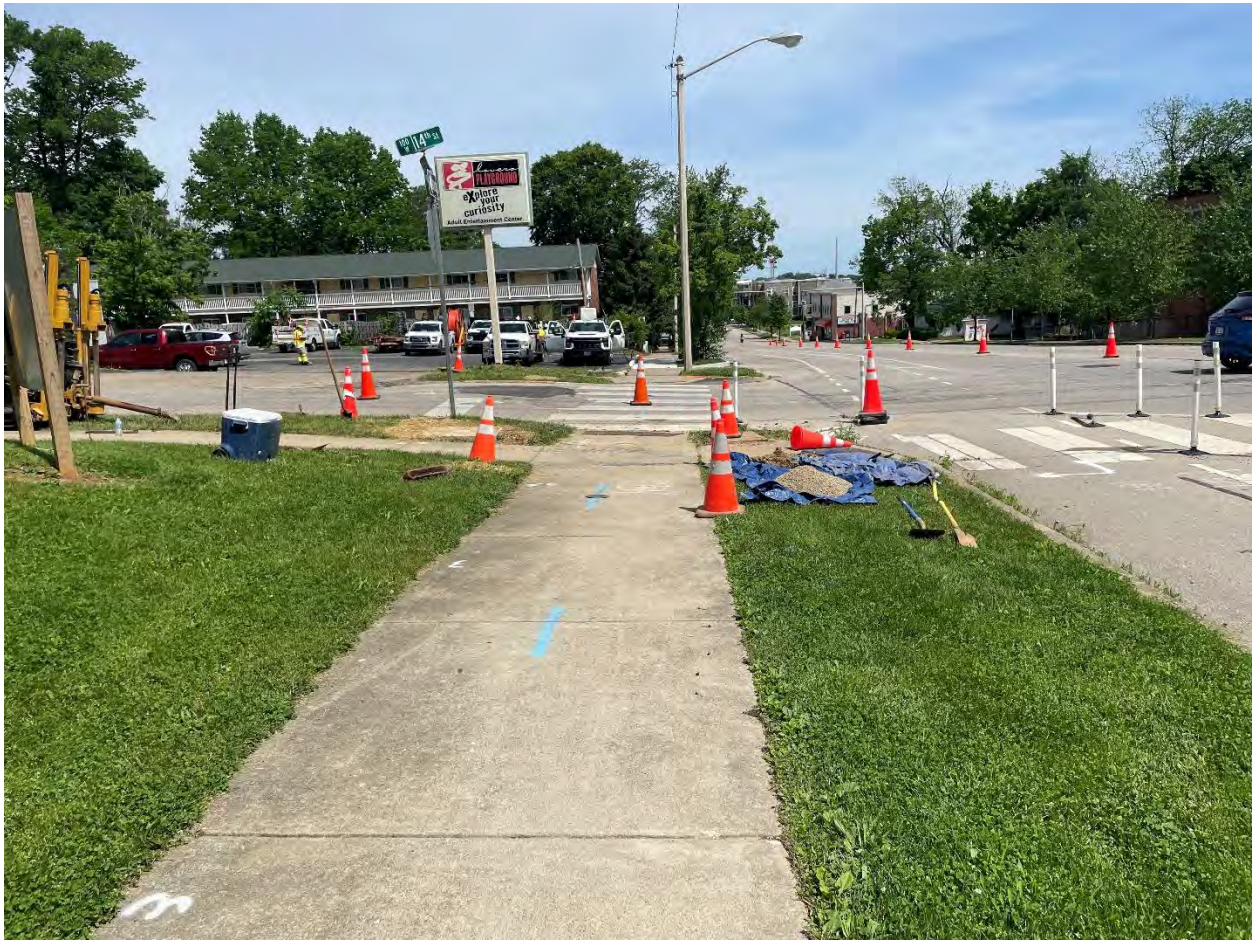
Photo 3: Unclear the intended traffic control that is required to be in place at the site. The traffic control in place is blocking the pedestrian cross walk. (5/8/2024)
