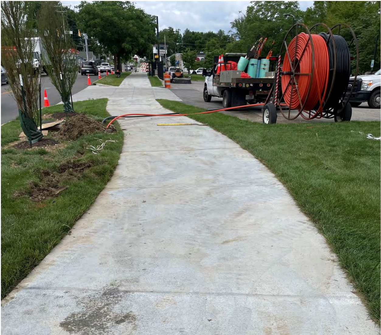
Photo 10: Sidewalk blocked by conduit that is being pulled through the ground. Traffic control is only in place at one side of the closure. (5/29/2024)
