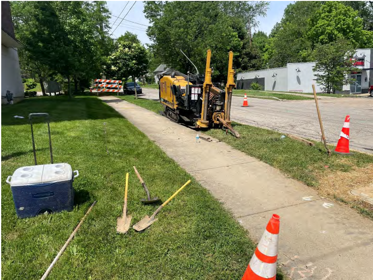
Photo 4: Sidewalk is blocked by barricades in the wrong location if it is intended to prevent pedestrians from encountering the work equipment. (5/8/2024)
