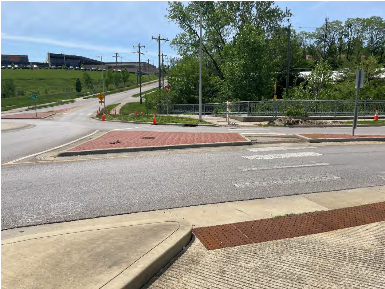
Photo 5: Improper sidewalk closure for work at the roundabout of W Arlington Rd, W 17 th St, and N Monroe St. The barricade is blocking the crosswalk preventing pedestrians to detour around the closure. (5/8/2024)
