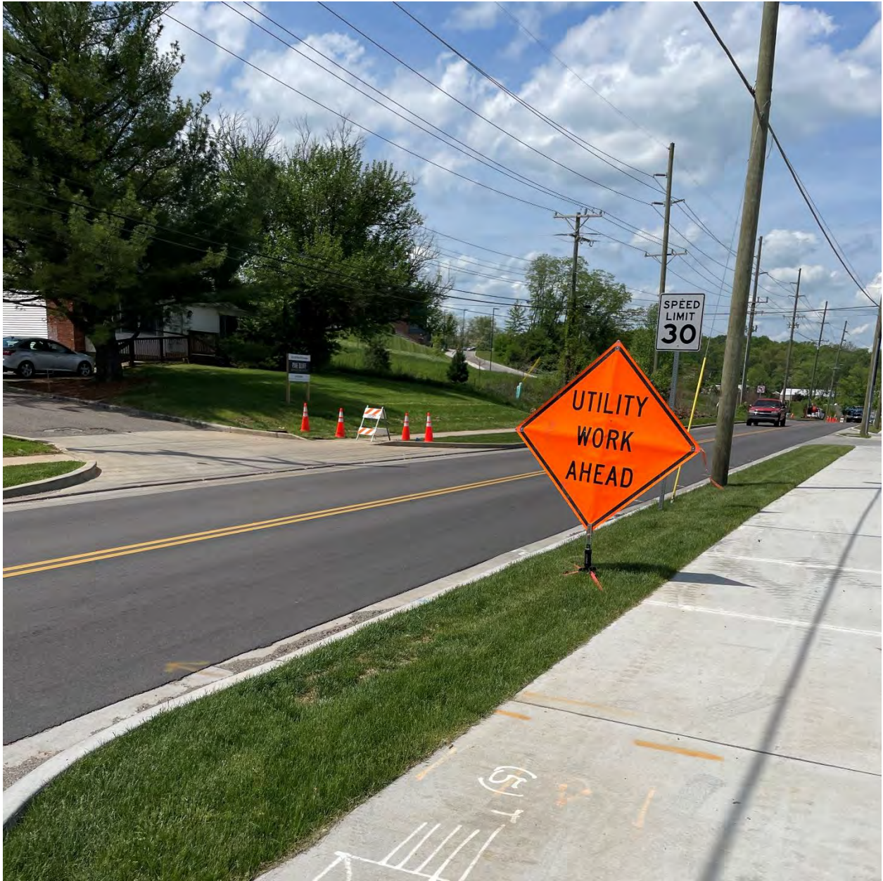
Photo 1: Improper sidewalk closure between N Maple St and N Monroe St (5/2/2024)
