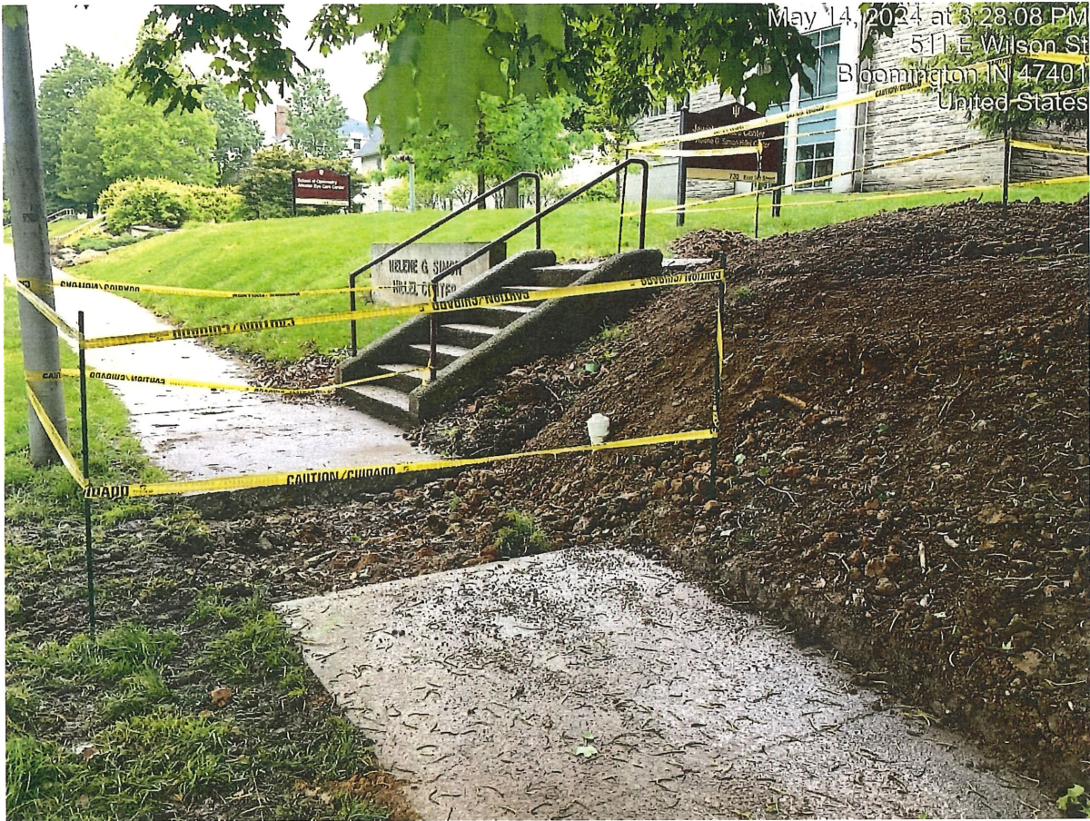
Photo 1: Sidewalk in front of 703 E 3 rd St that has been removed after recent sanitary sewer repairs and is only protected from pedestrians via caution tape (5/14/2024)
