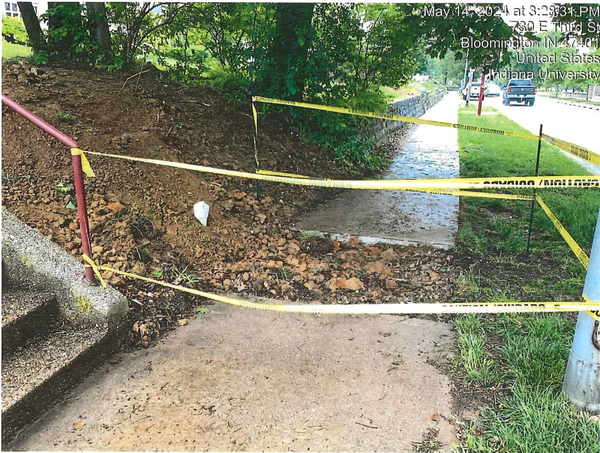
Photo 2: Opposite view of the sidewalk in front of 703 E 3 rd St that has been removed after recent sanitary sewer repairs and is only protected from pedestrians via caution tape (5/14/2024)
