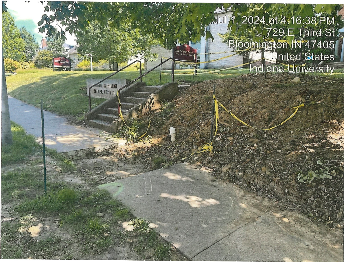
Photo 3: Sidewalk in front of 703 E 3 rd St with the caution tape fallen and no barricades having been put in place (7/1/2024)
