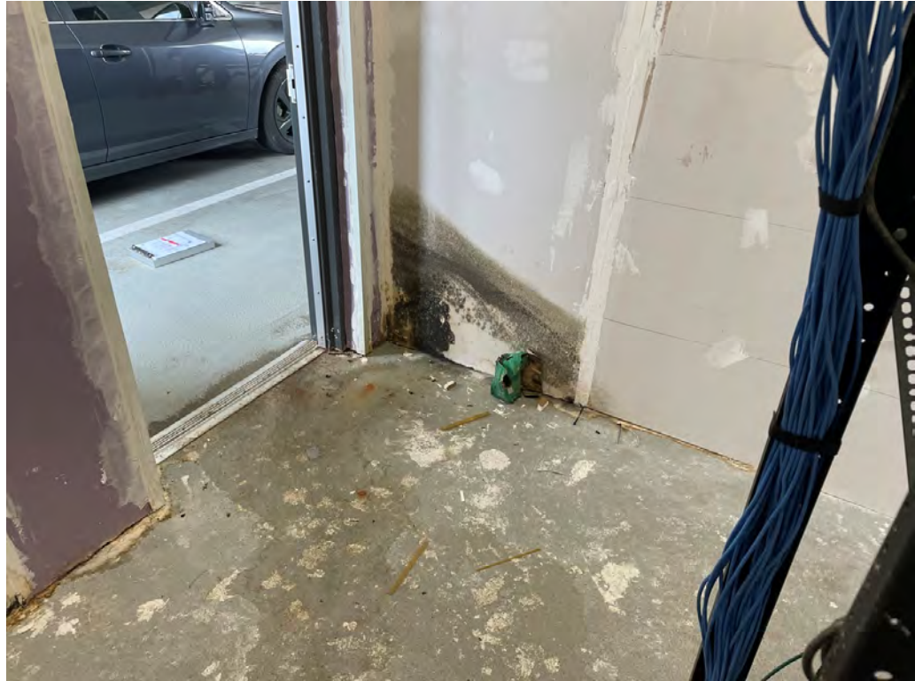
Photo 01: Evidence of water infiltration into IT room and mold on drywall
