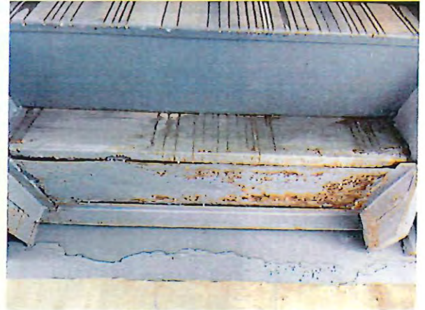
18 - stair steel corrosion.JPG
