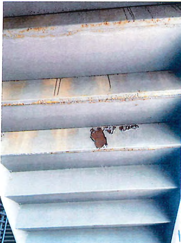
19 - stair steel corrosion.JPG
