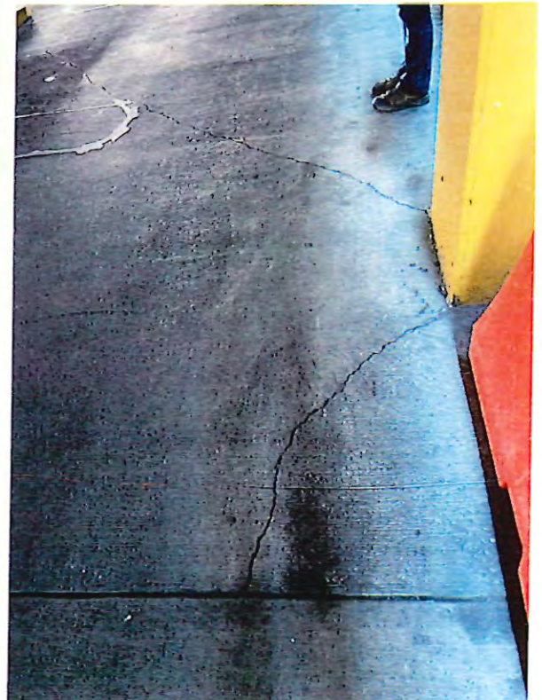
12 - SOG parking deck cracks.JPG
