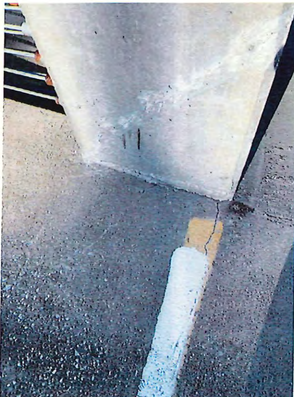
11 - elevated parking deck crack.JPG
