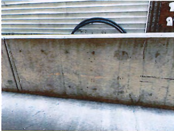
5 - tier 1 - exterior wall cracks.JPG
