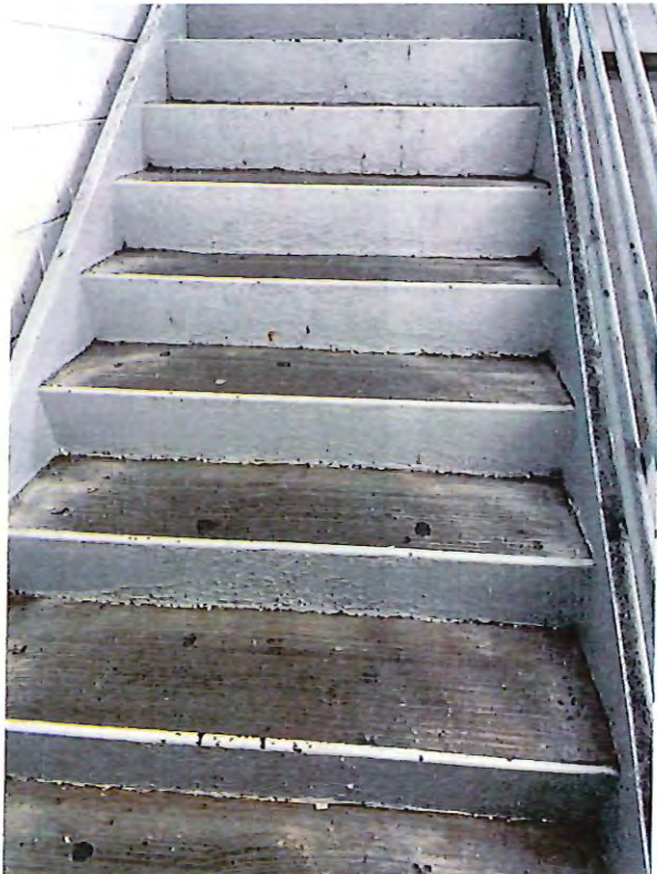
27 - west stair steel corrosion.JPG
