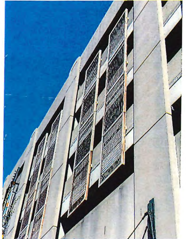
34 - facade panel corrosion.JPG
