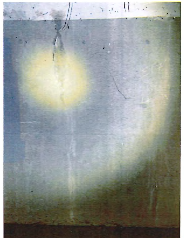
8 - basement level - wall crack.JPG
