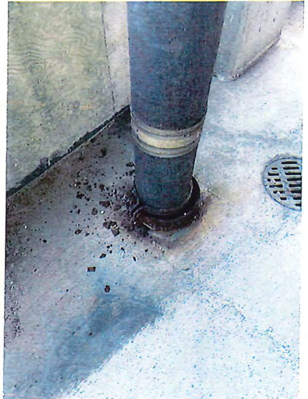
28 - corroded drain pipe sleeve.JPG
