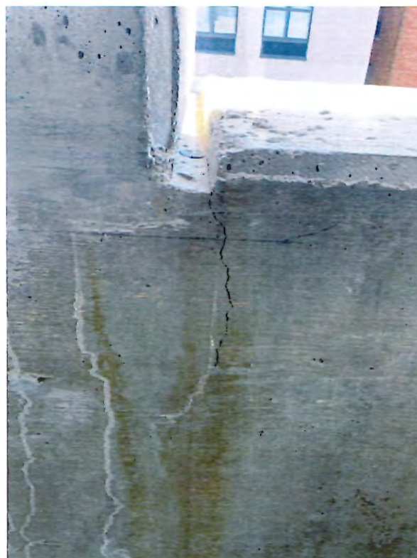
7 - exterior wall cracks.JPG
