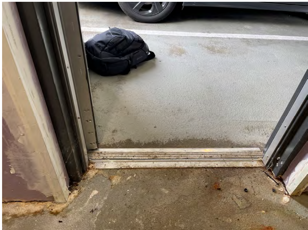
Photo 02: Debris at IT room door threshold
