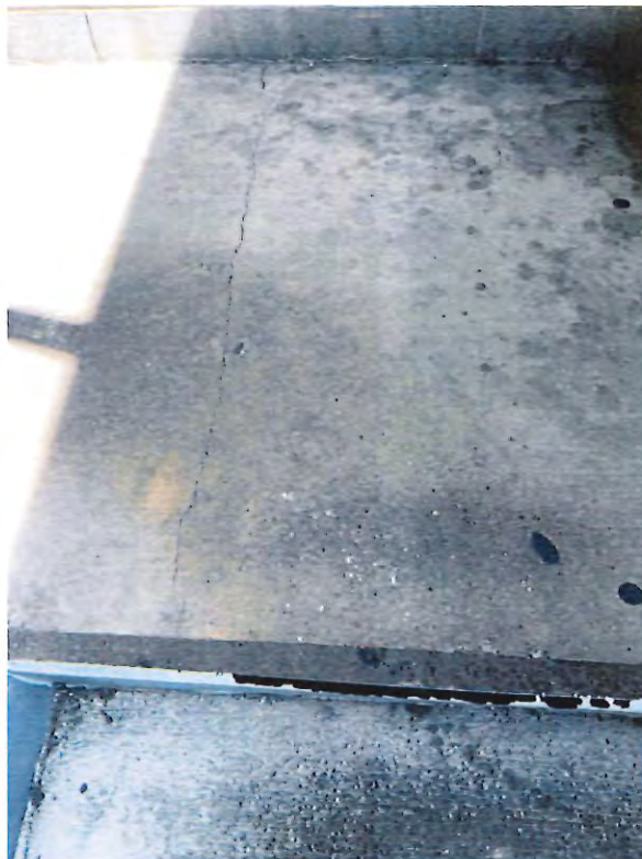
15 - crack in stair landing.JPG
