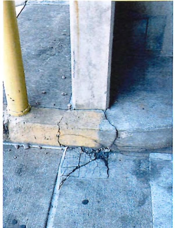
14 - spalled concrete curb.JPG
