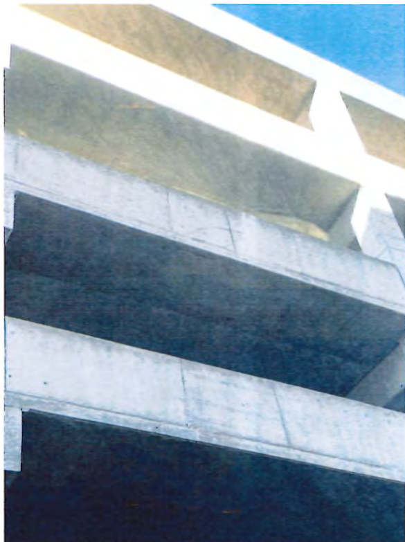
7 - tier 4 - exterior wall crack.JPG
