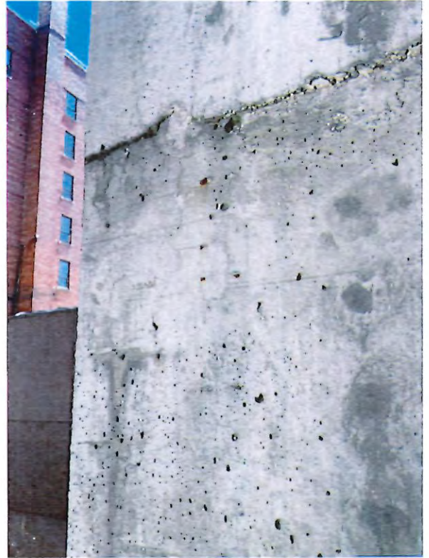
6 - column cracks with delamination.JPG
