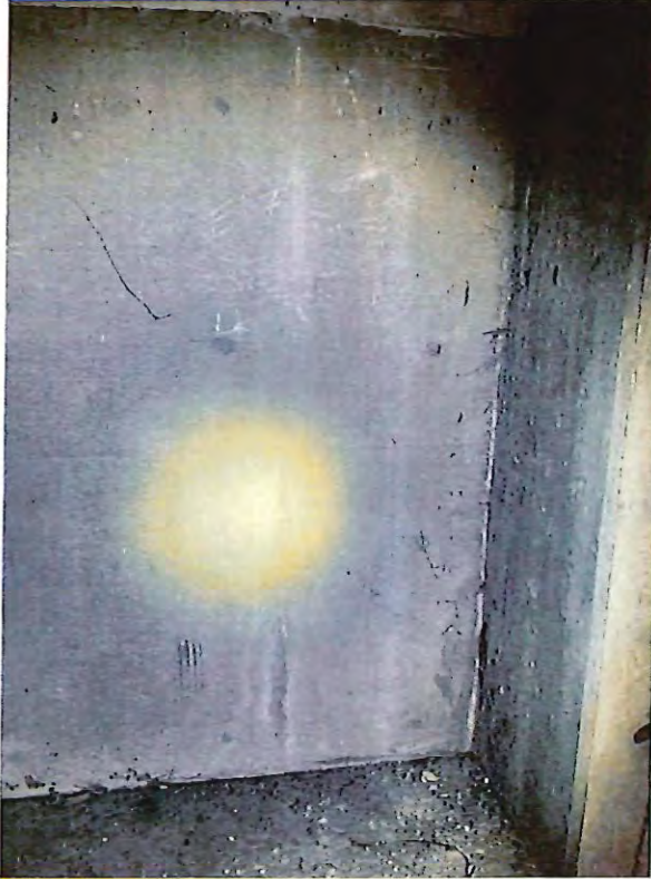
9 - basement level - wall crack.JPG
