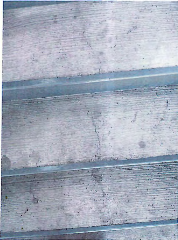
17 - crack in stair tread.JPG
