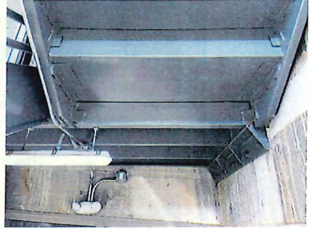
26 - east stair steel corrosion.JPG
