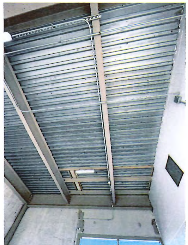
24 - stair tower steel corrosion.JPG
