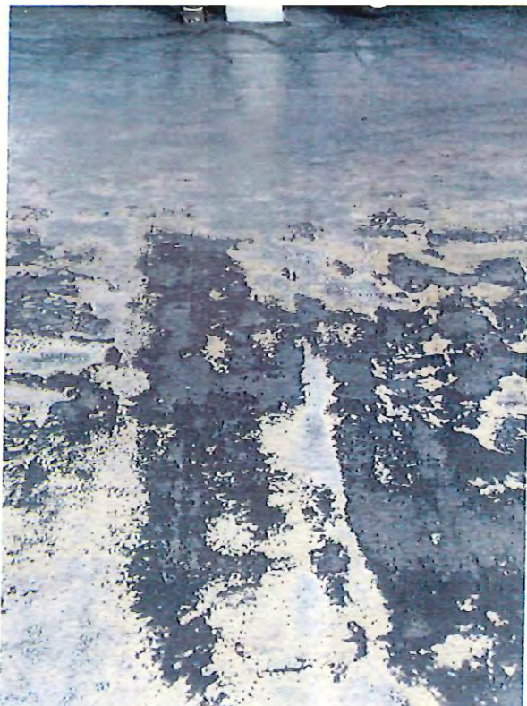
19 - traffic coating wear.JPG
