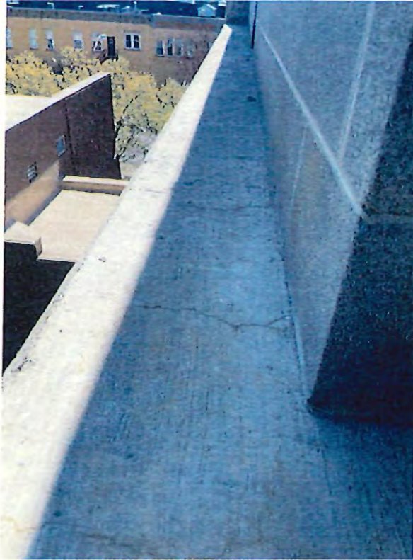
9 - exterior wall cracks.JPG
