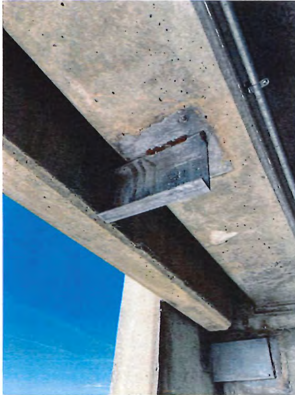
21 - corroded wall panel connection.JPG
