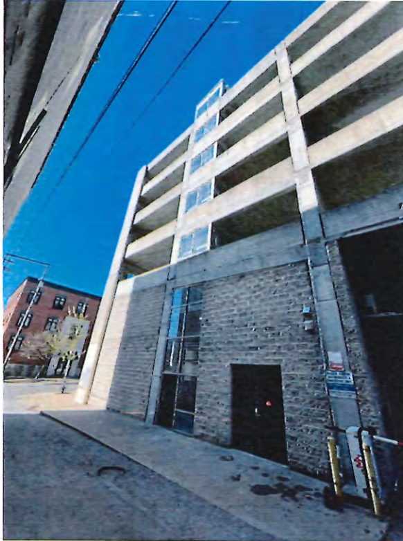
13 - PT pocket deterioration.JPG
