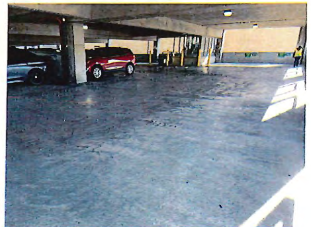
20 - traffic coating wear.JPG
