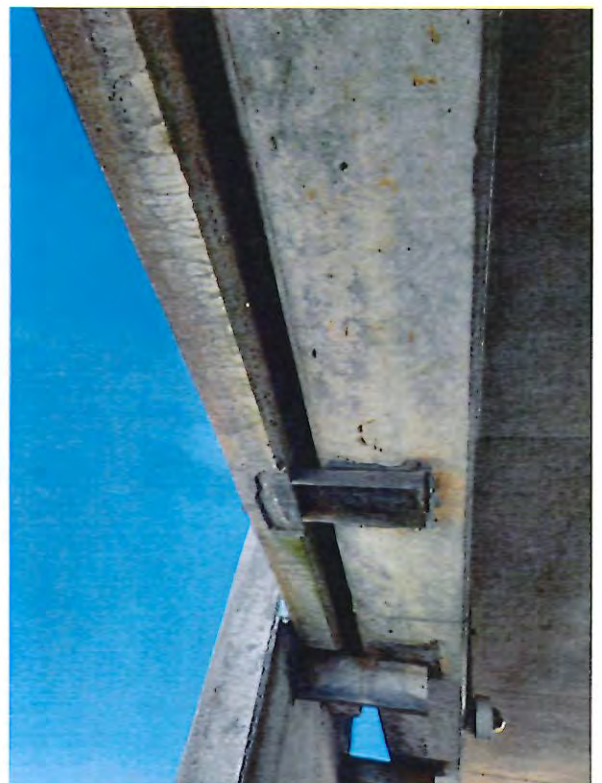
16 - spalled concrete at embed.JPG
