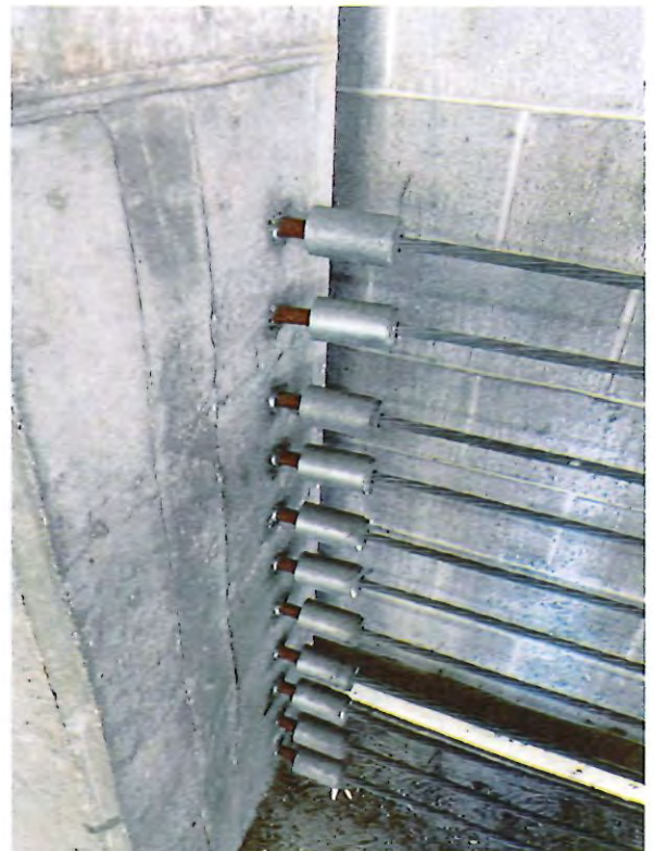
16 - corroded vehicular barrier cabling connection.JPG
