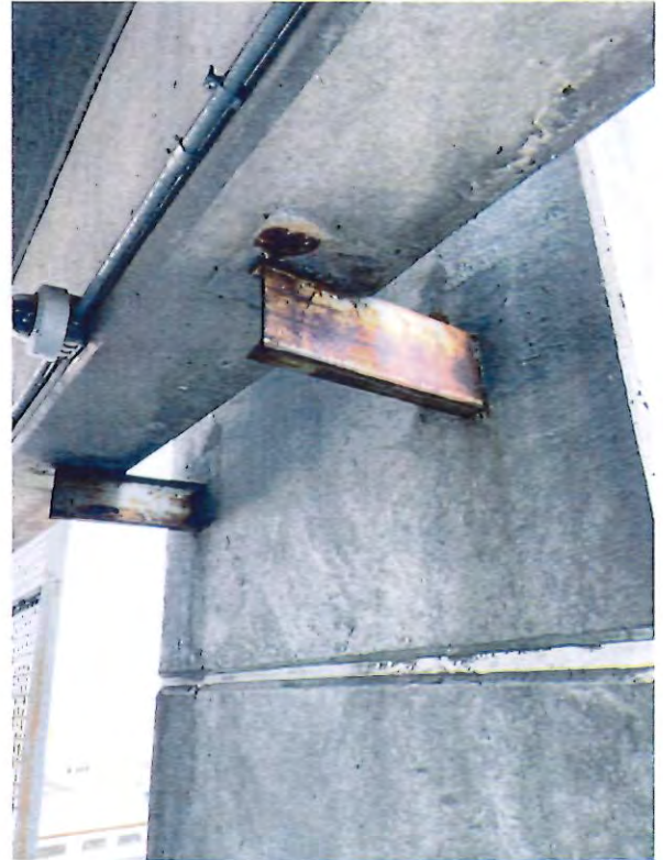
22 - corroded wall panel connection.JPG
