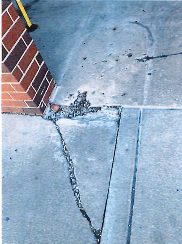
13 - SOG spalled concrete.JPG
