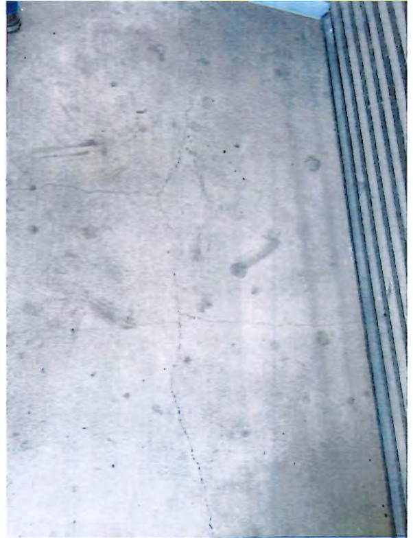
14 - crack in stair landing.JPG
