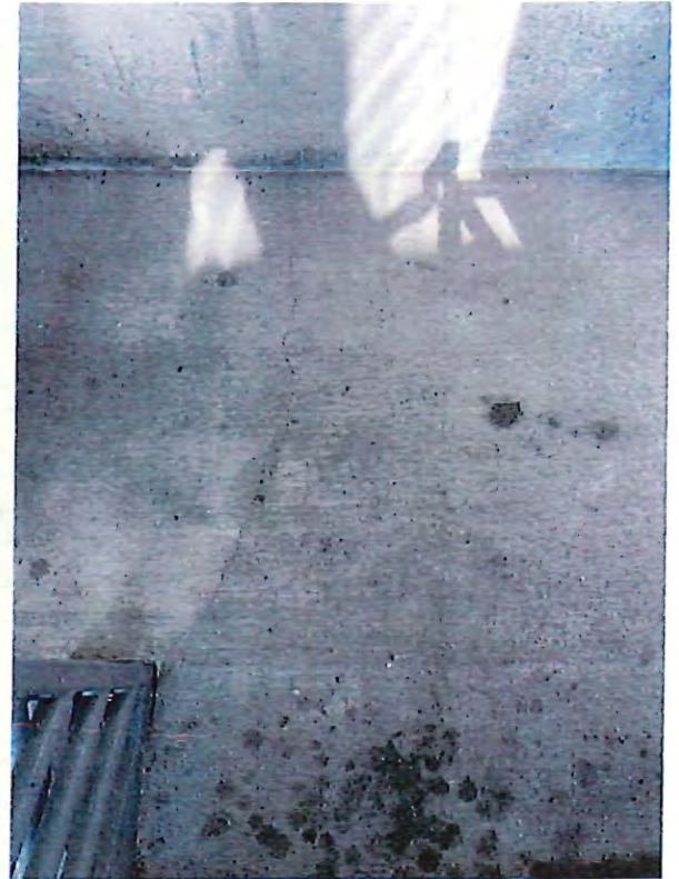
18 - crack in stair landing.JPG
