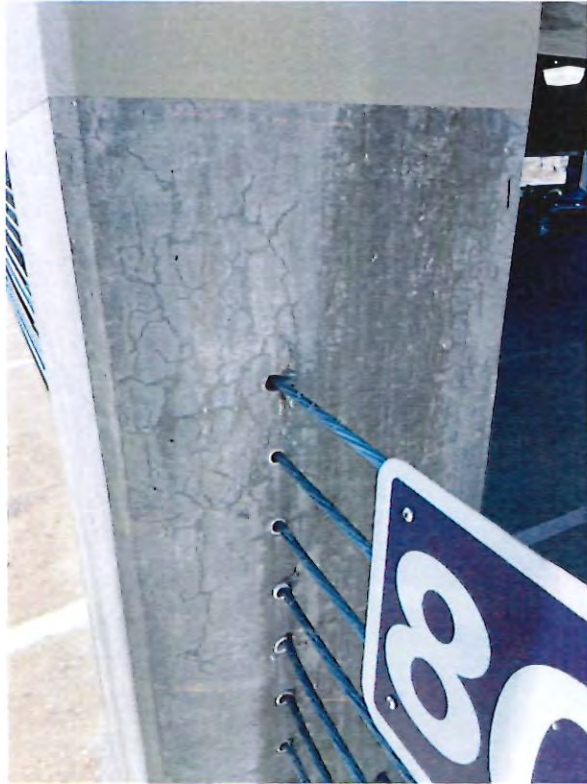
5 - column cracks with delamination.JPG
