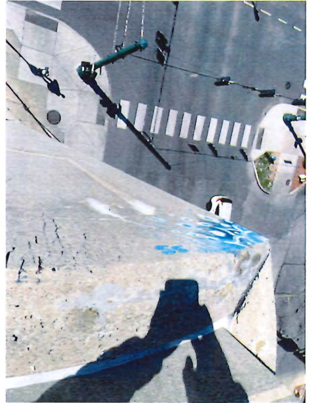
6 - tier 6 exterior wall crack.JPG
