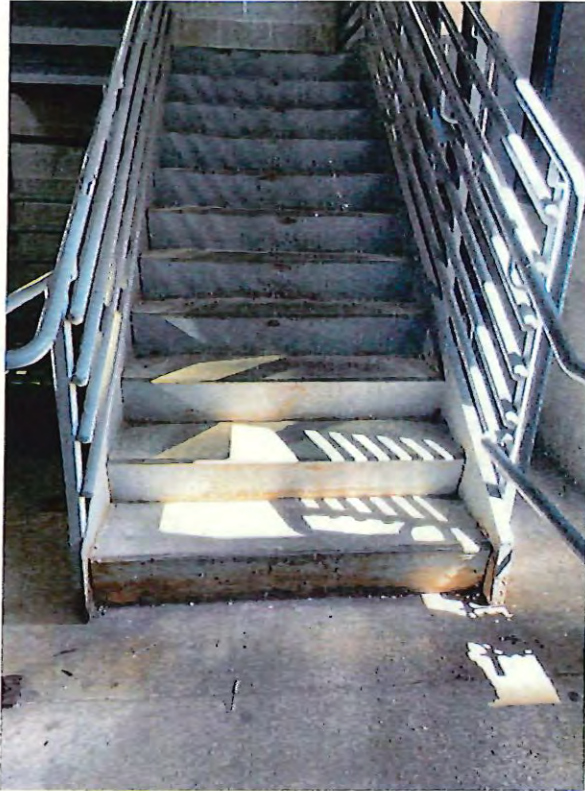
17 - stair steel corrosion.JPG
