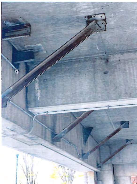
23 - corroded wall panel connection.JPG
