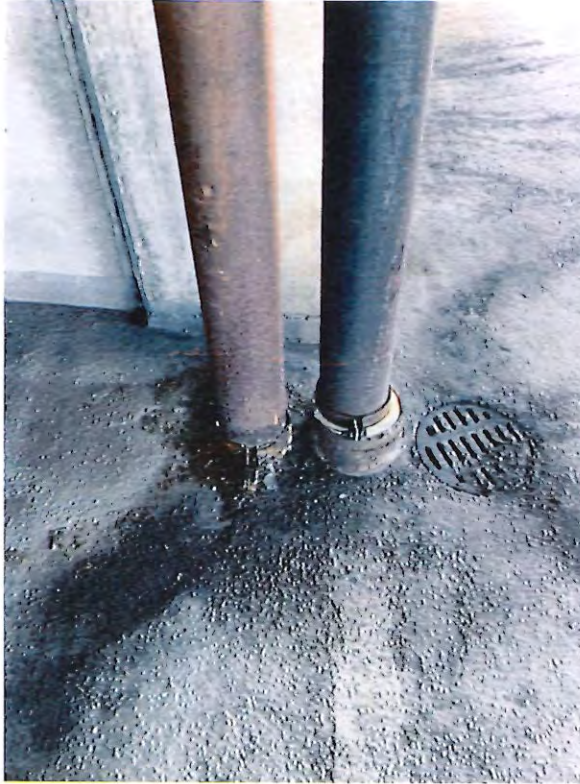
29 - corroded drain pipe and sleeves.JPG
