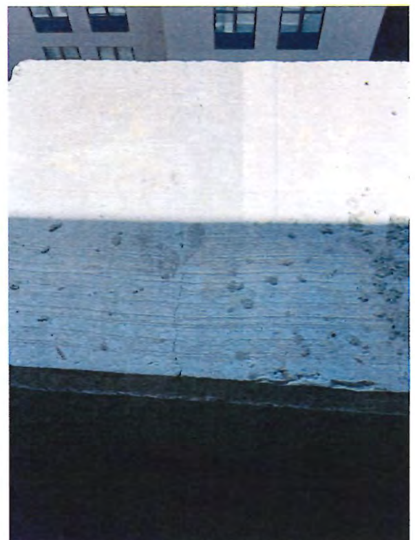
8 - exterior wall cracks.JPG
