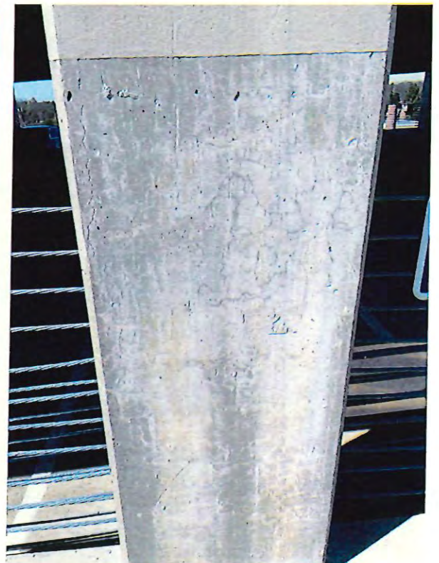
4 - column cracks with delamination.JPG
