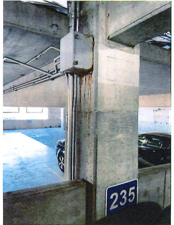
30 - corroded electrical box.JPG
