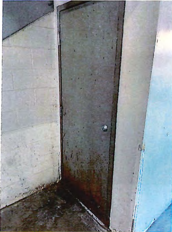
33 - door and frame corrosion.JPG
