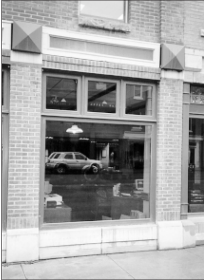
Include traditional elements such as display windows, kickplates and transoms on commercial storefronts. (Canton, OH)
