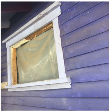
Incorrect trim profile and missing window.jpeg
