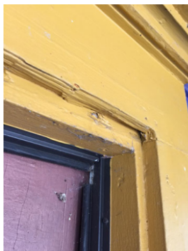
damaged trim .jpeg
