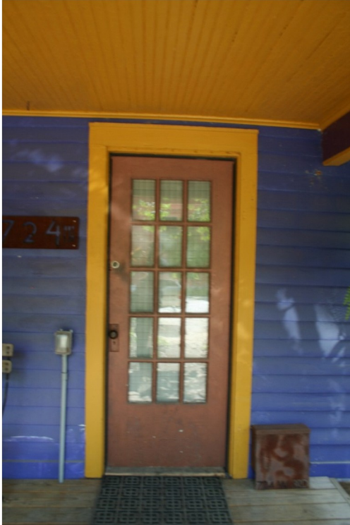
Non-original front door, to be replaced
