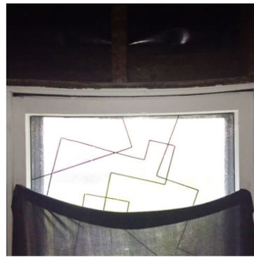
missing headers warped and broken windows and...
