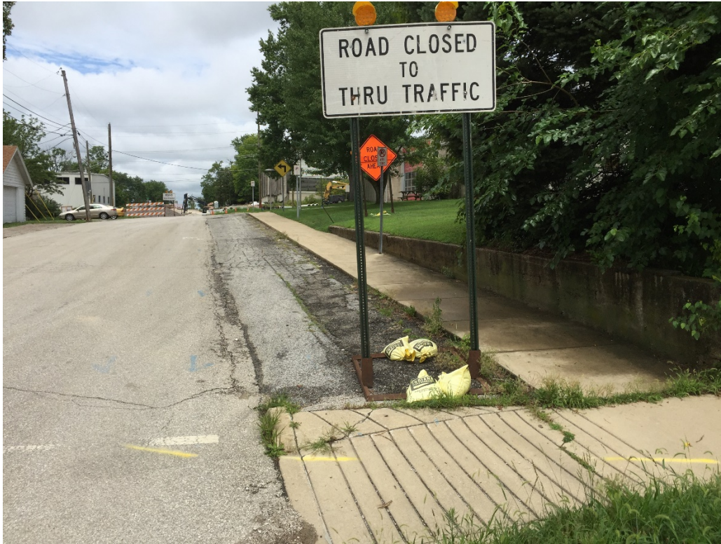
Woodlawn Avenue, north of 11 th . Wall to be removed, broken pavement to be replaced.
