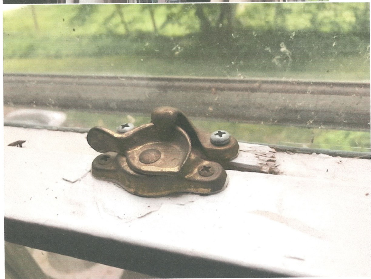
The top picture shows the outside of the window and the incorrectly installed storm window. The middle two pictures show the sash ropes cut and the bottom picture shows the modifications to the window lock.
