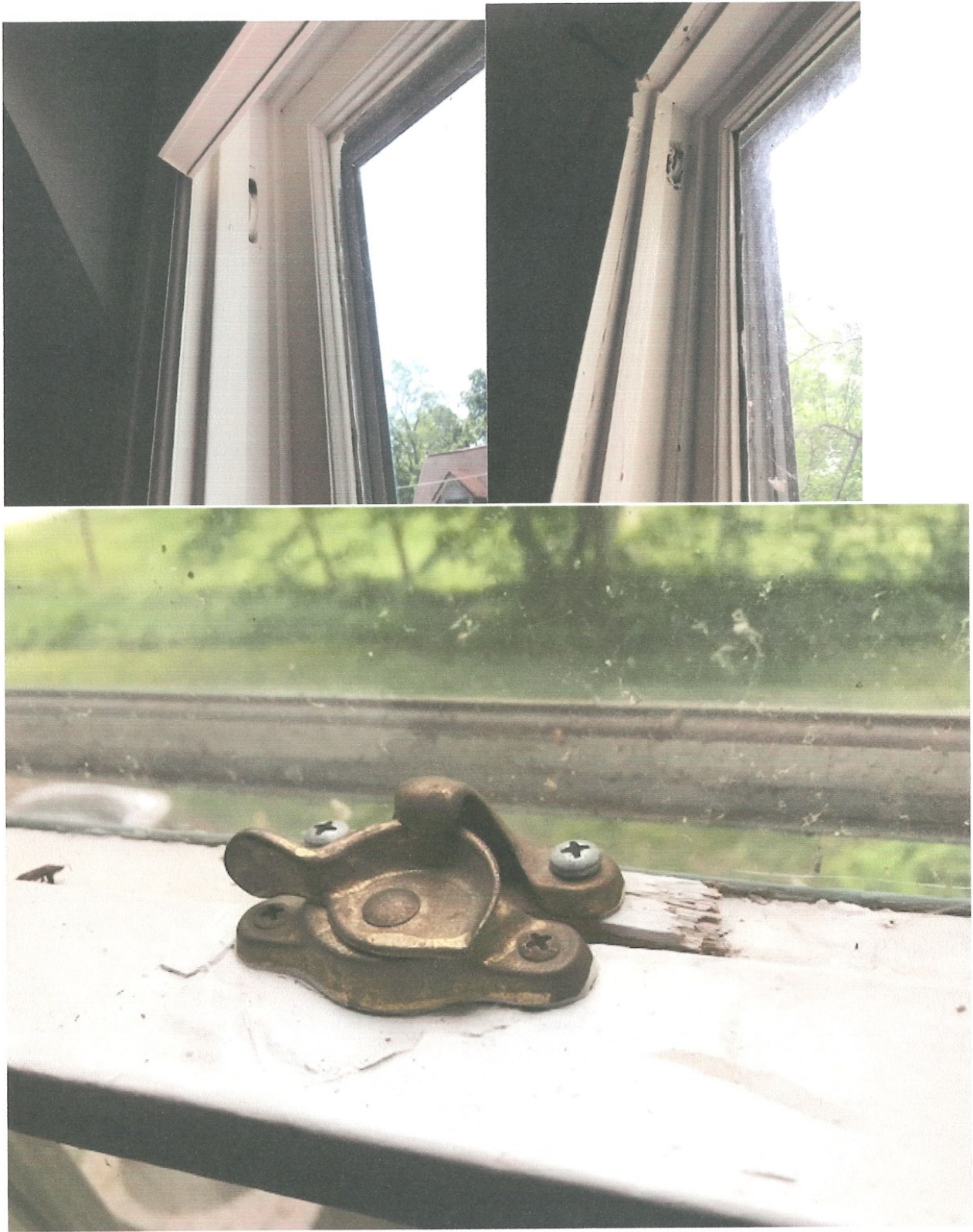
The top picture shows the outside of the window and the incorrectly installed storm window. The middle two pictures show the sash ropes cut and the bottom picture shows the modifications to the window lock.
