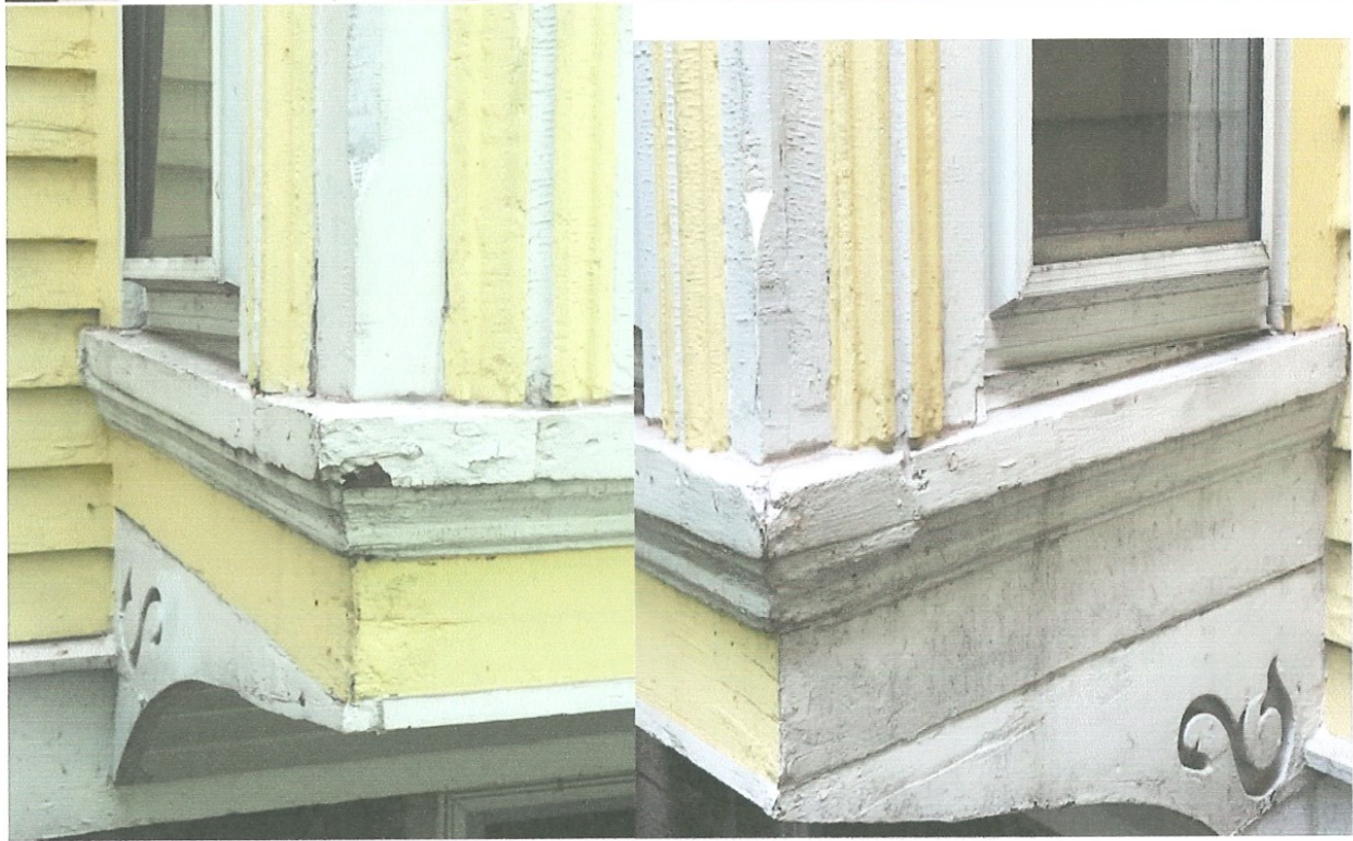
These pictures show a wide range of issues with these windows and supporting structure.
