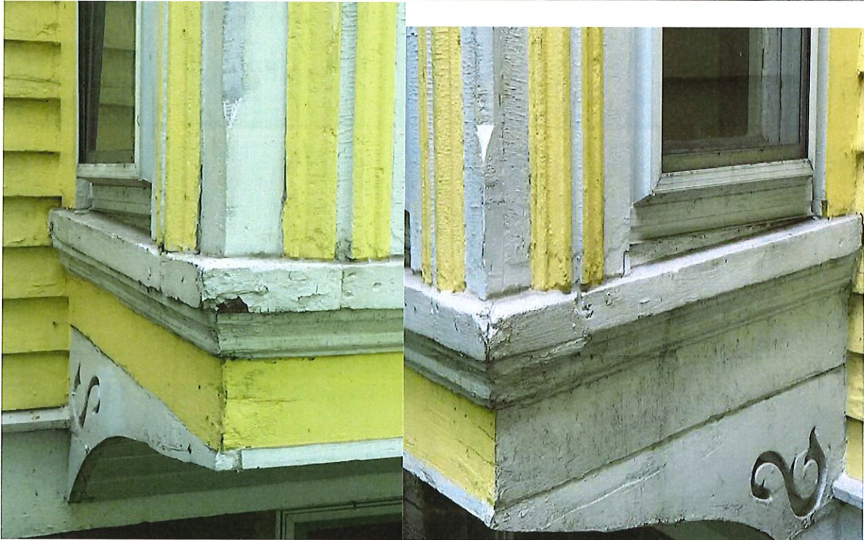
These pictures show a wide range of issues with these windows and supporting structure.
