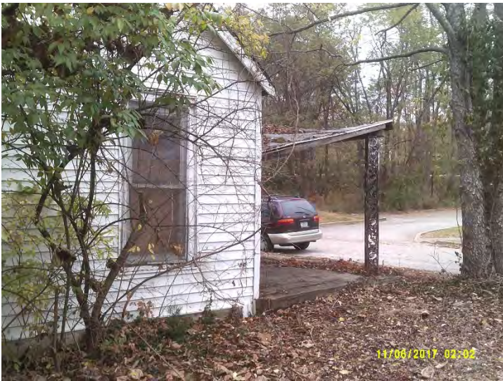
East wall and collapsed porch roof No. 10
