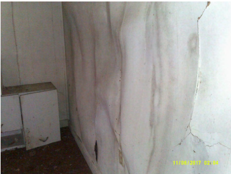
Interior wall damage- No. 15
