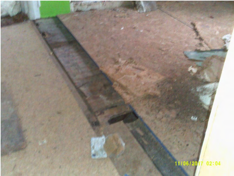
Interior floor damage – No. 13
