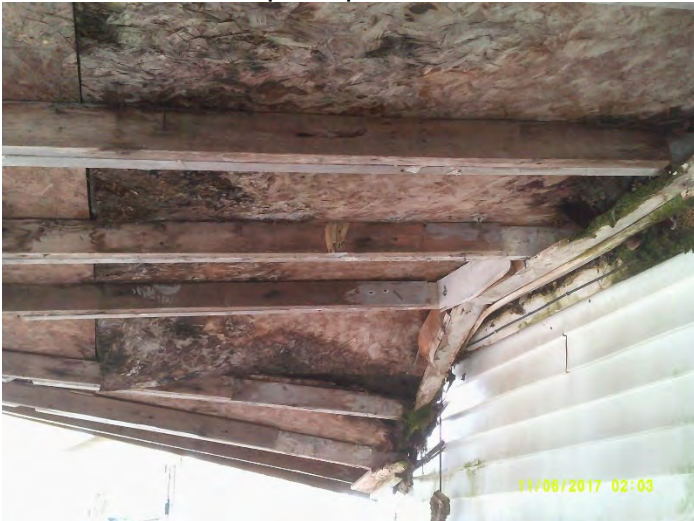
Porch roof failure – No 11
