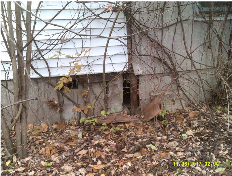
Foundation gap on west side- Rear addition built on posts – No 5
