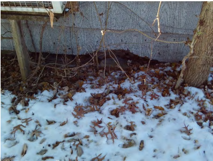
Hole in foundation on east wall – No. 10
