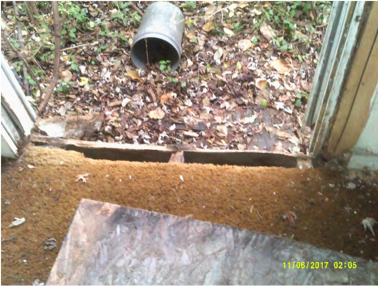
Damage at rear entrance – No. 16
