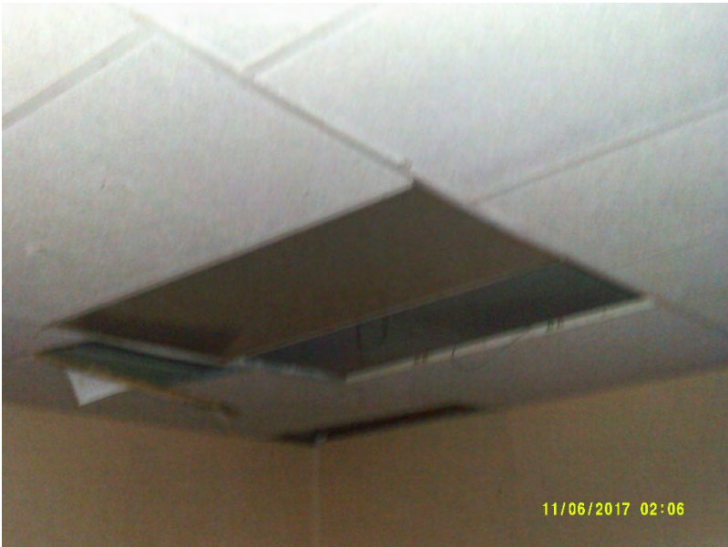
Ceiling damage – No. 18
