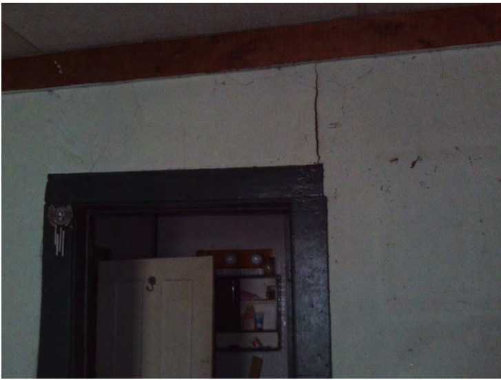
Movement at interior door corner- No. 23
