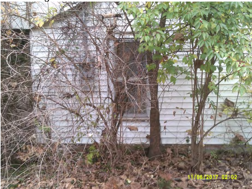
Trees along east wall – No. 9
