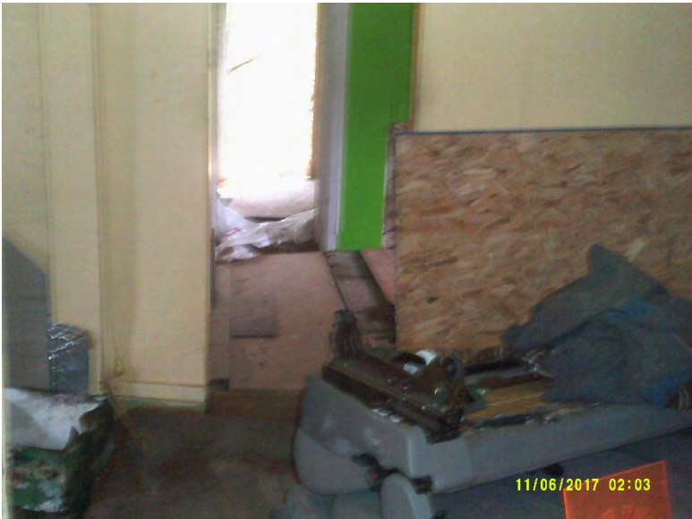
Floor damage at front door No. 12
