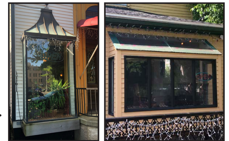
Examples of Incompatible Windows
